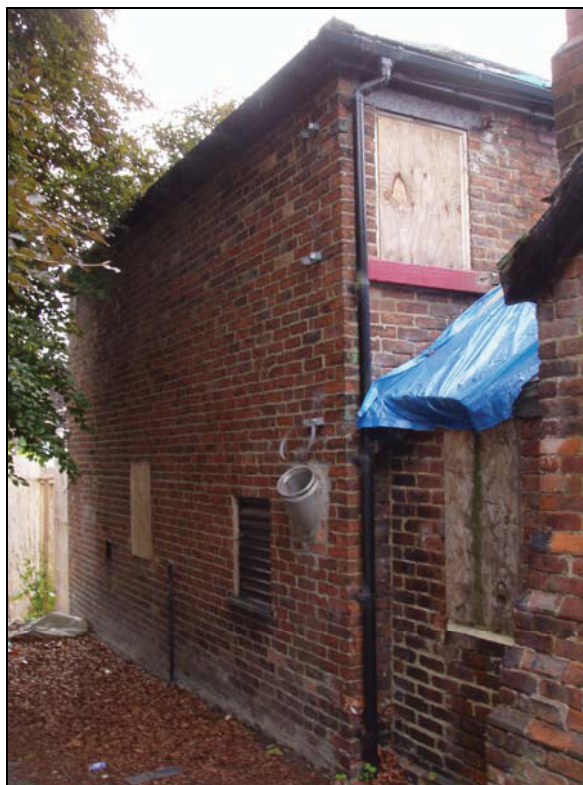
Plate 12: view of the gable wall (southeast elevation: Building A2), from the northwest
