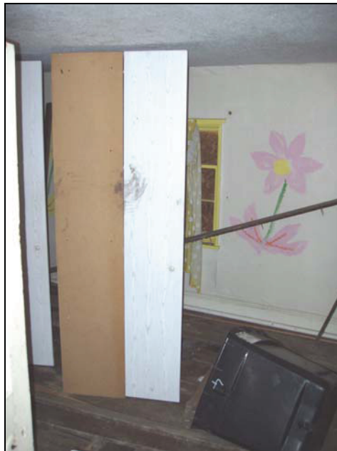
Plate 18: one of the bedrooms to the first floor (Building A2), from the west
