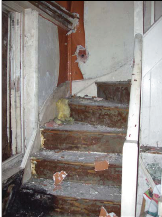
Plate 15: The remodeled early 20 th century quarter-turn principal staircase (Building A2), from the south
