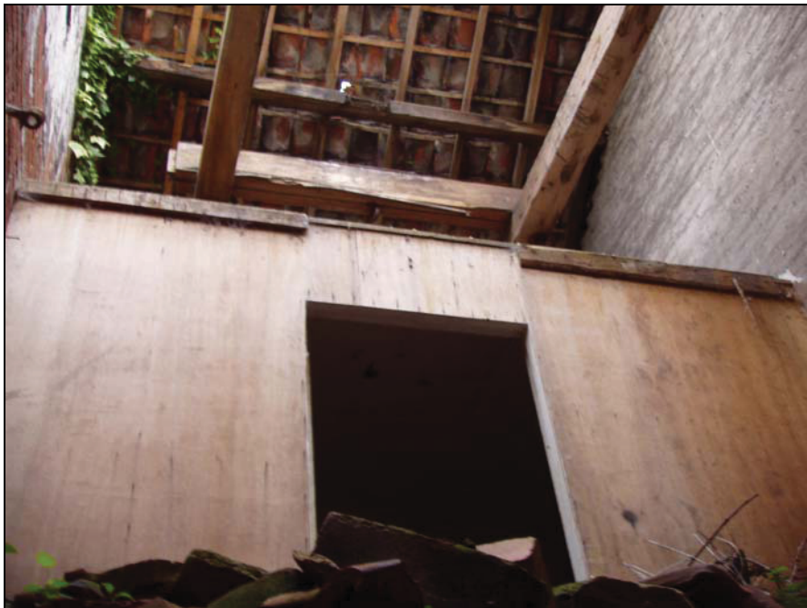
Plate 22: internal view of the probable stable with hayloft above, which forms the central 2-storey section (Building A3), taken from below the doorway, from the southwest
