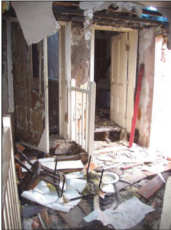
Plate 17: The first floor landing of the principal staircase (Building A2), from the northeast
