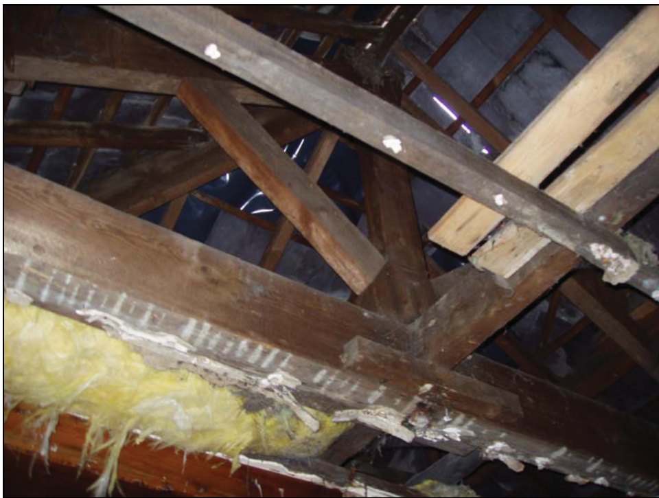
Plate 8: The original hipped roof with king-post truss (Building A1), from the north
