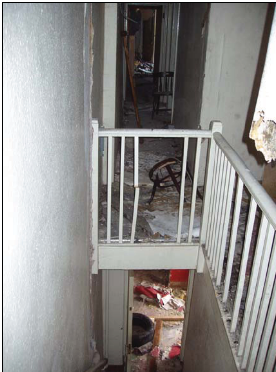
Plate 16: view of the plain balustrade of the straight flight northern staircase (Building A2), from the northeast
