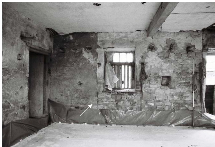
Plate 28, 71: view of the east wall with vertical building line [1], from the west
