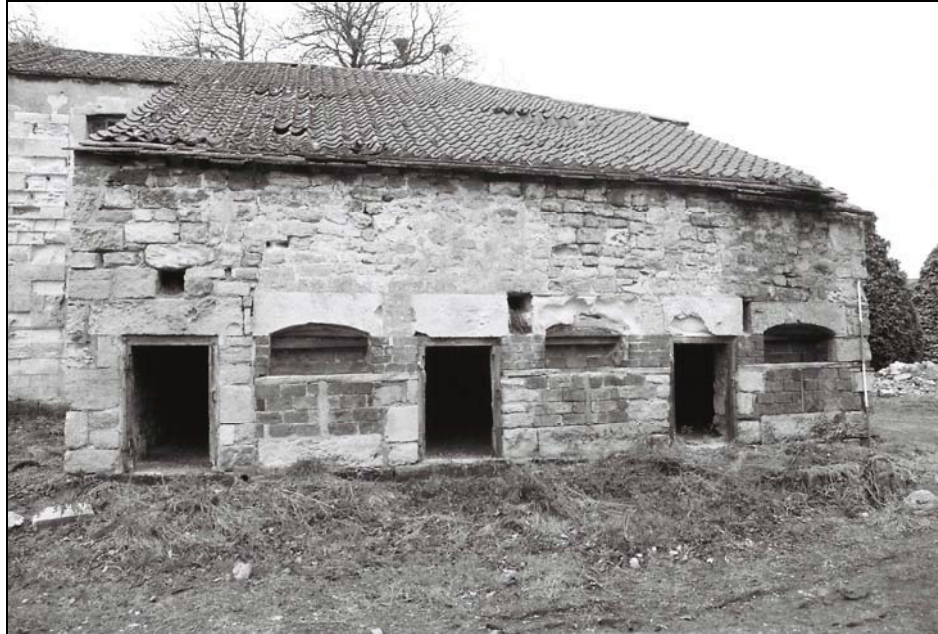
Plate 21, 44: view of the front, east elevation of the eastern extension, from the east
