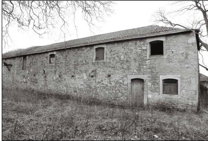
Plate 25, 53: view of the southern end of the west elevation, from the south southwest
