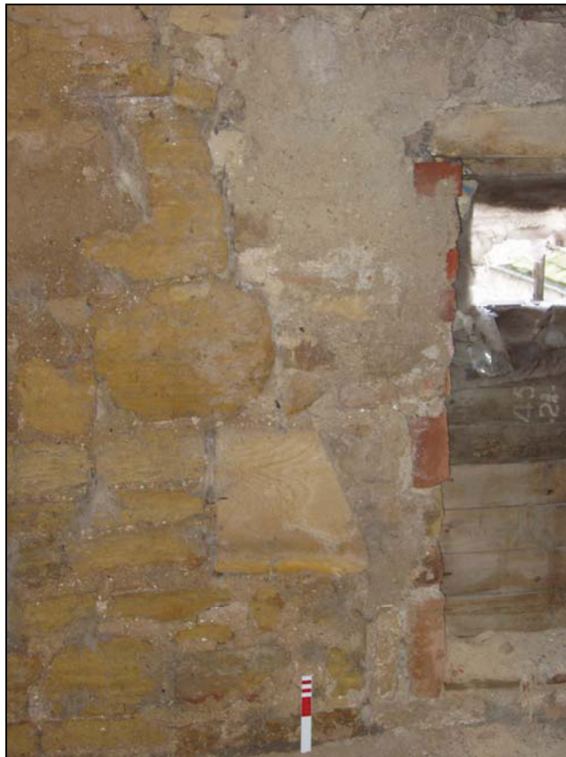
Plate 34, 230: detail of the in situ voussoir to the east wall, from the west
