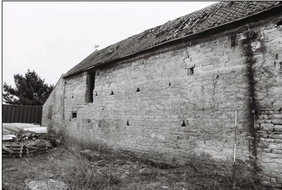
Plate 3, 5: oblique view of the eastern end of the north elevation, from the northwest
