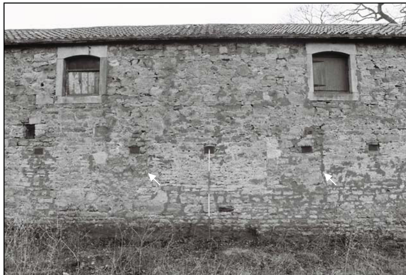
Plate 26, 59: view of the west elevation with original arched windows, inserted modern ventilators and two blocked windows, from the west
