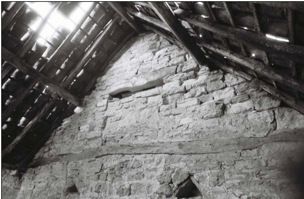
Plate 18, 173: oblique view of the blocked pitching hole [2] and ventilators to the east wall
