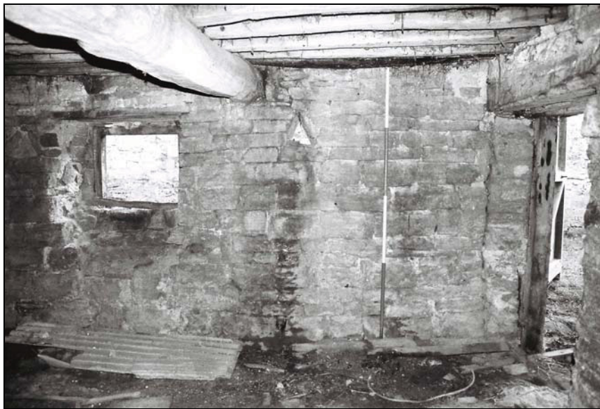
Plate 10, 143: view of the south wall with original triangular ventilator, from the north
