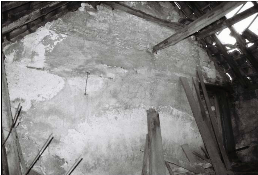
Plate 16, 156: General view with the inserted ceiling beam with mortice holes, from the southeast
