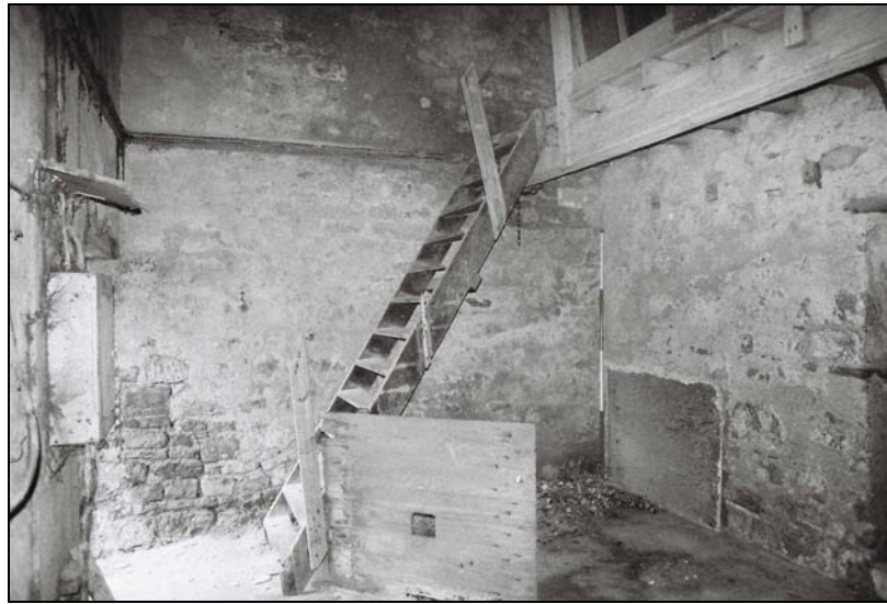
Plate 29, 79: general view with the probably original oak beam (ladder abutting) that would have supported the original hayloft
