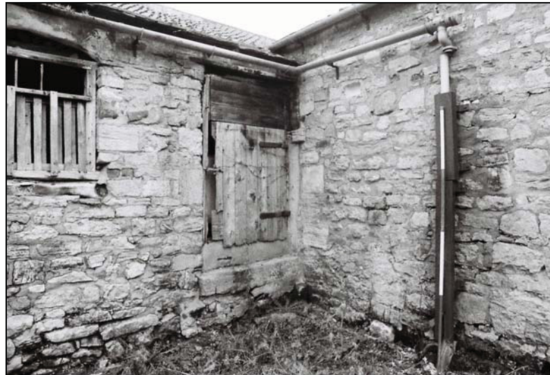
Plate 42, 27: detail of the corner with the built in pier, from the northwest
