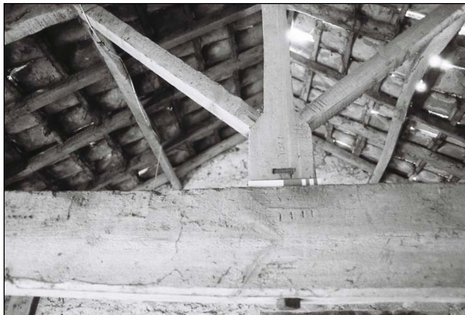
Plate 32, 100: detail of the carpenters marks (truss '1111') in ascending order S-N, from the south
