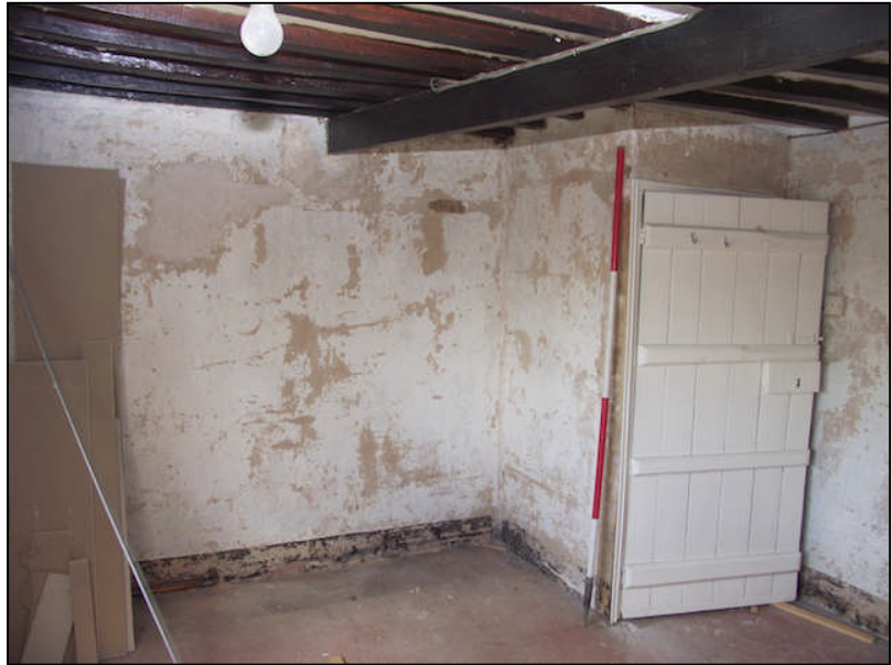
Plate 4: Exposed gypsum plaster floors in the rear bedroom and faint outline of a timber frame within the rear wall
