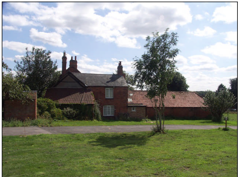
Plate 2: North facing elevation of farmhouse, showing two storey extension at right angles to timber frame cell and pantile roofed lean-to extension
