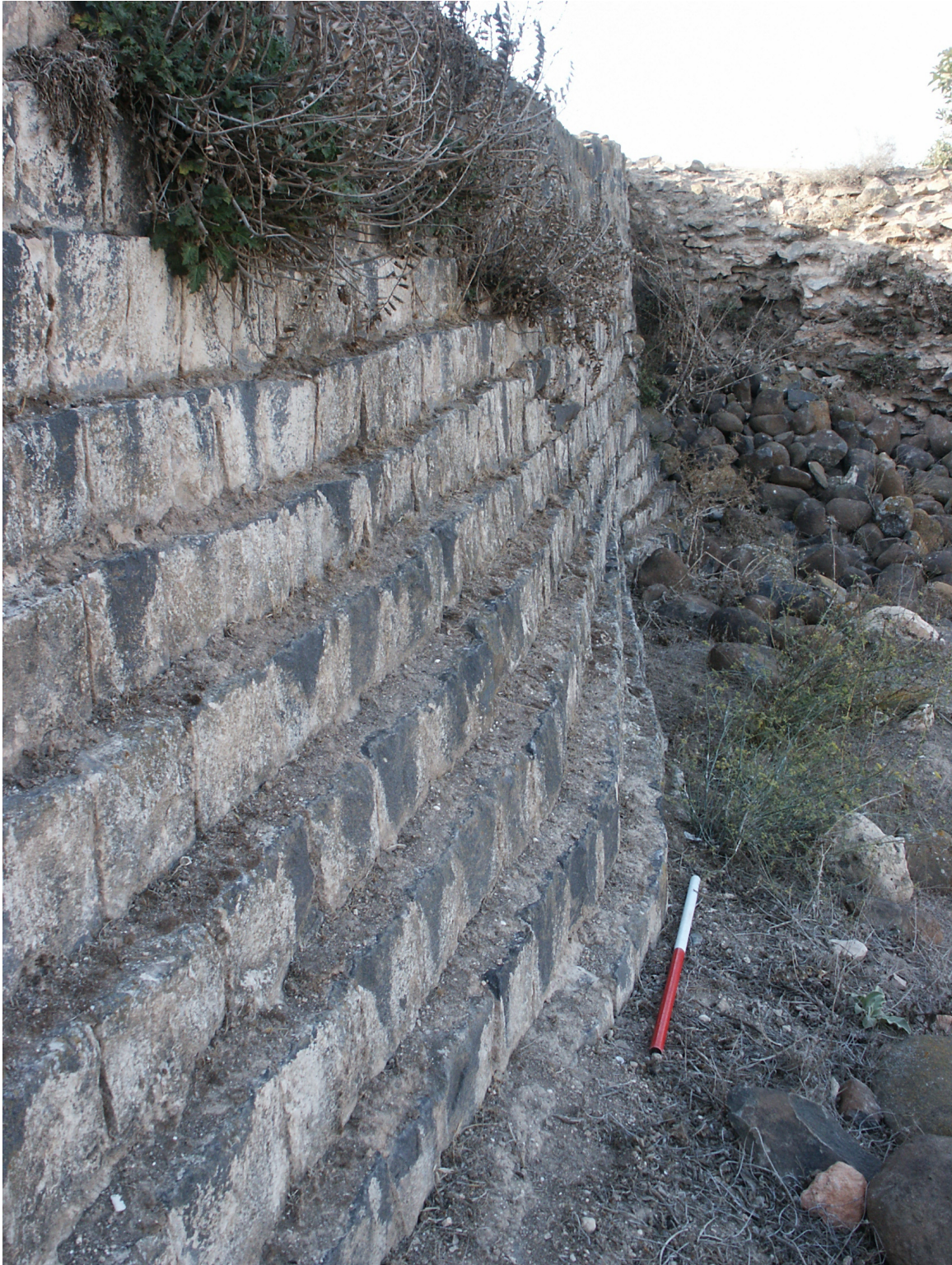
Fig. 4.11: Detail of the Homs dam, Syria showing the waving stepped courses [photo: author].
