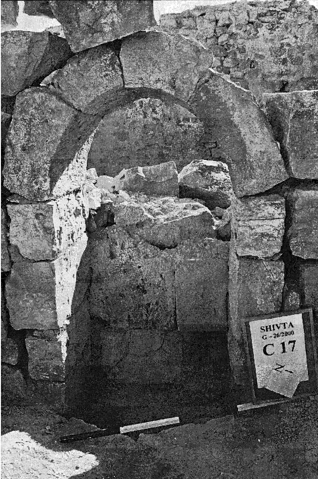
Fig. 9.12: Cistern no.17, Sbeitih/Shivta. A hole, 15 mm large, was found in the arch structure that may have been used for a pulley system over the recessed draw-shaft [Tsuk 2002c, fig. 3].
