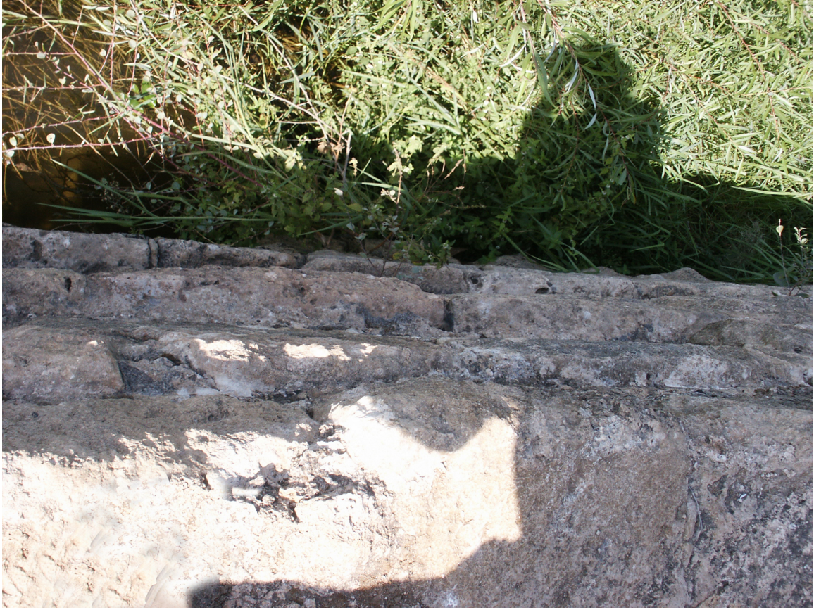
Fig. 4.17: Detail of the Tell Kazel dam, Syria, showing the stepped courses [photo: author].
