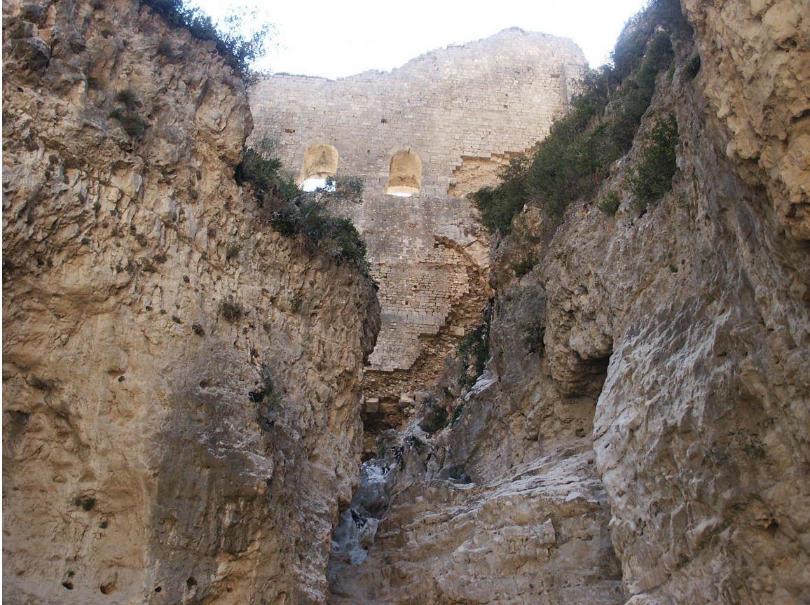
Fig. 4.5: 'Iron Gates' dam at Antioch, south-east Turkey, in a narrow valley [photo: author].
