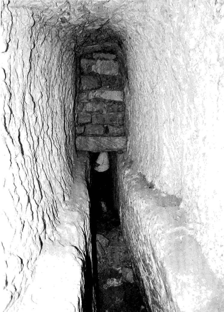
Fig. 6.9: Tunnel section of the Eleutheropolis aqueduct, Israel, showing a built-up section to support the tunnel roof [Sagiv et al. 2002, fig. 8].
