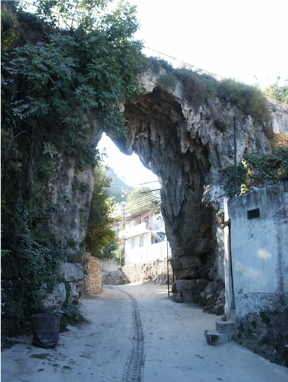
Fig. 6.30: Limescale incrustation on an aqueduct bridge in Antioch, south-eastern Turkey [photo: author].
