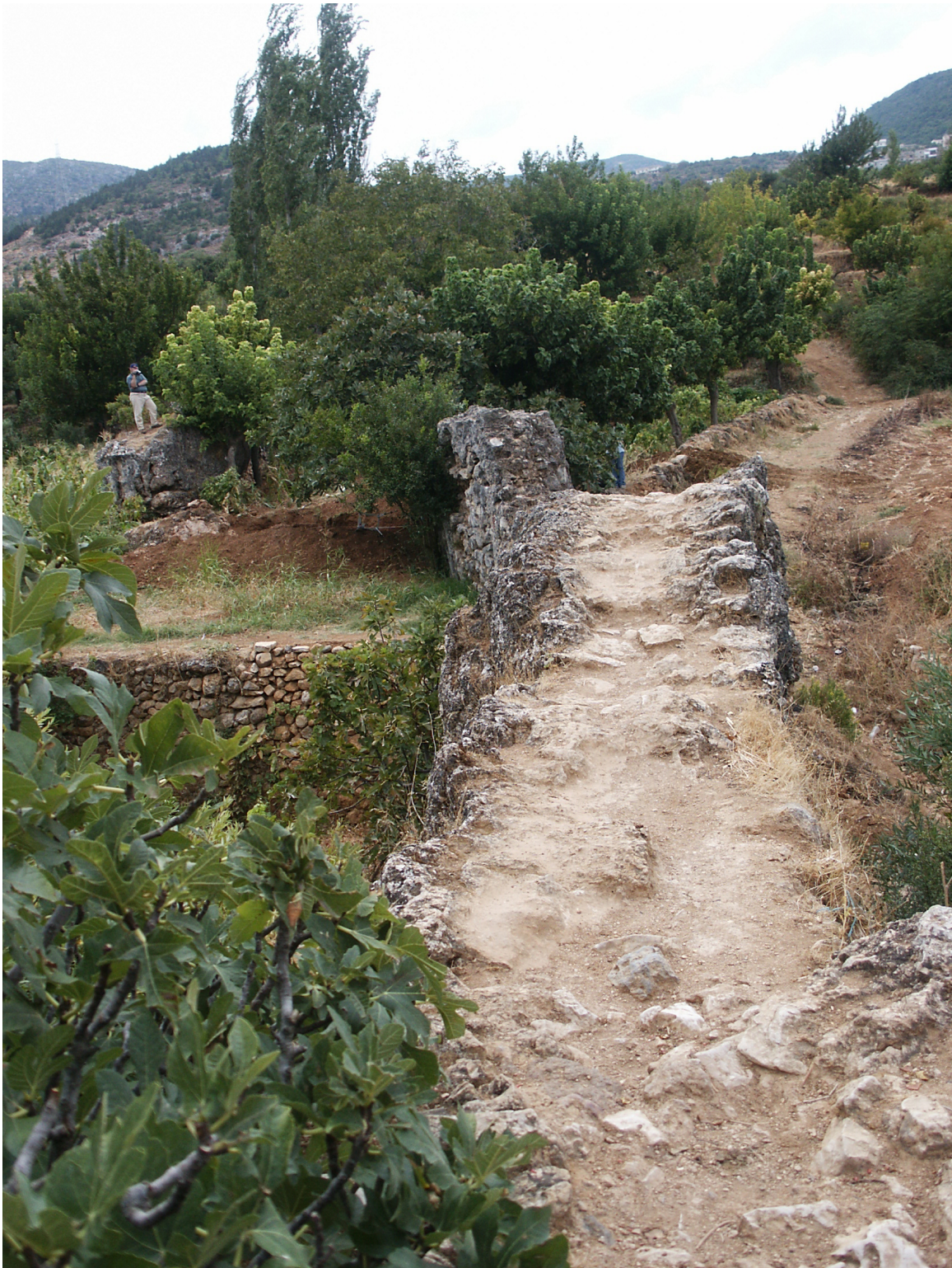
Fig. 6.29: Earthquake damage at the Misyaf aqueduct, Syria; the figure in the background is standing on the section of the aqueduct that has shifted [photo: author].
