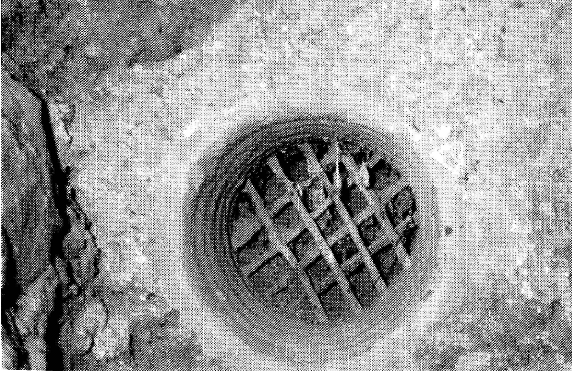
Fig. 7.11: Iron grille set into opening of a terracotta pipe, Baniyas [Hartal 2002, fig. 19].
