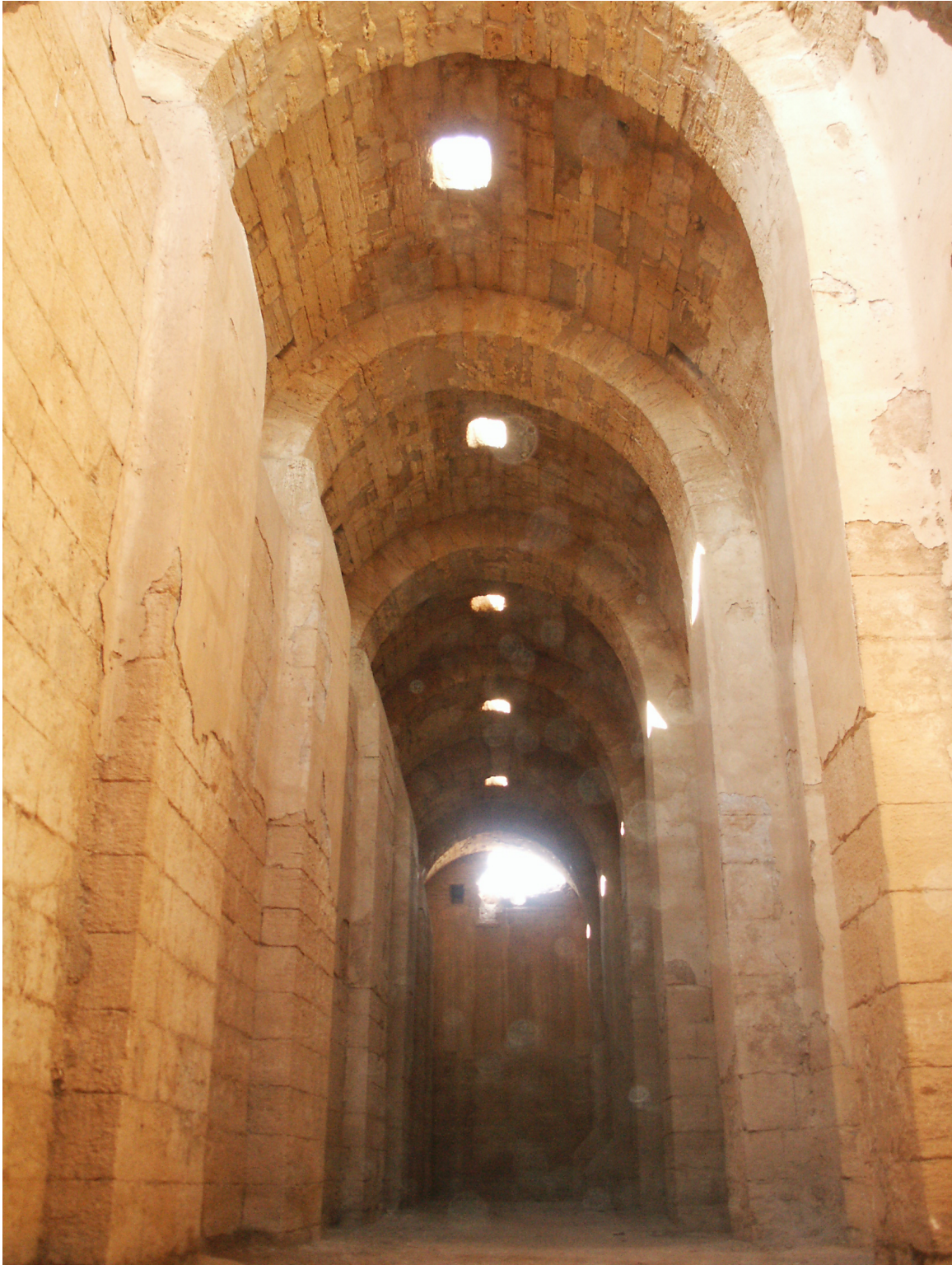
Fig. 7.23: Holes in the ceiling of the 'Big Reservoir-Cistern', Resafe [photo: author].
