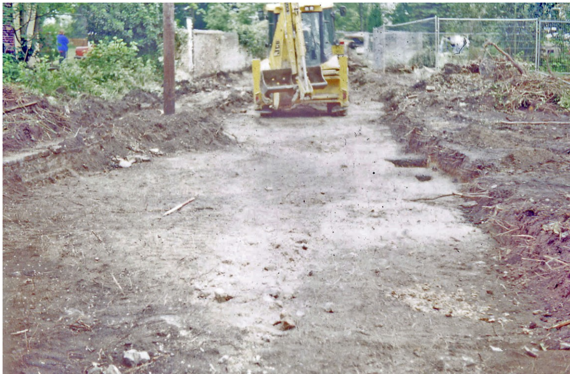
Plate 2. General view, looking north, of topsoil stripping at the south end of the access road with disturbance by tree root action in foreground.
