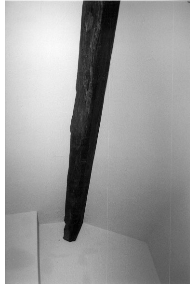
02/07 Cottages interior, west of centre, 2 nd floor detail of purlin facing W
