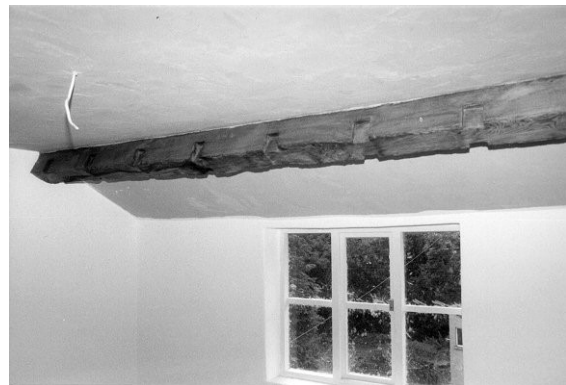
02/09 Cottages interior, east of centre, 2 nd floor detail of purlin facing SE
