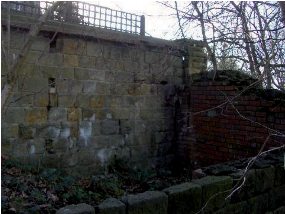
Plate 16 – S view of intersection of dilapidated outbuilding (probable former cold frame) and terrace wall
