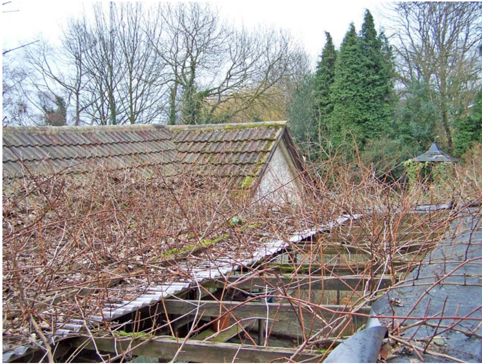
Plate 9: View of extension, looking east, showing missing sections of roof.
