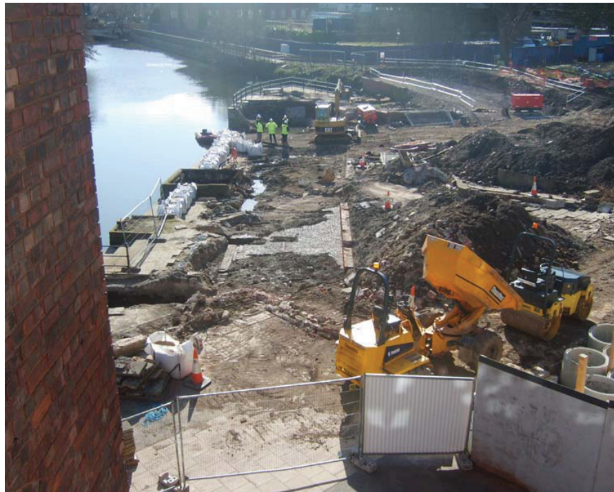
Plate 4: High level view of doubling shop site, showing the surviving footings and floor (centre). View south.
