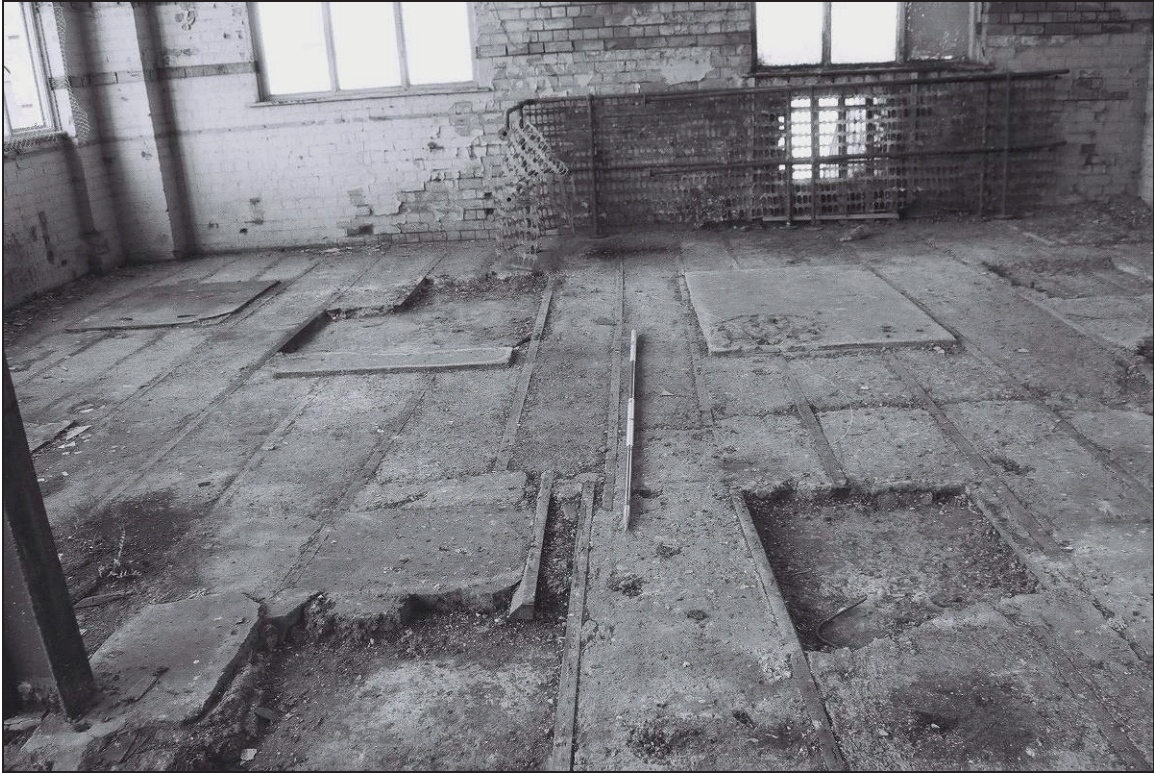
Plate 52: Detail of machine base scars in floor of F1 (film 14.31)
