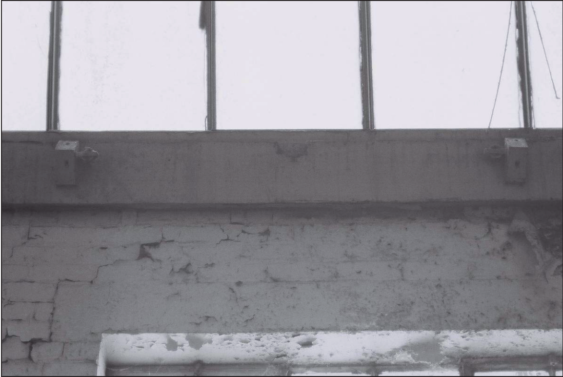
Plate 66: Detail of pulley wheels on truss of north light roof, F2 (film 14.10)
