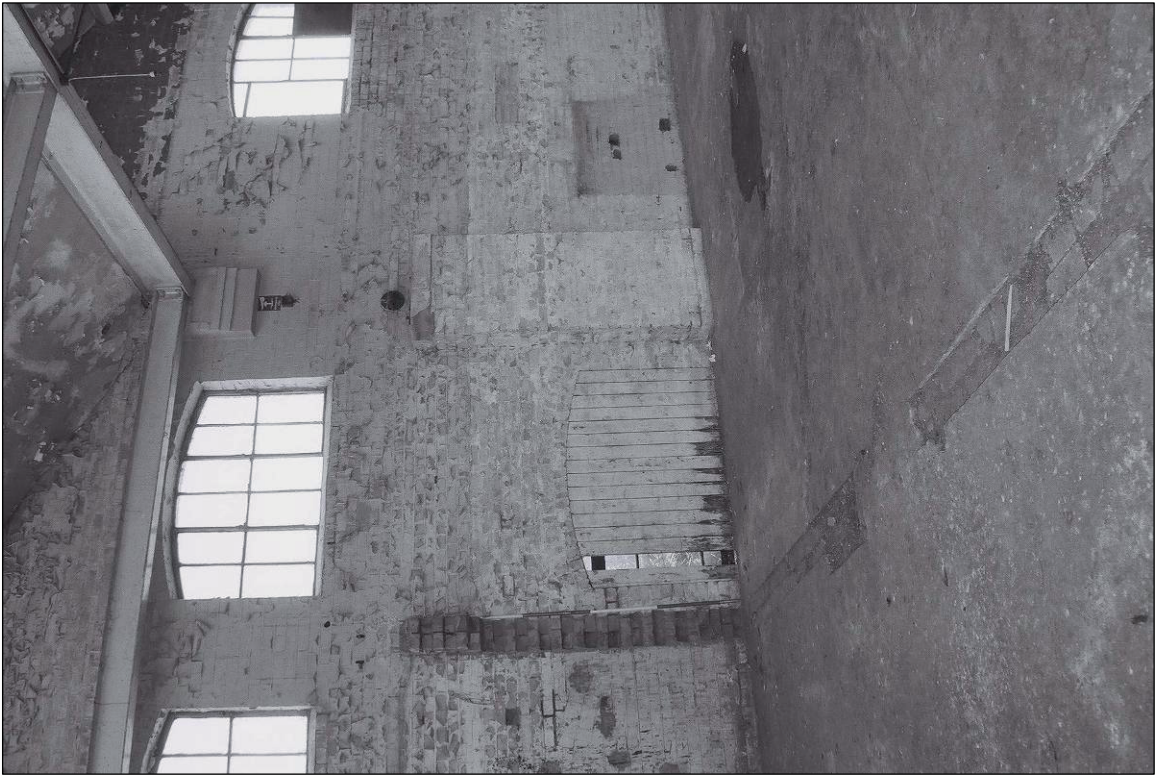
Plate 64: General view of southeast wall of F3 showing scar in wall, window and brick pier (film 14.15)
