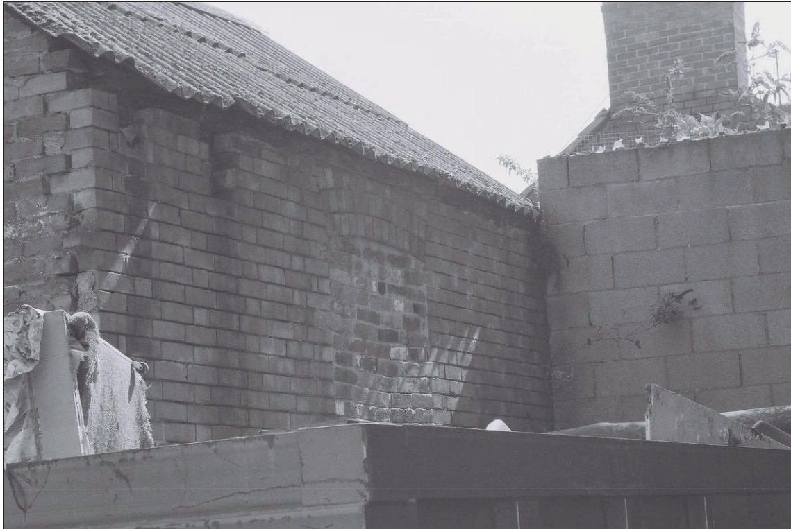
Plate 85: End gable wall of building 2 note blocked window/doorway (film 10.31)
