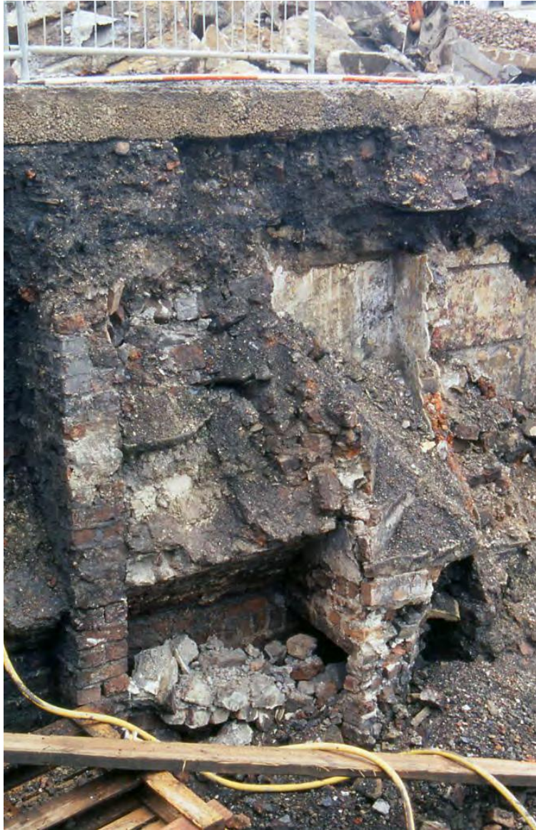
Plate 3: Section at western end of site before battering; vaulted cellars at the western edge of Court No.10 are visible
