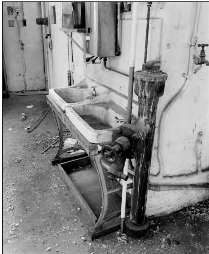
Plate 137: Building 4; detail of wash station and fire hydrant in A34 (Film 1.5)
