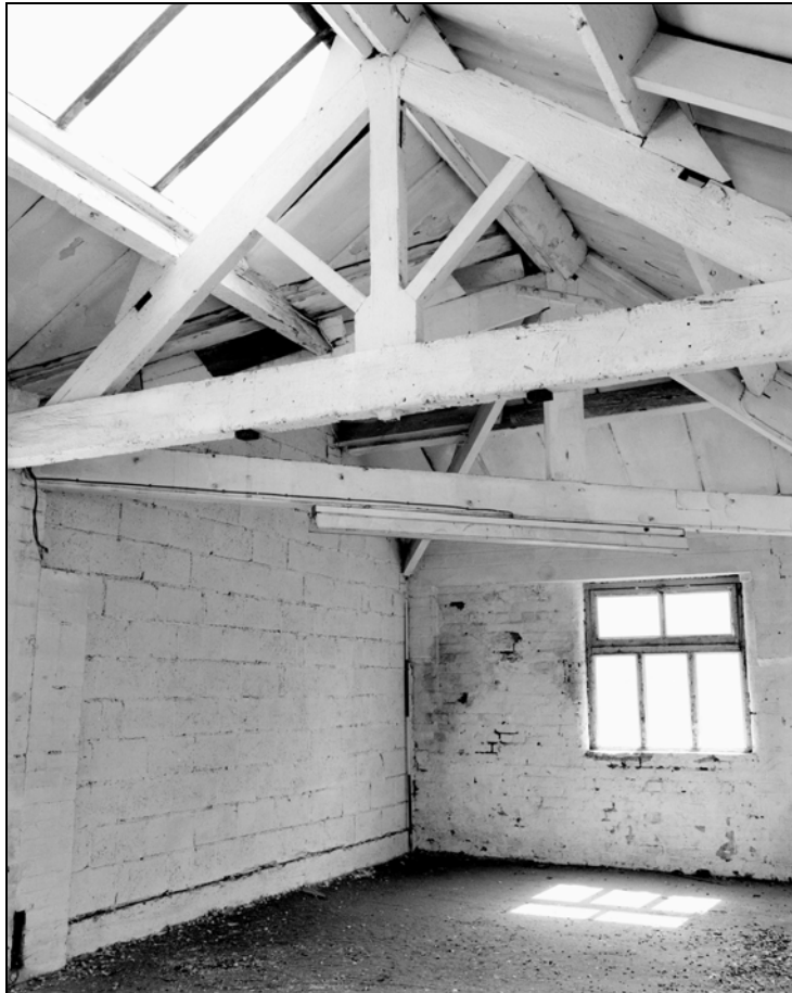
Plate 61: Building 2; hip trusses and inserted blanking wall at south-east end of A32b (Film 2.1)
