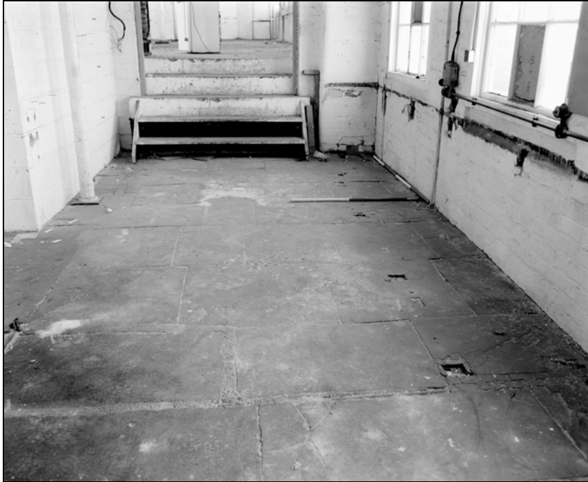
Plate 51: Building 2; first floor, detail of flag floor & removed benches in A20 (Film 4.6)
