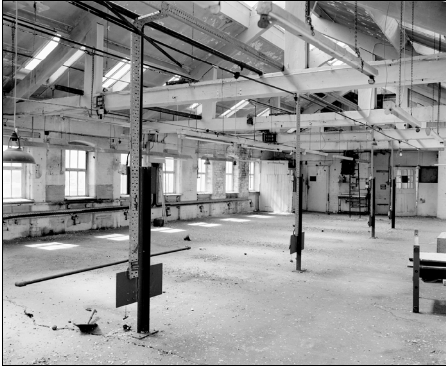
Plate 134: Building 4; second floor, general shot of A34 looking south to door partition (Film 1.2)
