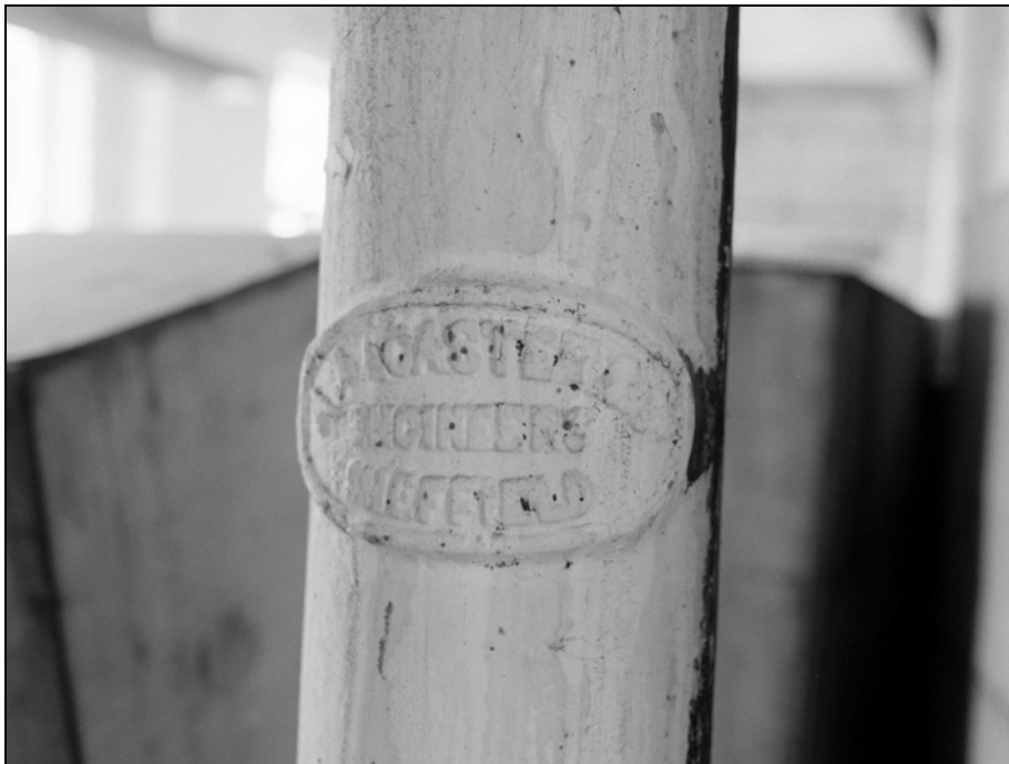
Plate 25: Building 1b, first floor; maker's name 'Lancaster & Co. Engineers Sheffield' on cast iron column, A15 (Film 3.5)
