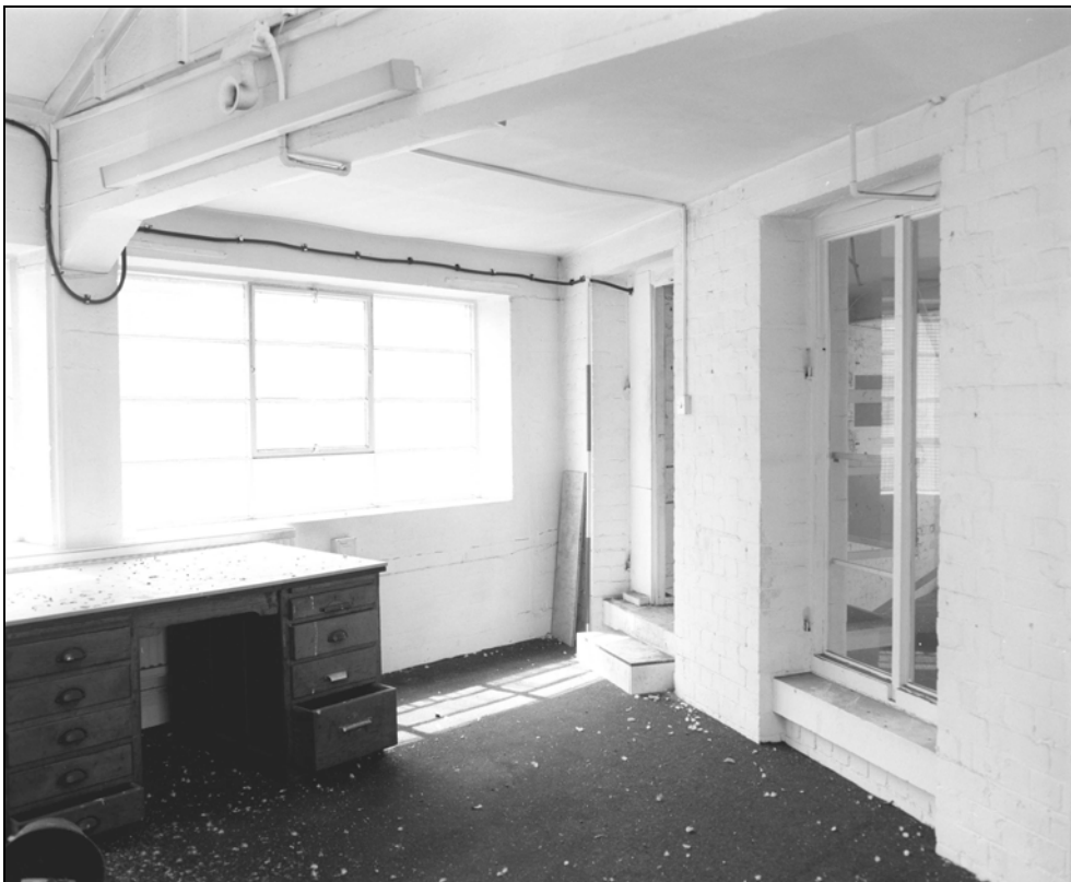
Plate 141: Building 5, first floor room A22a; door inserted in window bay of building 3 (Film 5.1)
