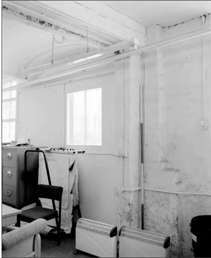
Plate 13: Building 1a, room A1; jack-arch ceiling and truncated wall return at east end (Film 7.10)
