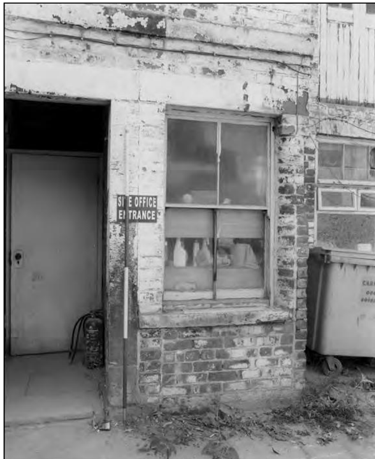
Plate 8: Building 1b rear elevation; door to stairwell A49, inserted window in blocked door (Film 10.8)
