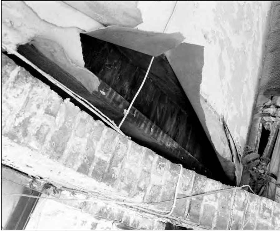
Plate 35: Building 2, east elevation, detail of beams over passage showing lath and plaster scars (Film 18.1)
