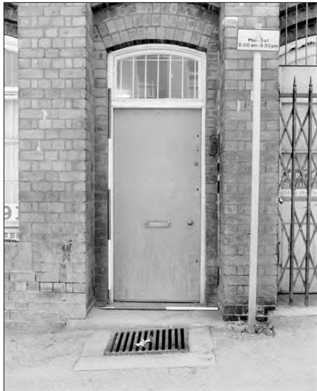
Plate 87: Building 4; east end of Upper Allen Street elevation, basement office door (Film 18.7)
