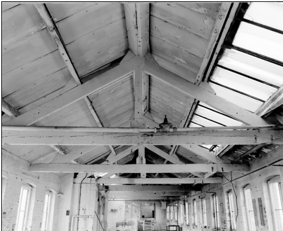
Plate 28: Building 1; second floor, detail of roof trusses, looking from A31b to A31a (Film 1.7)
