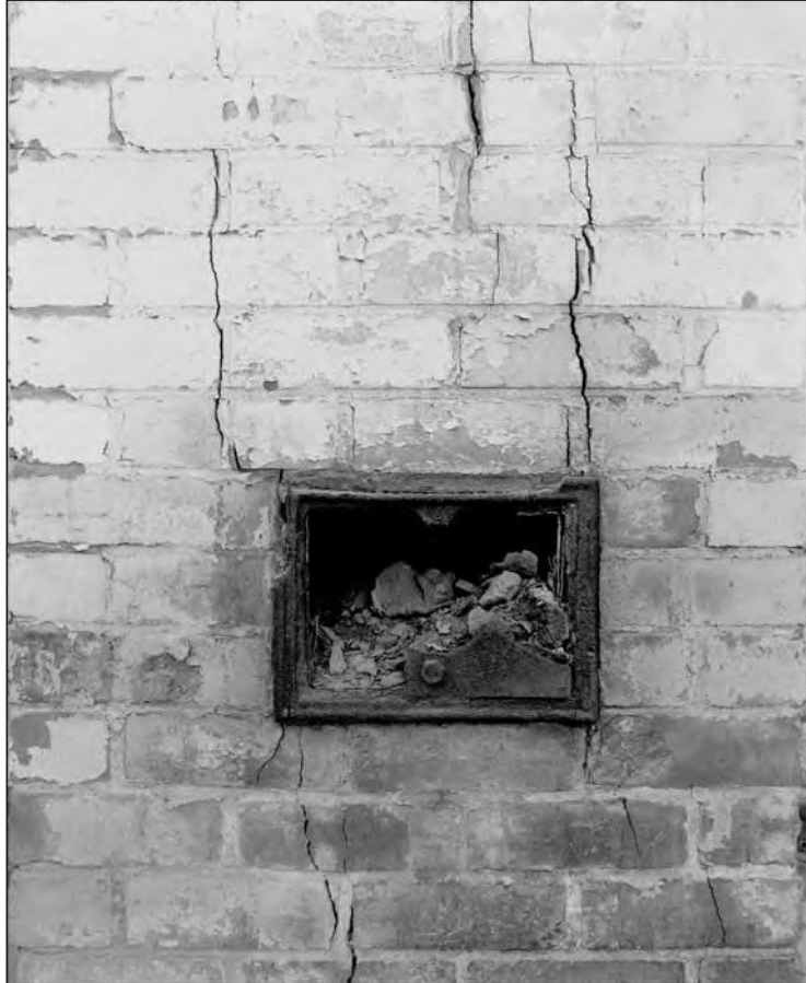
Plate 9: Building 1b rear elevation, rodding hole in flue at east end (Film 10.9)
