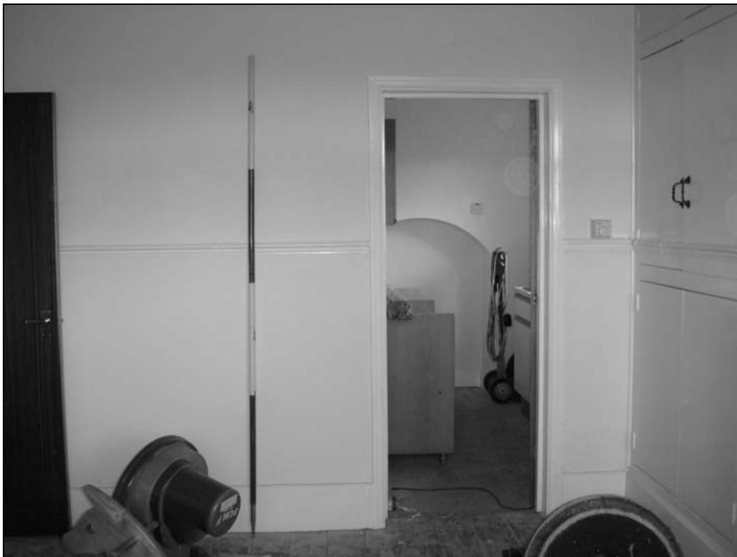
Plate 36 – General view of S2 & S3; note arch in south wall of S3 (film 2.03)
