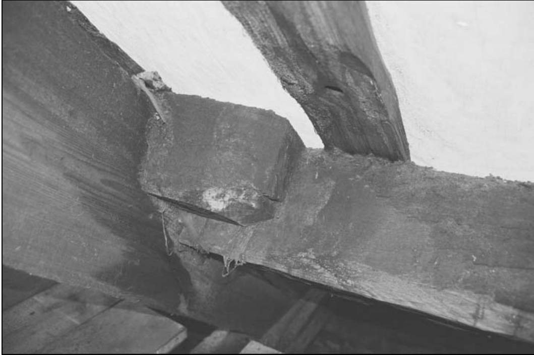
Plate 69 – Half lapped joint of purlin and principal in northern part of building (film 2.27)
