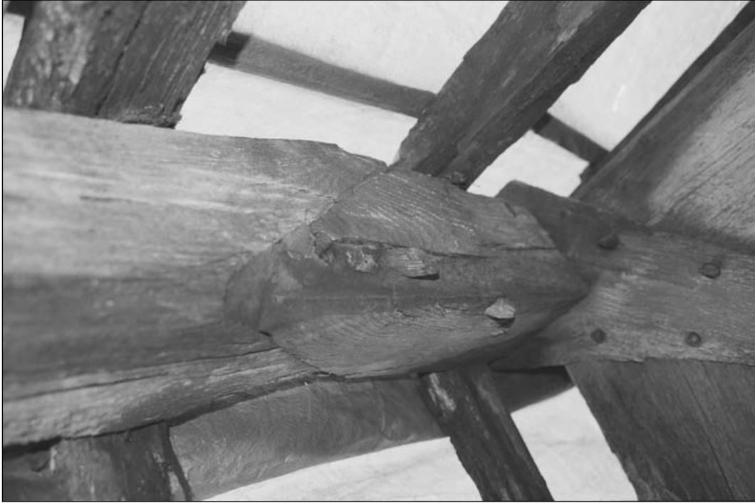
Plate 68 – Detail of lapped scarf joint in ridge piece of northern part of building (film 2.07)
