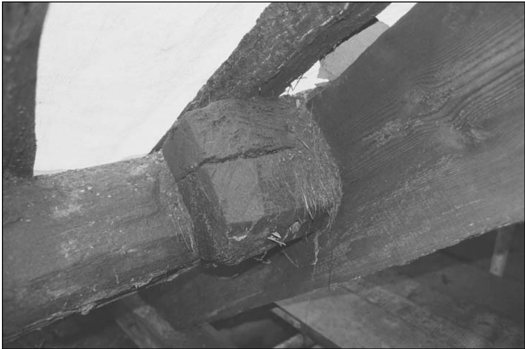
Plate 70 – Half lapped joint of purlin and principal in northern part of building (film 2.29)
