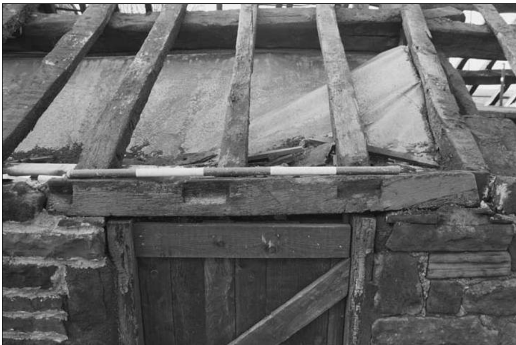
Plate 42 – Detail of notches in a lintel above an opening in the east wall (film 3.23) – 1m scale rod (in 20cm bands)
