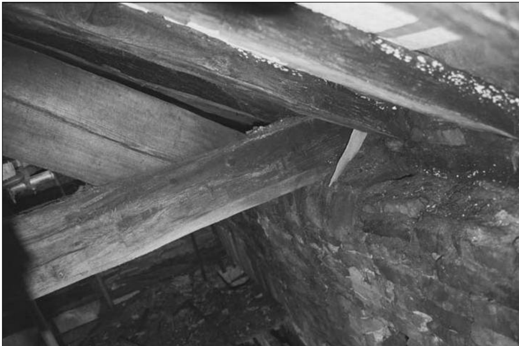
Plate 66 – Conjunction of tie beam and wall in northern part of building (film 2.03)
