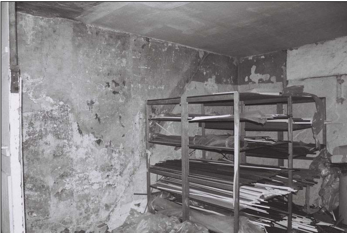
Plate 25: Room F9, detail of staircase scar on wall (film 1.11)
