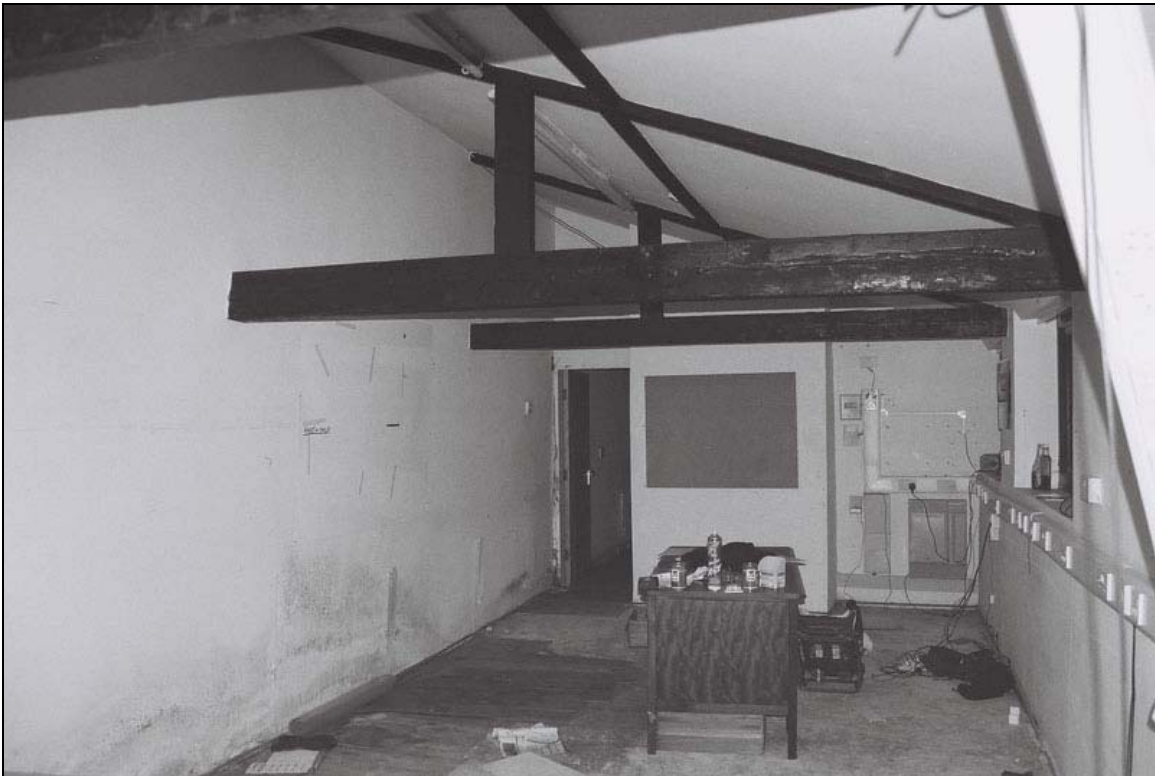
Plate 29: General view of room G10 looking north west, note timber trusses (film 1.2)
