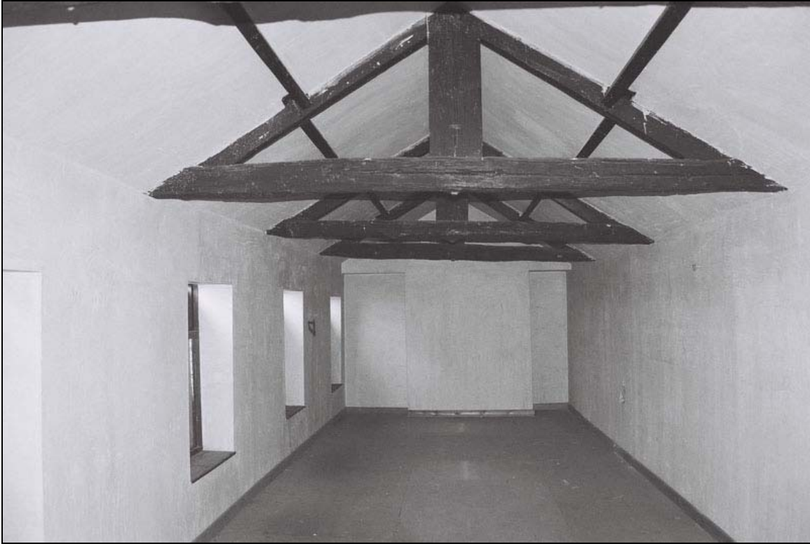
Plate 26: General view of room S6 looking south, note king post trusses (film 1.26)
