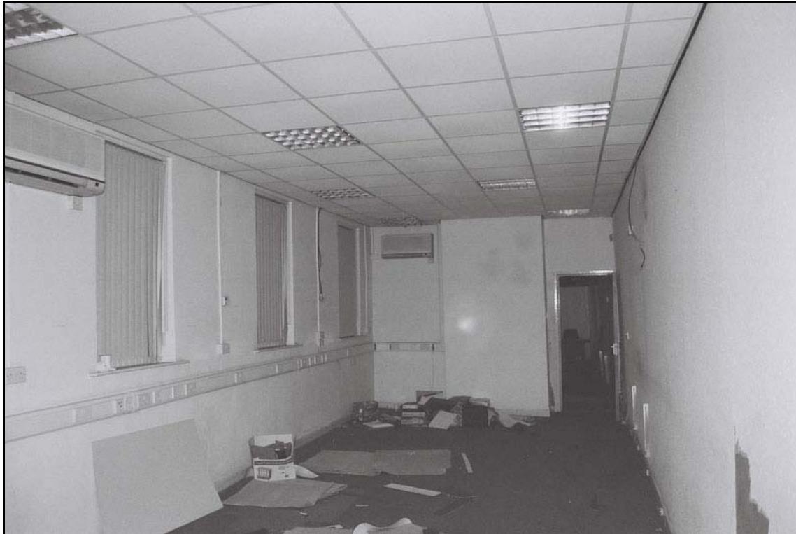
Plate 23: General view of room G9, note suspended ceiling and plaster boarding obscuring original features (film 1.3)
