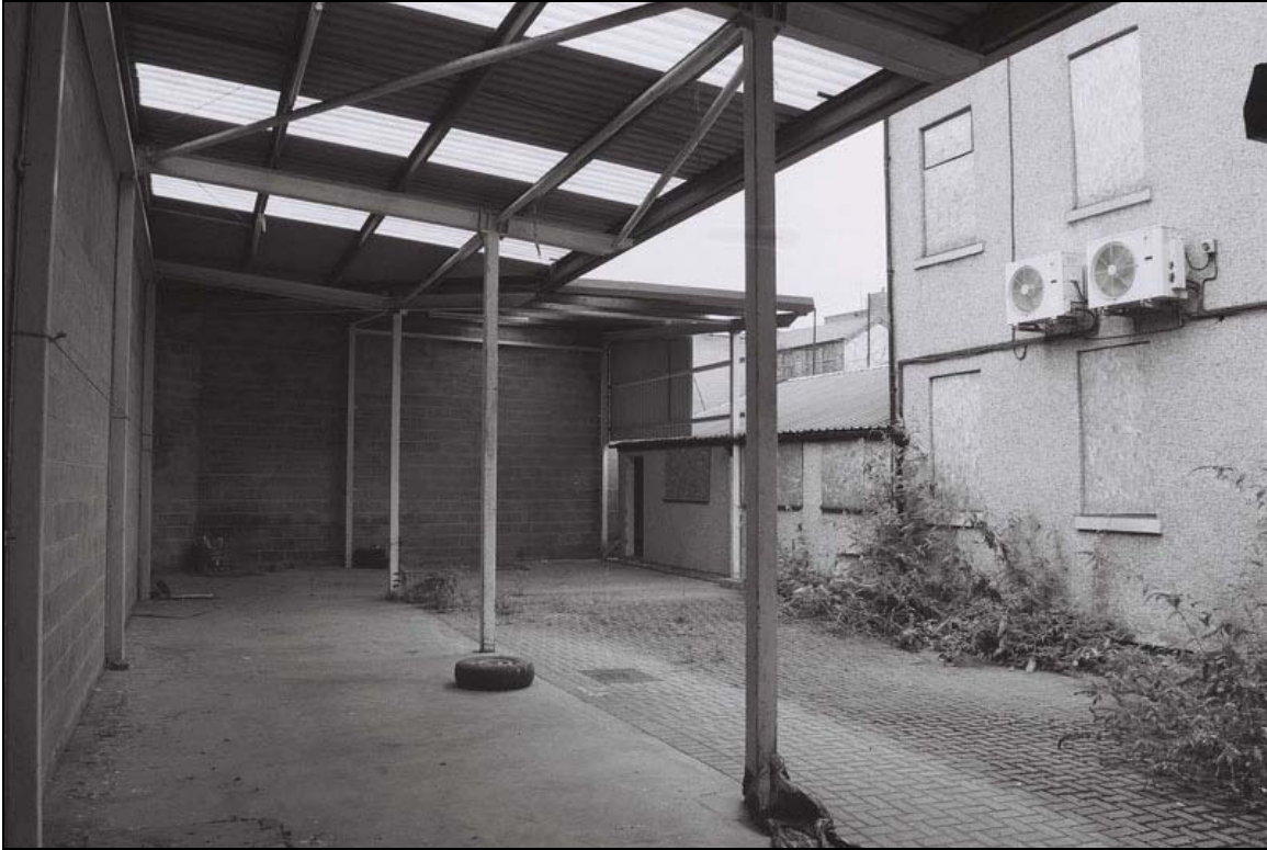
Plate 28: General view of central yard area and east elevation of building, note later single storey extension (film 1.35)
