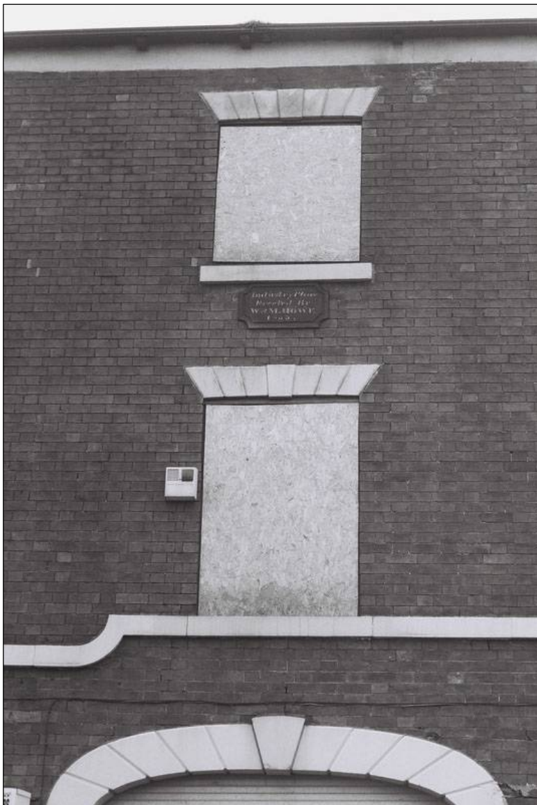
Plate 6: Detail of windows and date stone above cart passage in north elevation (film 1.31)
