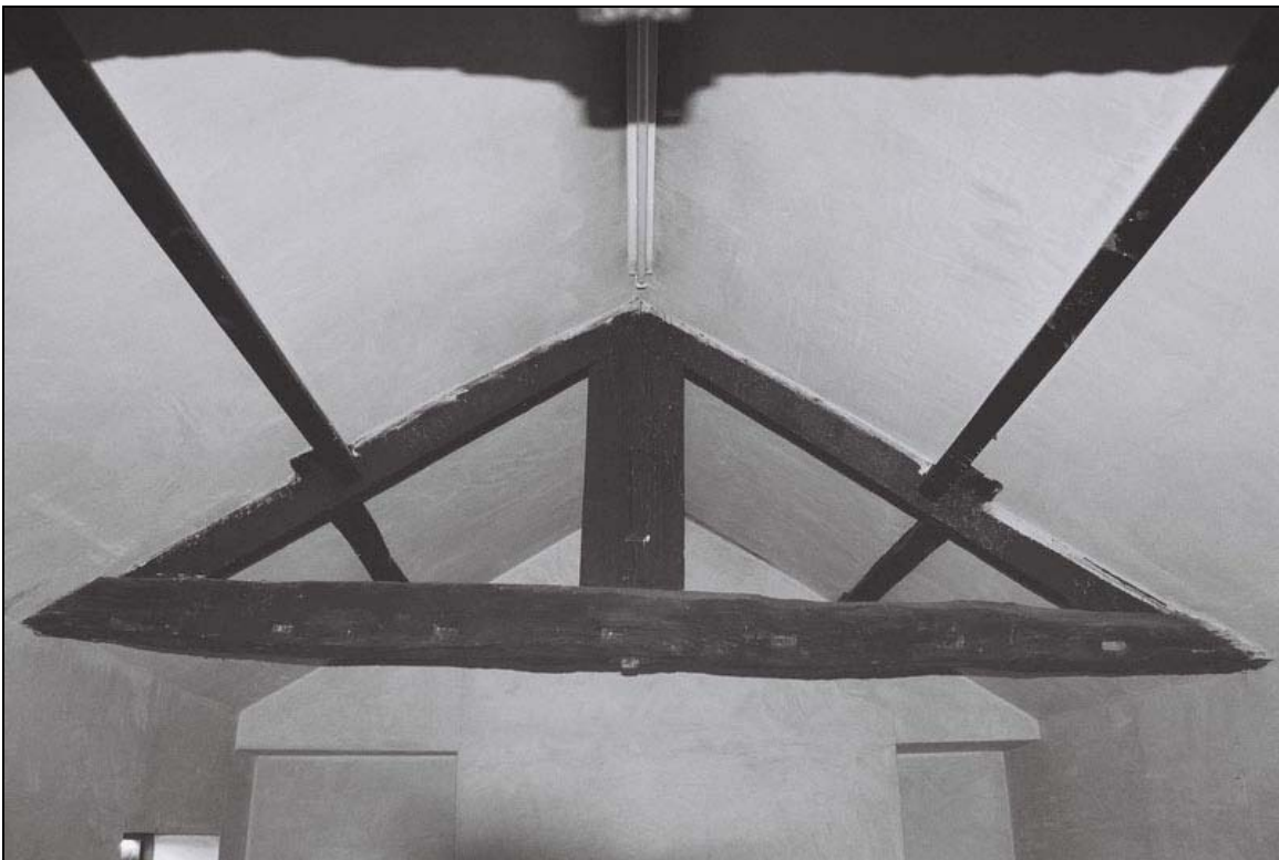
Plate 27: Room S6, detail of roof truss, note in filled slots suggesting a removed partition situated below (film 1.25)
