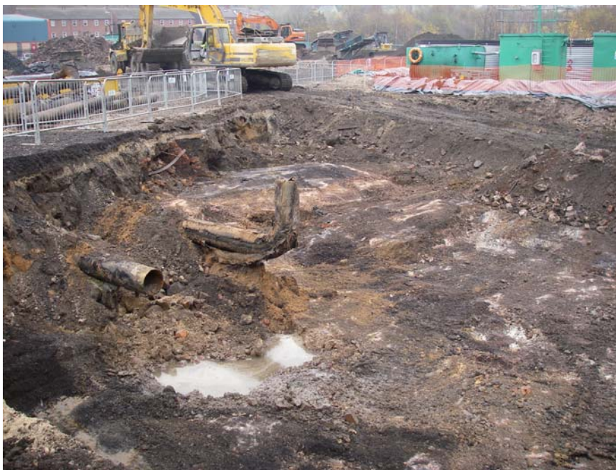
Plate 14: North-east view of the northern end of Area 6 showing the large pipes [028]
