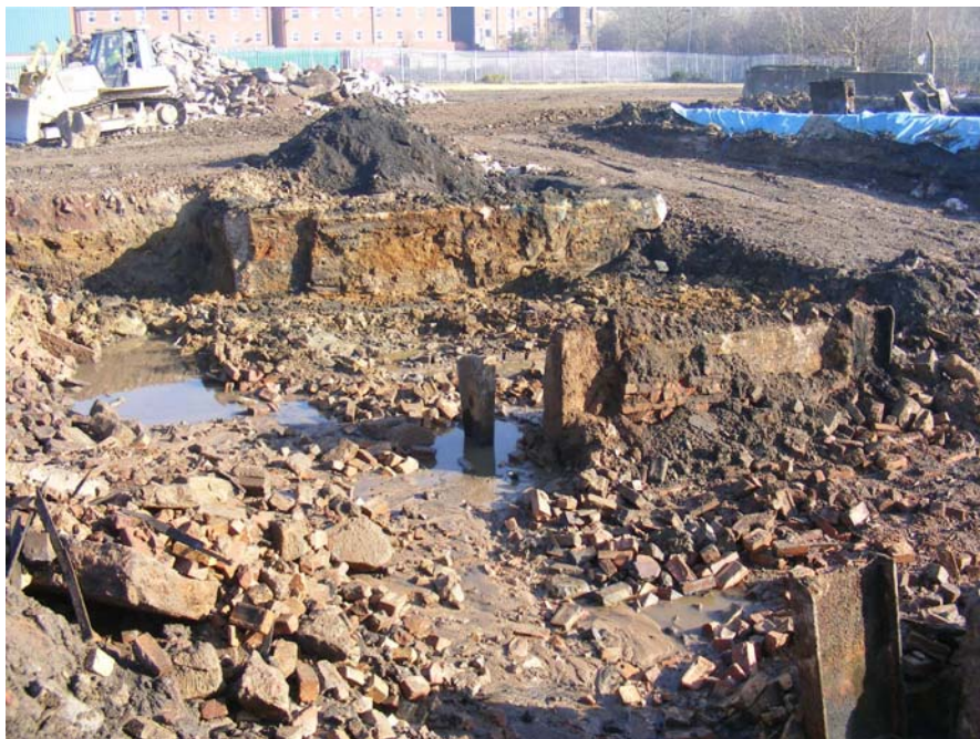
Plate 6: View looking east of a row of RSJ's [007] and structure [009] comprising of two parallel concrete walls and a red brick pad
