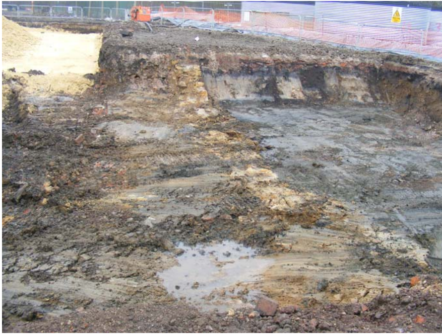
Plate 3: External sandstone wall [004] of the Exhauster House in the western half of Area 2; looking south
