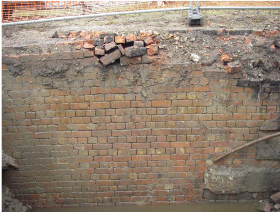
Plate 17: Gasholder No. 2: two large sandstone blocks laid into the inner face of the red brick structure
