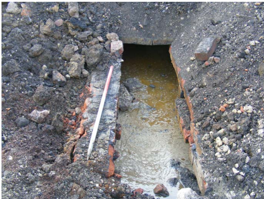
Plate 10: Red brick drain [017] with a sandstone slab top concrete base recorded in the Exhauster House
