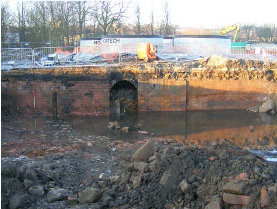
Plate 7: Concrete vaulted arch [008], possibly being a flue within Area A2; looking south-west
