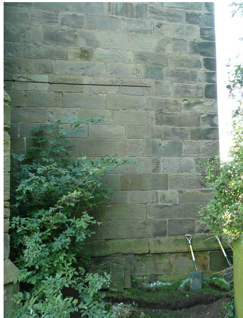
Plate 6 Scar of building against the north wall of the tower
