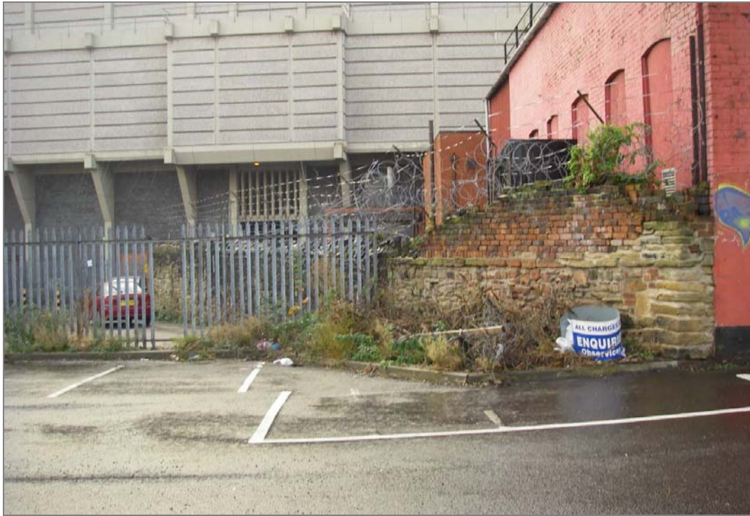
Plate 3 – Stone wall at southern side of site, formerly part of the Corporation's stone yard, viewed facing southeast
