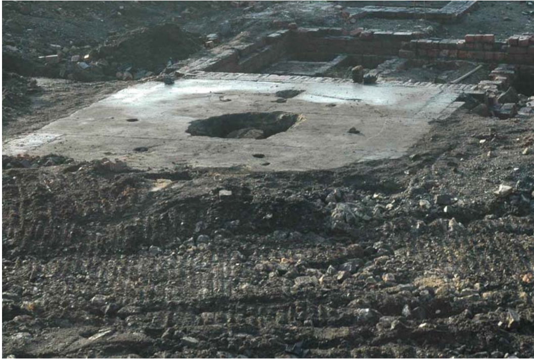
Plate 3: Facing site WSW, showing the large crane base in Trench A. Note the circular groove and fixing bolts.
