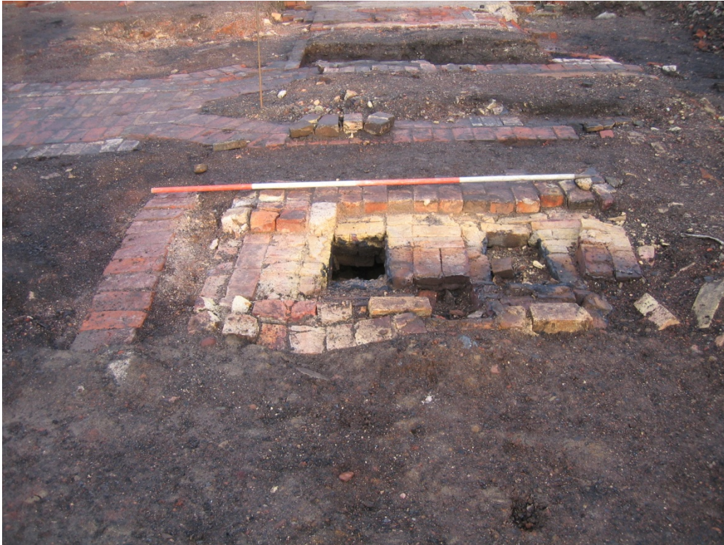
Plate 23: Facing site N. Showing the flues in the upper part of gas regenerator Alpha prior to excavation. These flues linked the hot and cold air chambers beneath (see plate 15 above) allowing hot air to circulate around the structure.
