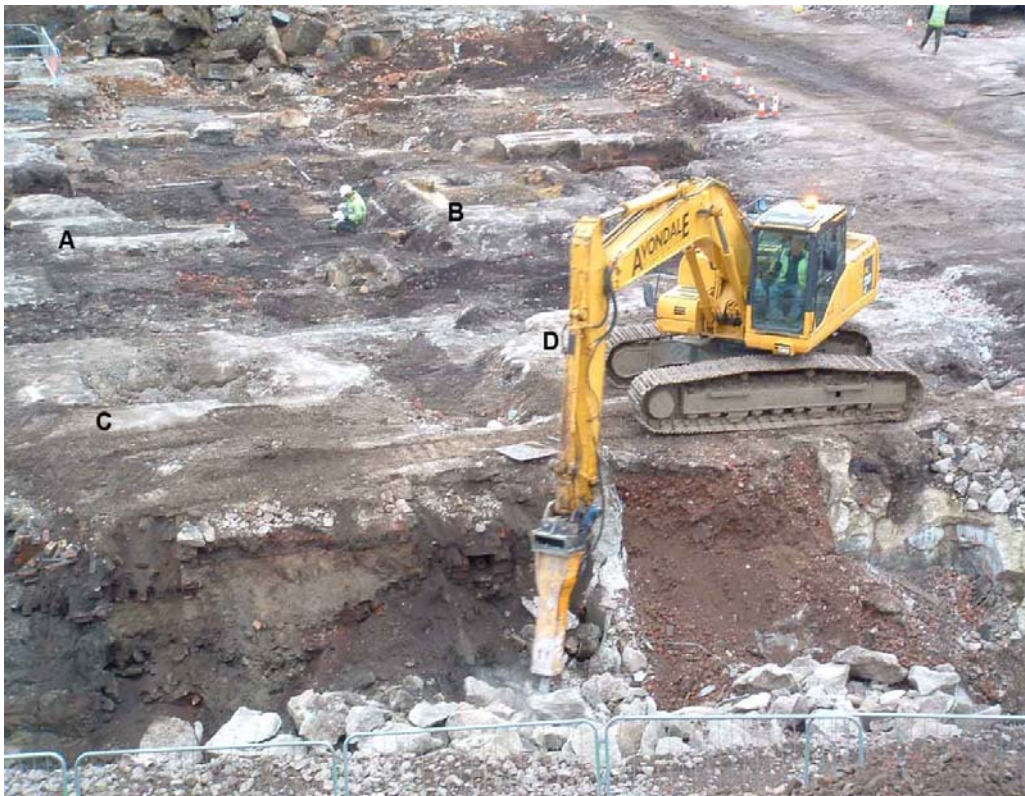
Plate 17: Facing site SSW. Showing the large modern tanks (A – D) possibly associated with the Doncasters factory on strip & record Area 2. Note that the features were being recorded whilst ground reduction was taking place.
