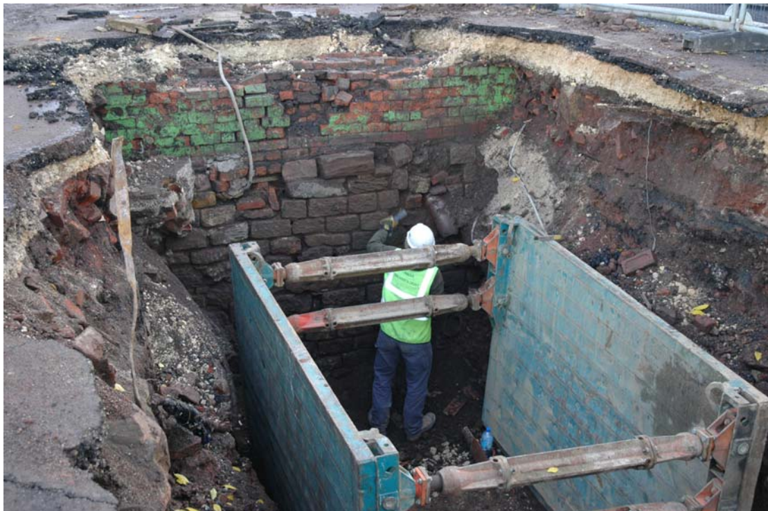
Plate 8: West facing section of Trench 4 showing stone wall (409) with walls (403 & 404) directly overlying
