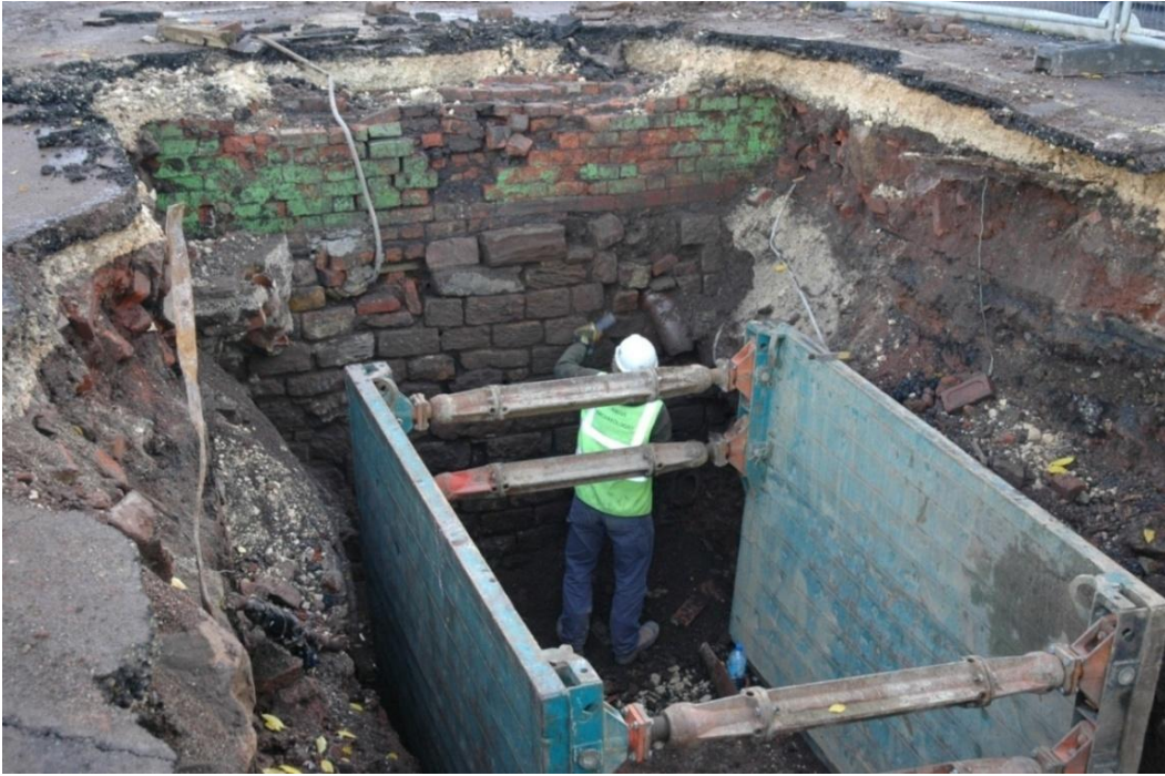
Plate 11: Facing ESE showing the western market hall walling as uncovered in Trench 4 [409].
