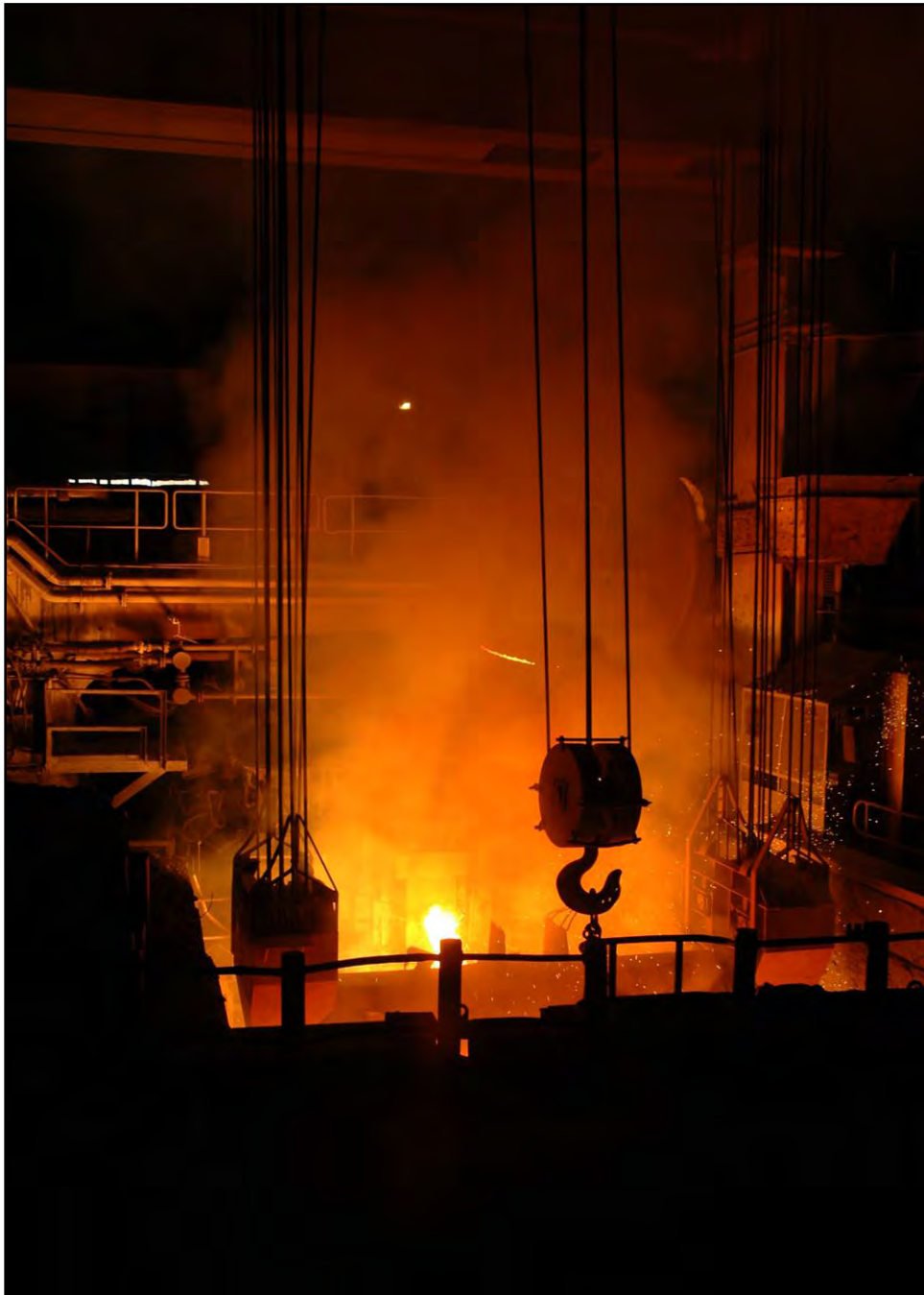
Plate 59: As soon as the chemical and physical properties of the melt are within specification the furnace is tilted and molten steel is tapped into a waiting ladle
