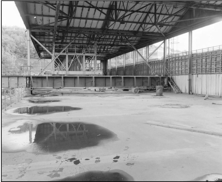
Plate 23: General view of Interior of top floor of building A1, noting gantry and end of travelling crane (film 10:8)
