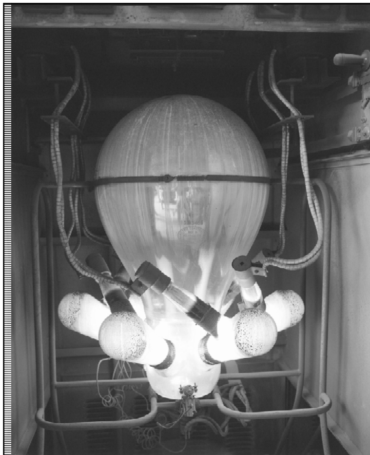
Plate 28: Detail of mercury arc rectifier in building A1 (film 11:9)
