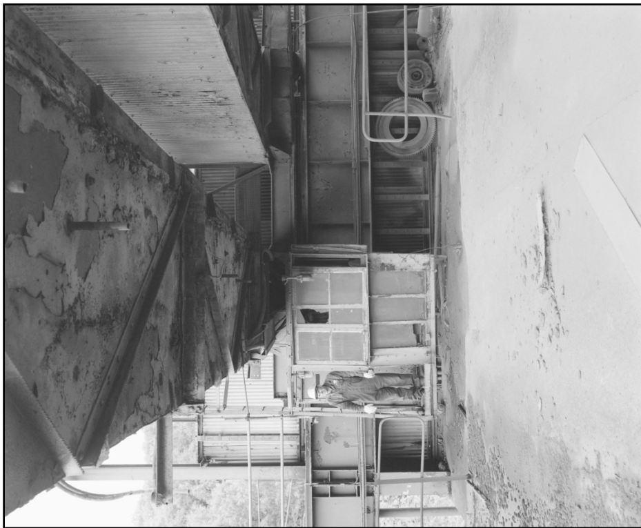
Plate 25: Detail of cab on overhead crane (film 11:4)
