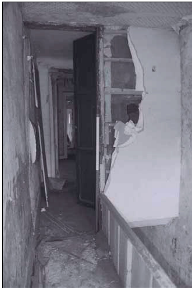
Plate 22: General view of F3, noting glazed panel to cupboard above stairs (film 7.34)
