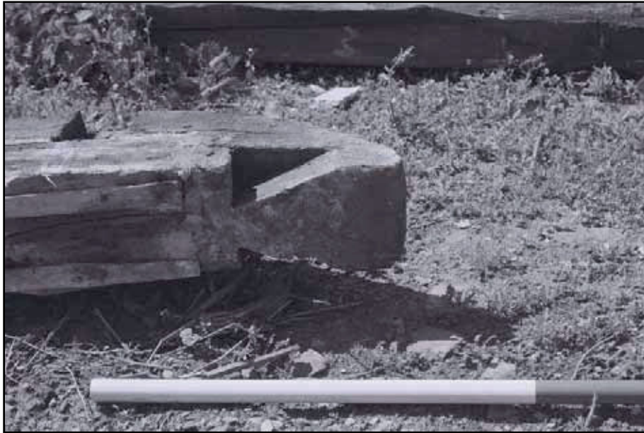
Plate 61: Detail of lapped dovetail joint on tie beam from East Range (film 8.15)
