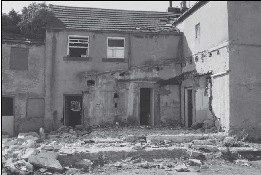
Plate 45: General elevation of north elevation of East Range after demolition of later lean-to (film 8.32)
