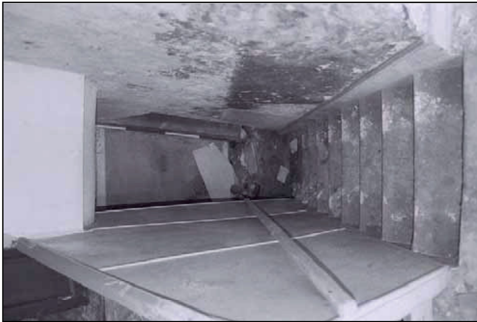
Plate 13: General view of looking down stairs from the first floor to G3 (film 7.23)
