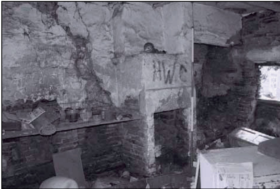
Plate 53: General view of G10, noting hearth and low flues in wall beneath shelf (film 1.04)
