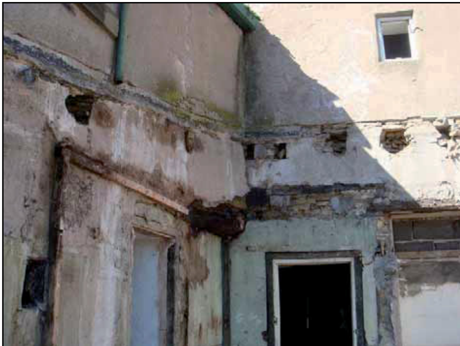
Plate 46: General view of jettied out wall on west side of north elevation of East Range
