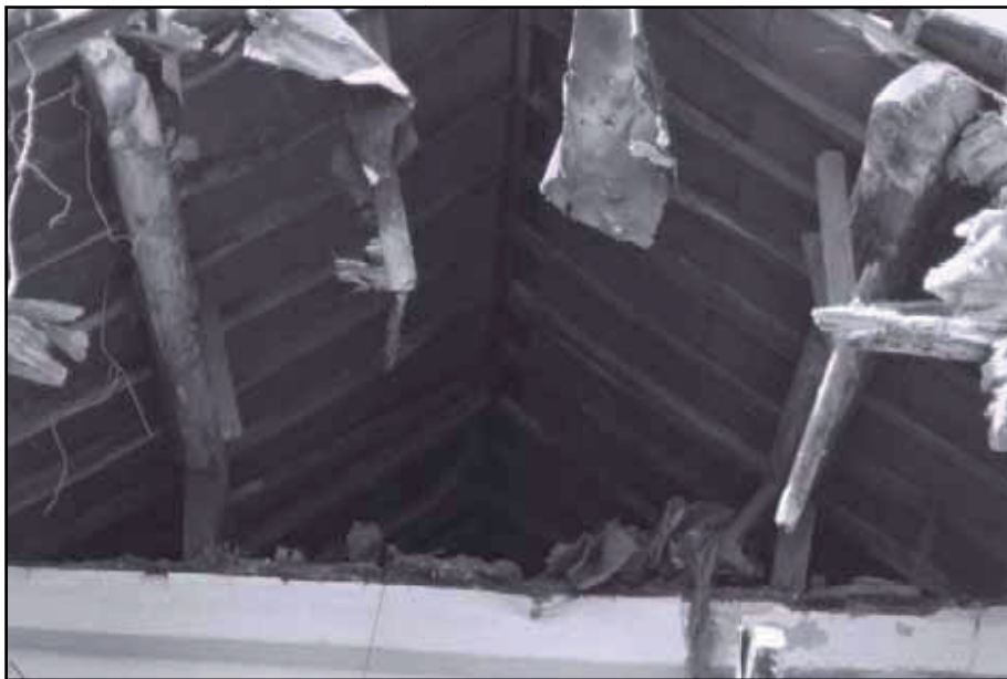
Plate 60: Detail of roof structure of East Range, noting large oak purlins and timber struts supporting them (film 8.18)
