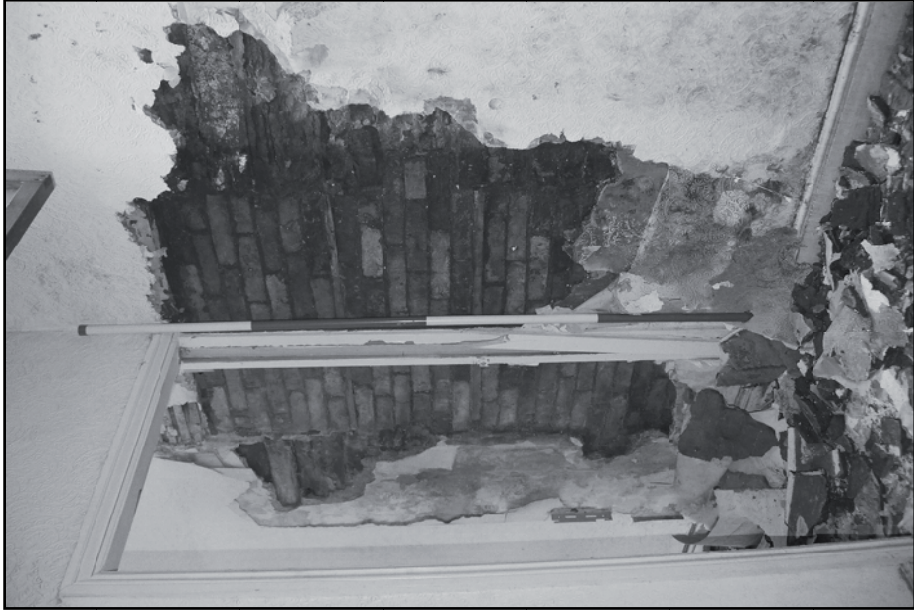
Plate 44: Detail of blocked doorway in east wall between F9 and F10 (film 7.3)
