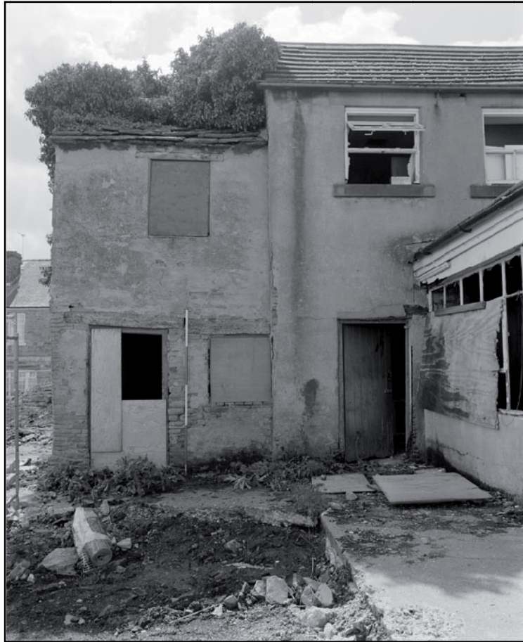
Plate 47: General view of east end of north elevation of East Range (film 3.7)
