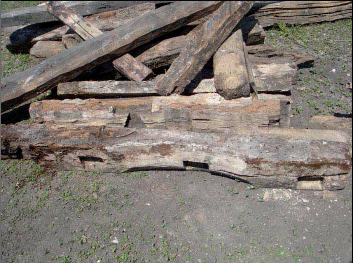
Plate 63: Detail of arched lintel reused as a wall plate in the East Range. Note the studding around the arch to support plastering and the inserted sockets for the rafters.
