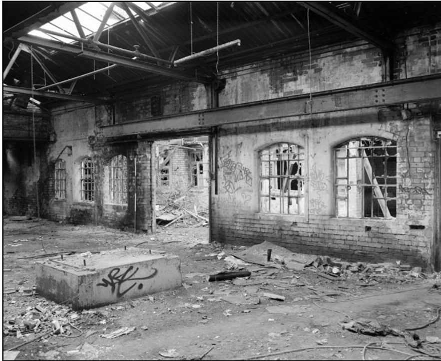
Plate 45: General view of internal east wall of range to east of eastern courtyard (film 8.06)
