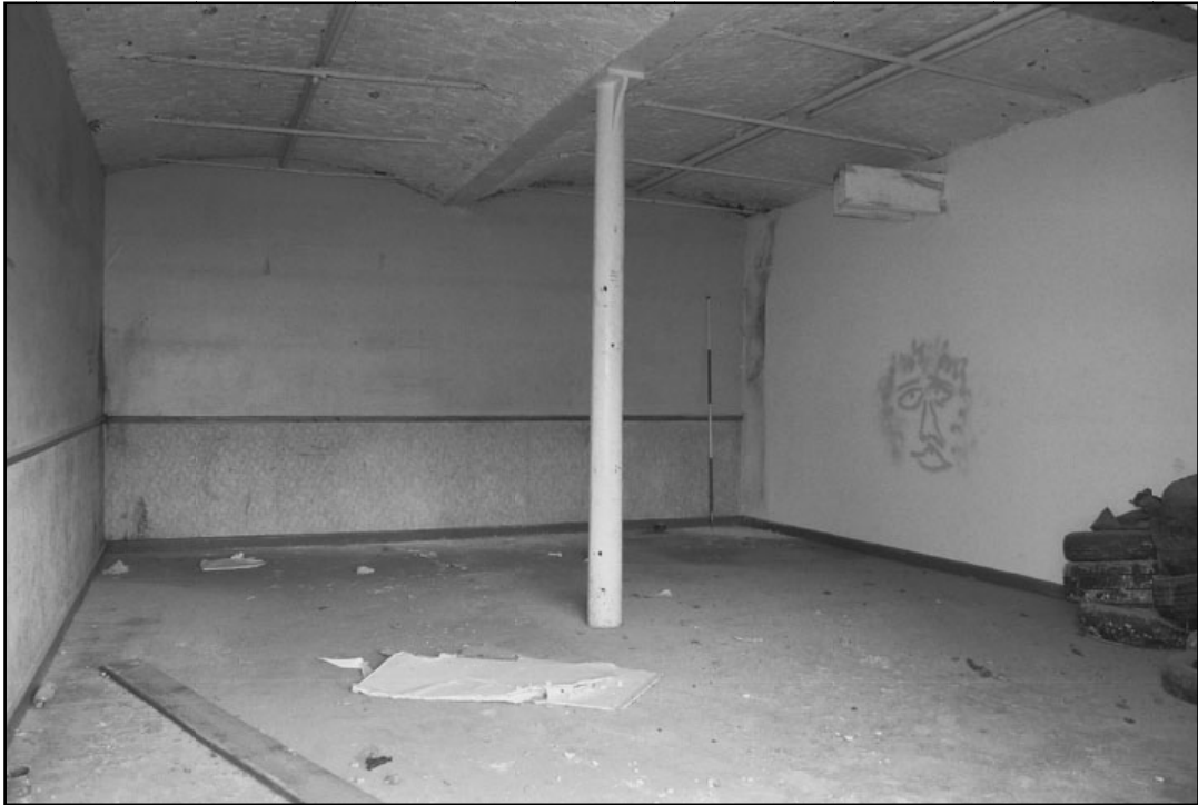
Plate 32: General view of room 2G1, noting jack arch ceiling and cast iron column (film 9.12)
