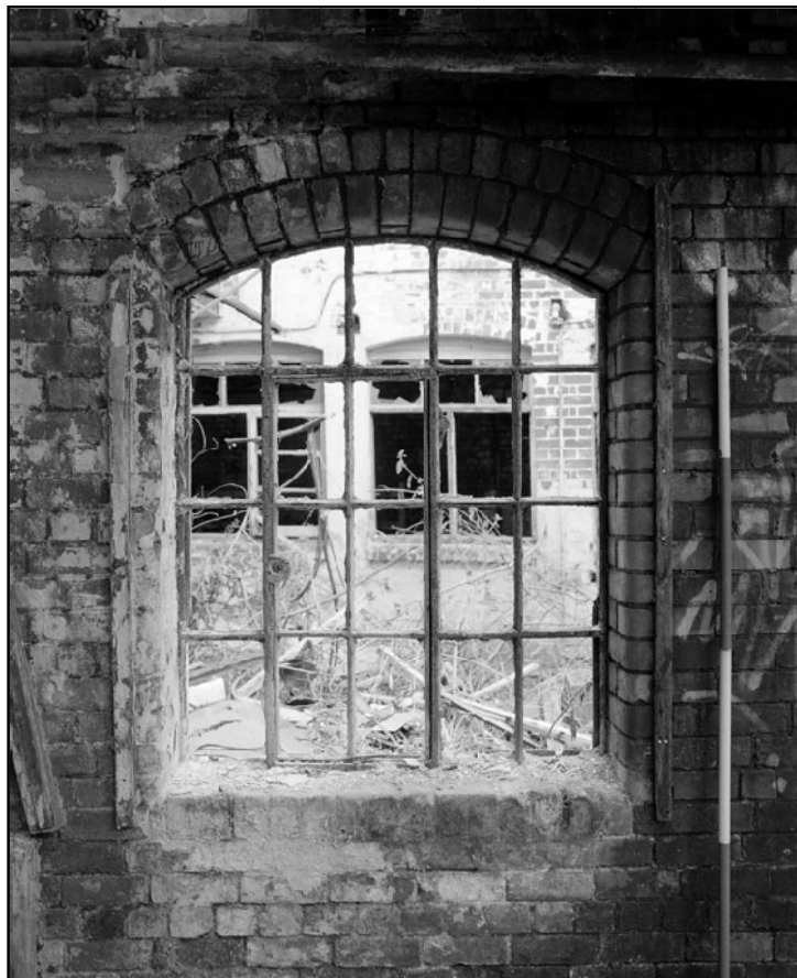
Plate 46: Detail of window in east wall of range to east of eastern courtyard (film 8.07)
