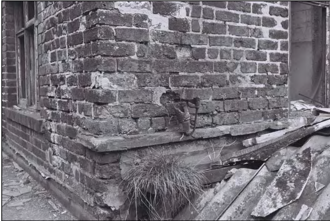
Plate 30: Detail of first floor stringcourse on south elevation of grinding workshop (film 1.27)
