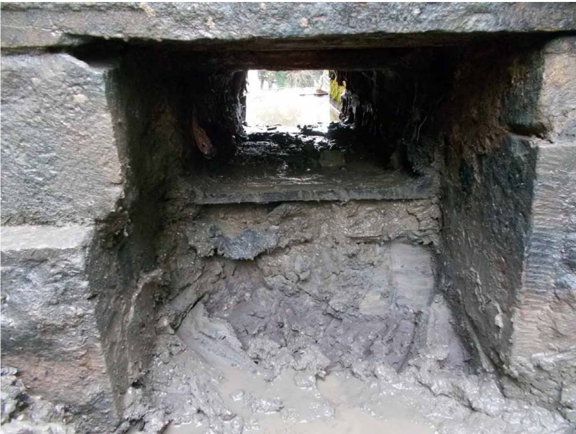
Plate 22. Completed excavation with same clay extending below base of culvert and dam footing, viewed from east.
