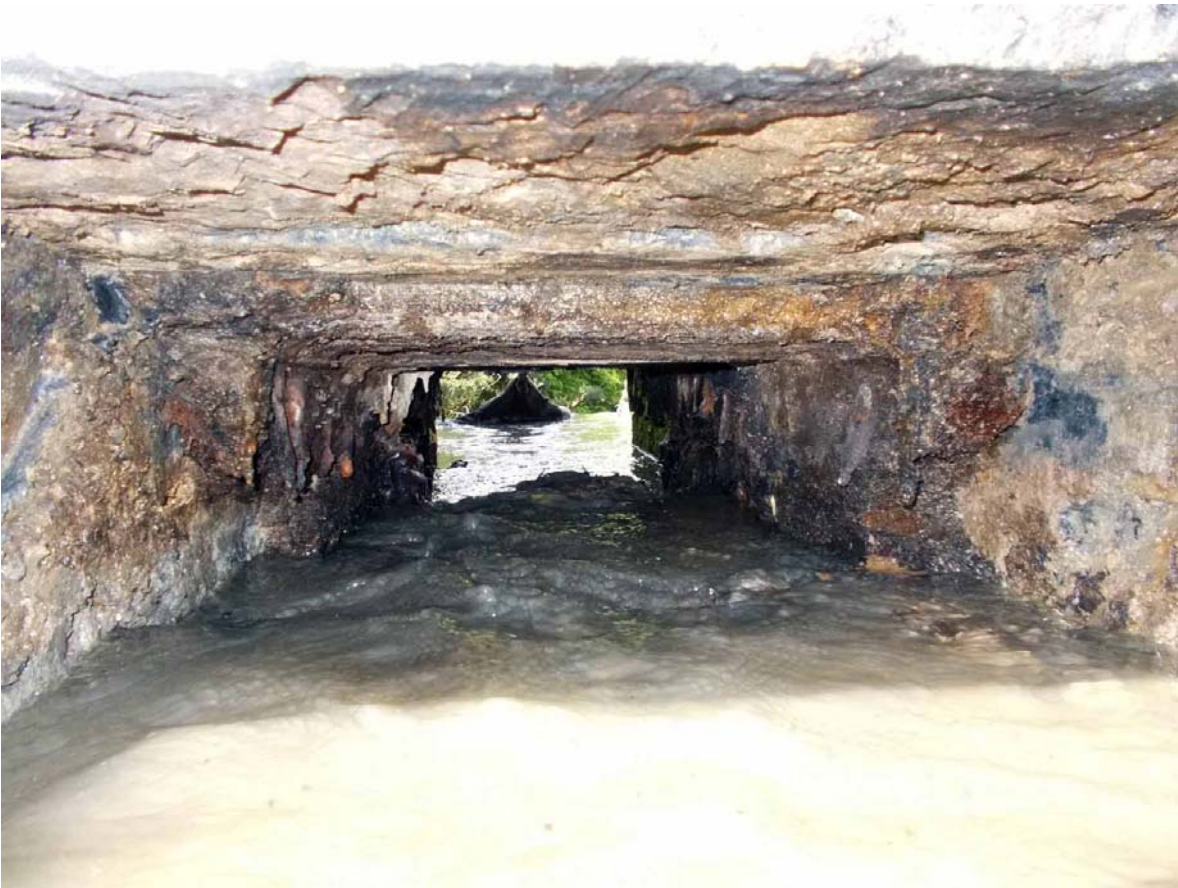
Plate 20. Culvert aperture beneath dam, with remains of timber culvert, viewed from east.
