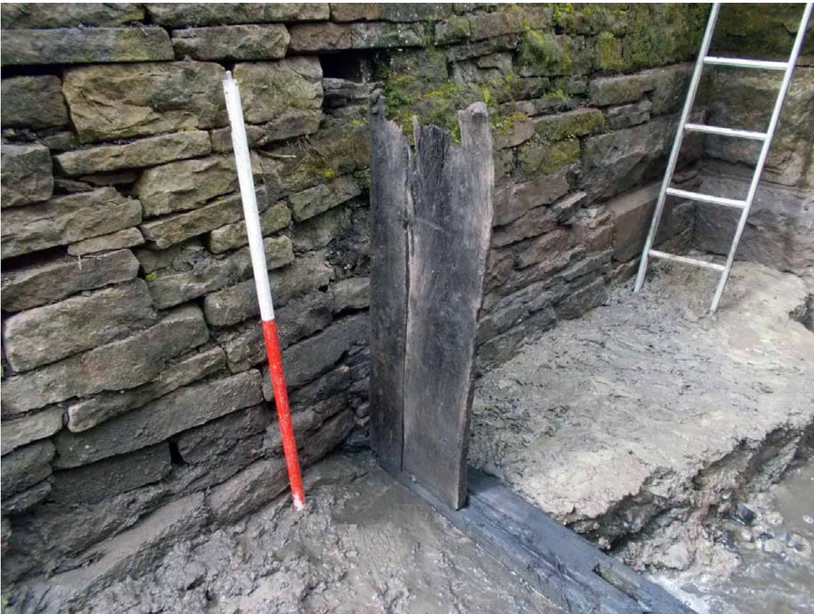
Plate 18. Base rail and partly reassembled barrier/fence. Note decayed top rail within recess, near top of photo, viewed from north-east.
