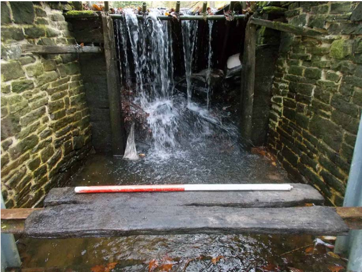
Plate 33. Worn drop board removed from original structure, visible in background, viewed from west.
