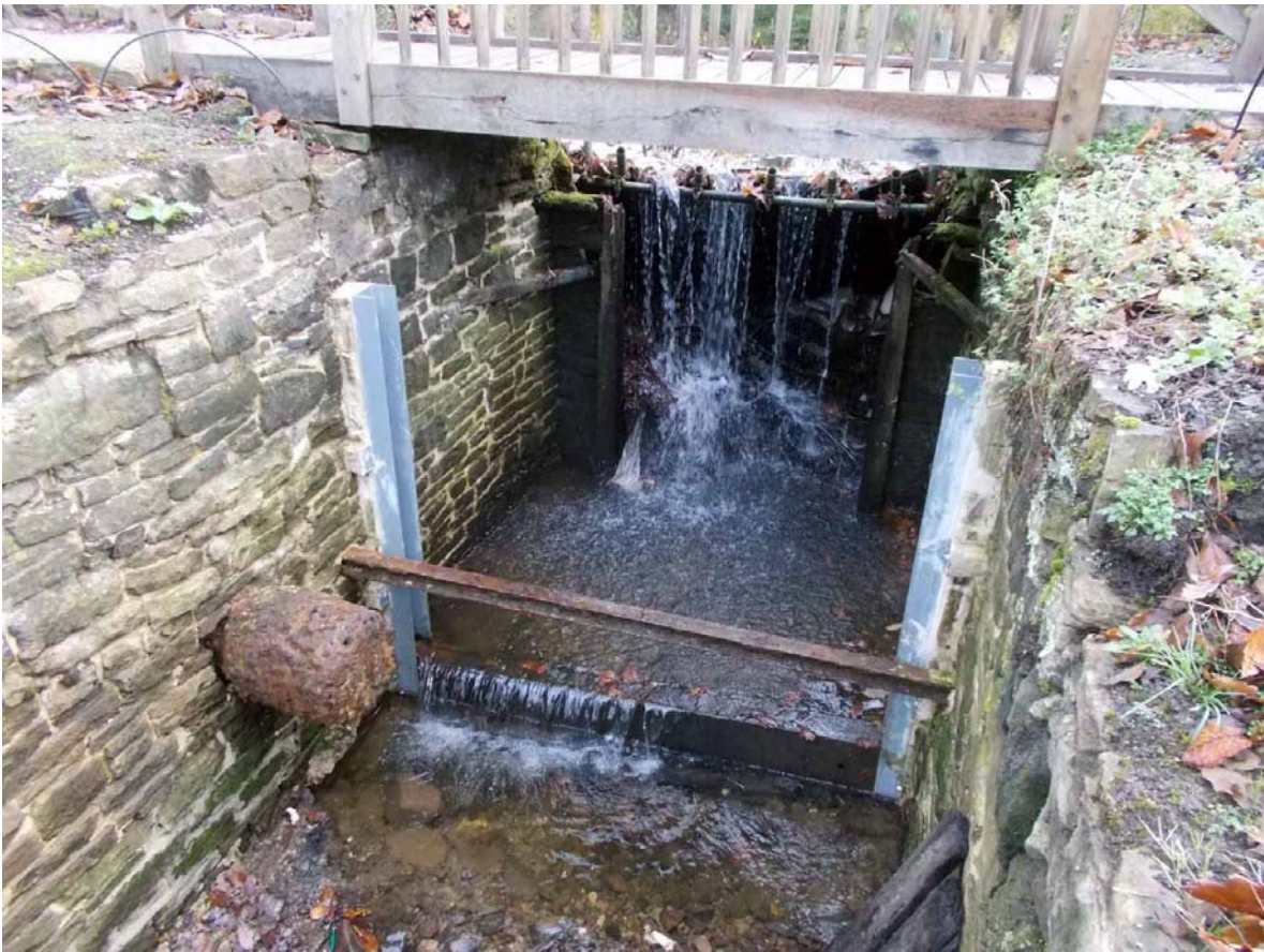
Plate 31. New drop board sluice and bridge, at east end of canal, 30 Oct. 2017, from west.
