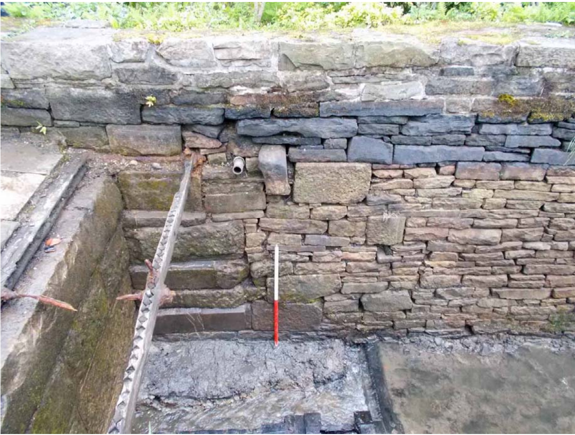
Plate 24. North side wall of canal nearest to the dam, viewed from south.
