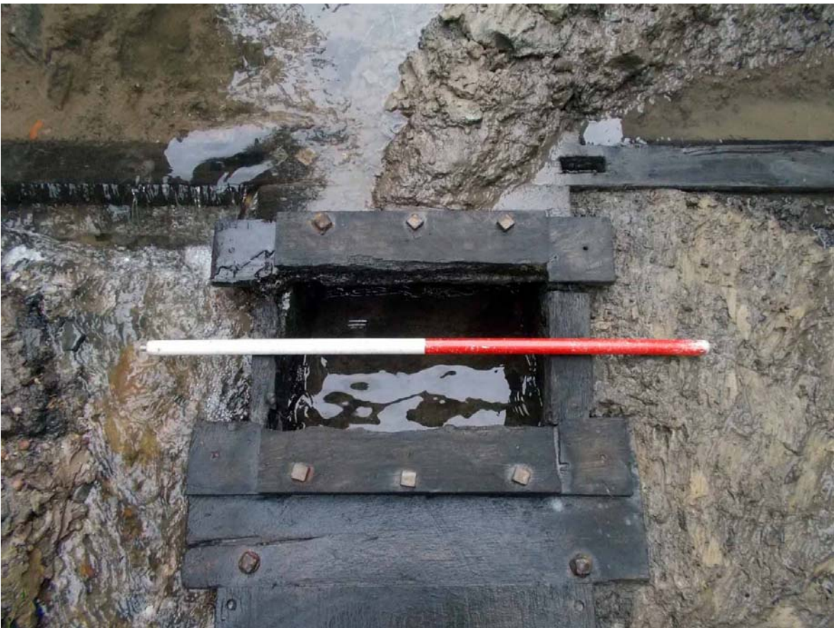
Plate 6. Culvert intake at east end, with flange plate removed (Plate 13), viewed from west.
