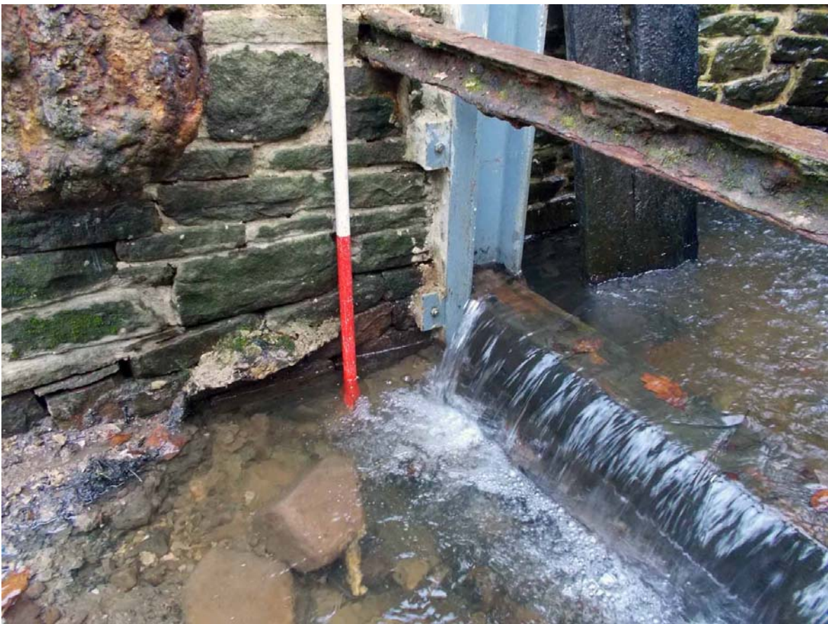
Plate 32. Detail showing north side wall, extending 0.22m below top of puddled clay, viewed from south.
