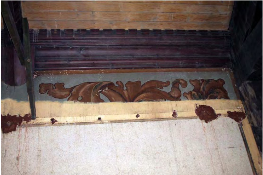
Plate 17. Bay 4, east elevation, remnant of decoration under eaves.
