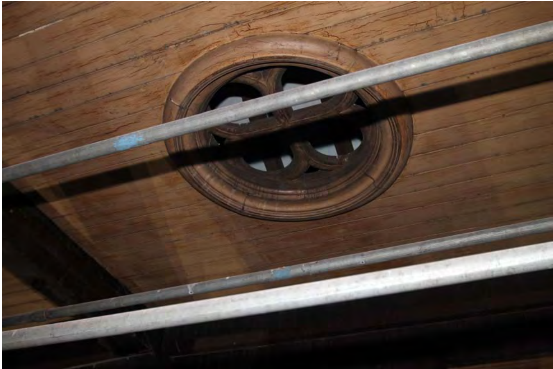
Plate 13. Timber roof lining above truss 4/5, detail on ventilation aperture, viewed from north-west.
