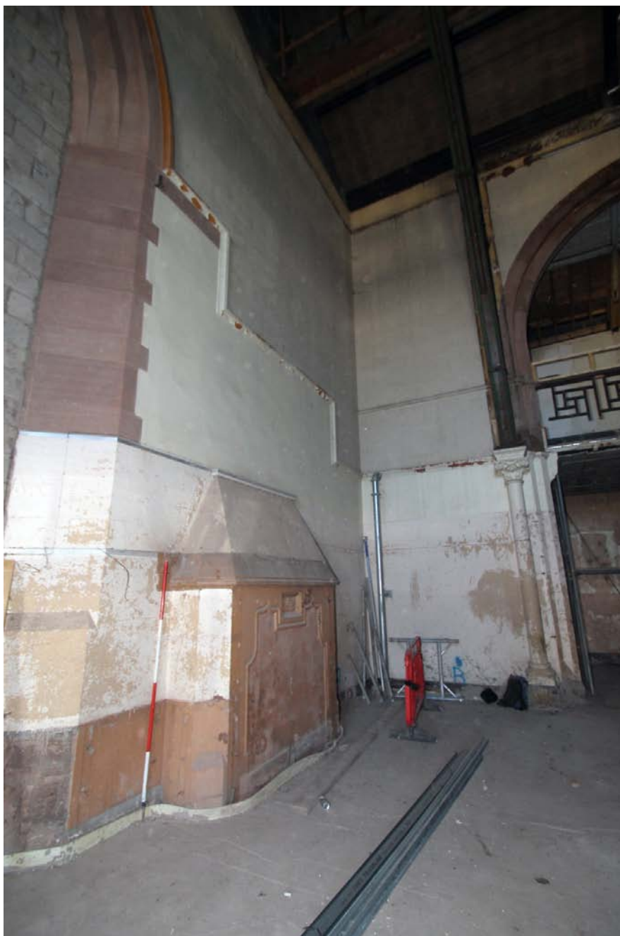
Plate 27. Bay 8, east section of north elevation, showing blocked fireplace location, viewed from south-west.
