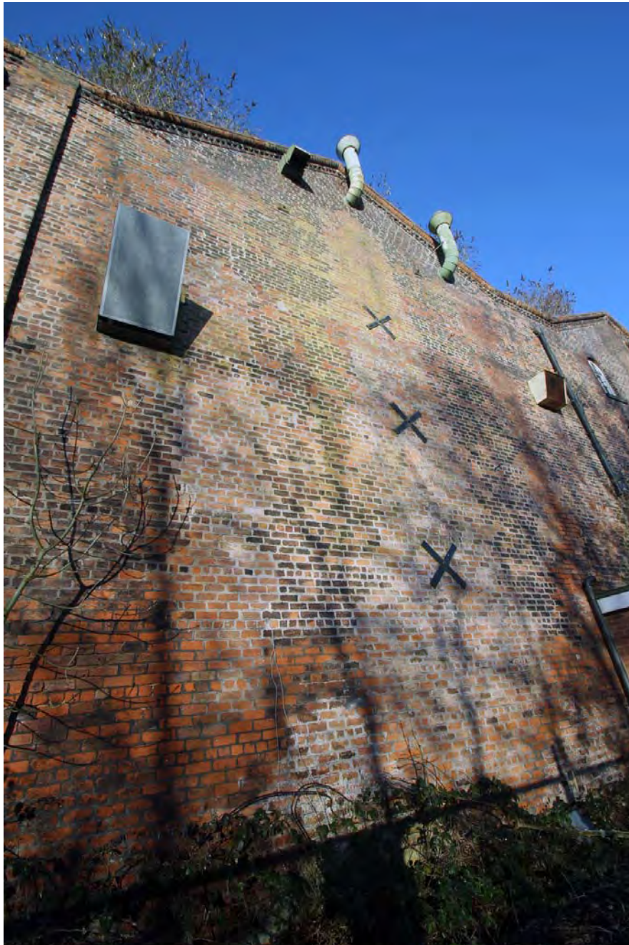
Plate 68. Warehouse Central Bay (Building 1B), viewed from east, line of blocked taking-in doorways can be seen where pattress plates are affixed.
