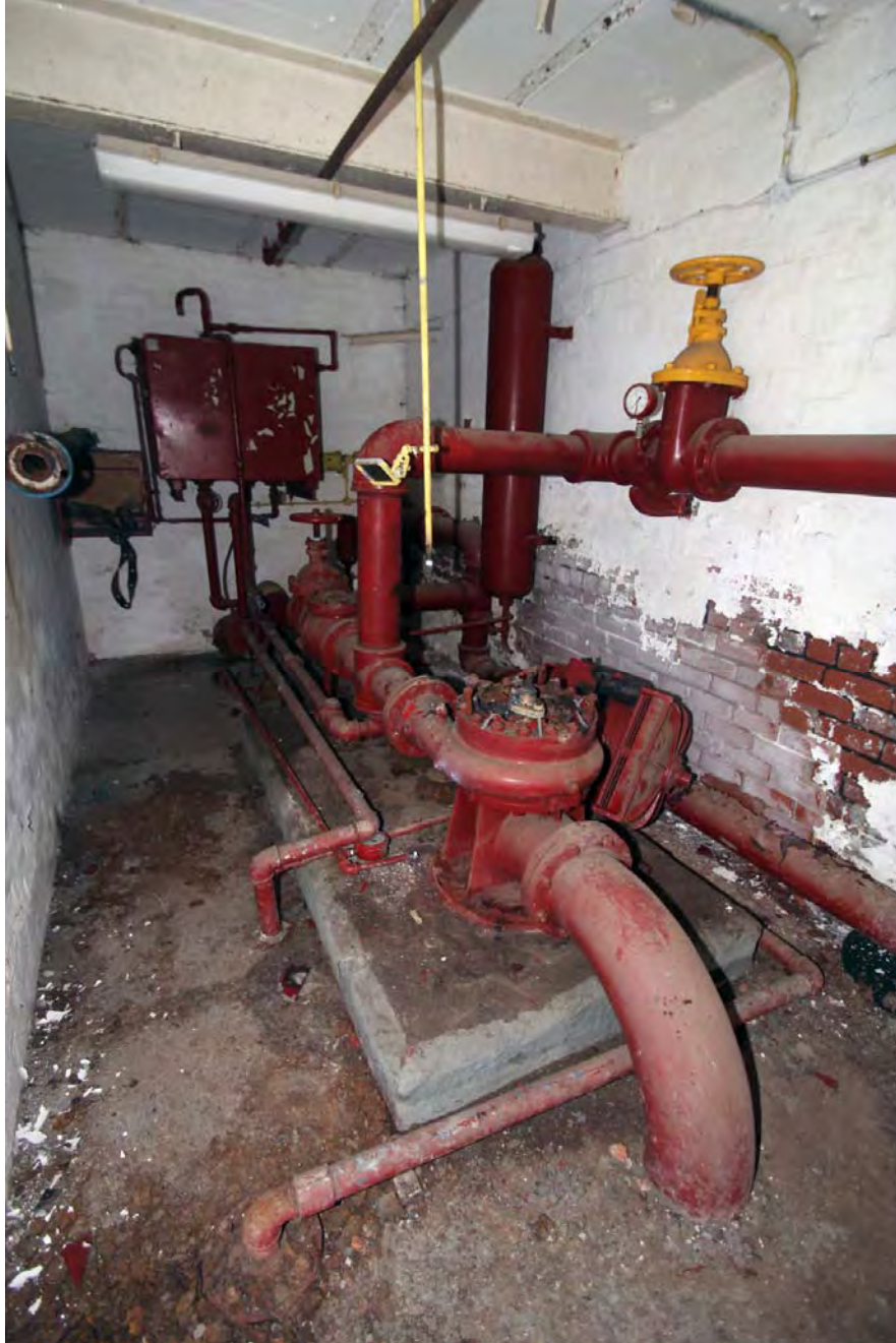
Plate 60. Pumphouse (Building 12), ground floor, pump mechanism, viewed from north.
