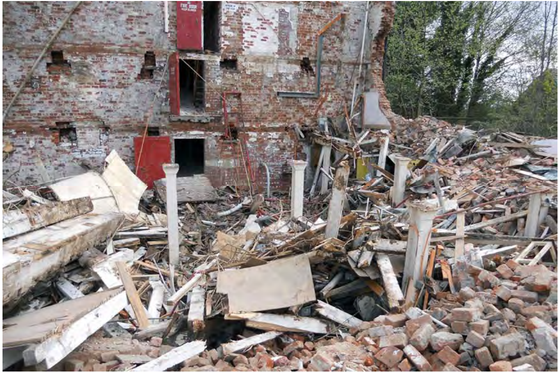
Plate 79. Warehouse Northern Bay (Building 1A), showing ground floor wrought-iron columns, following demolition.
