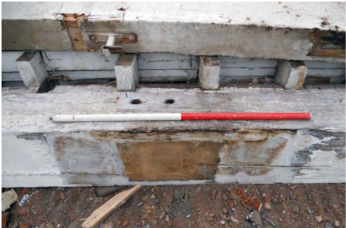
Plate 72. Warehouse Southern Bay (Building 1C), ex situ timber beam, showing soffit face where timber column located.
