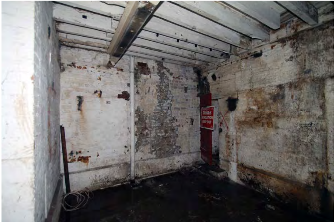
Plate 43. Former Beam Engine House (Building 11), ground floor, northern part, viewed from north-west.
