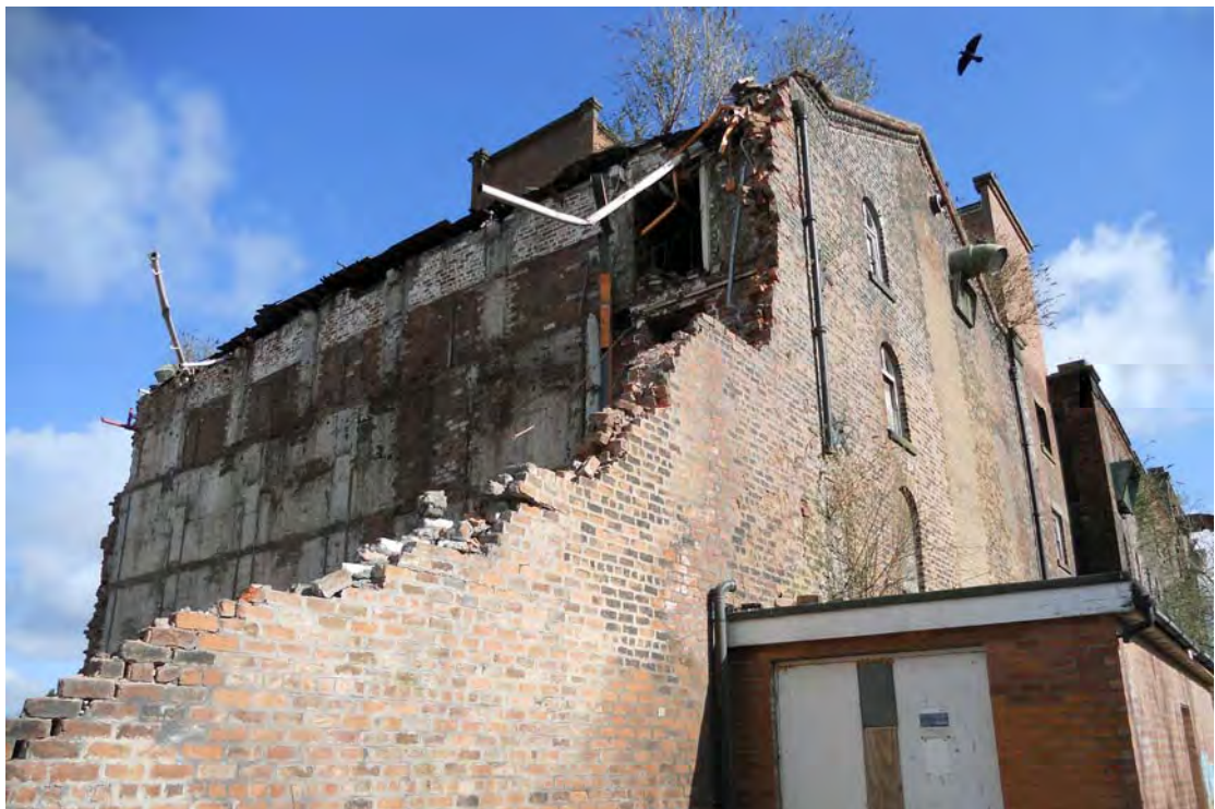
Plate 76. Warehouse Northern Bay (Building 1A), about to be demolished, viewed from south-east.
