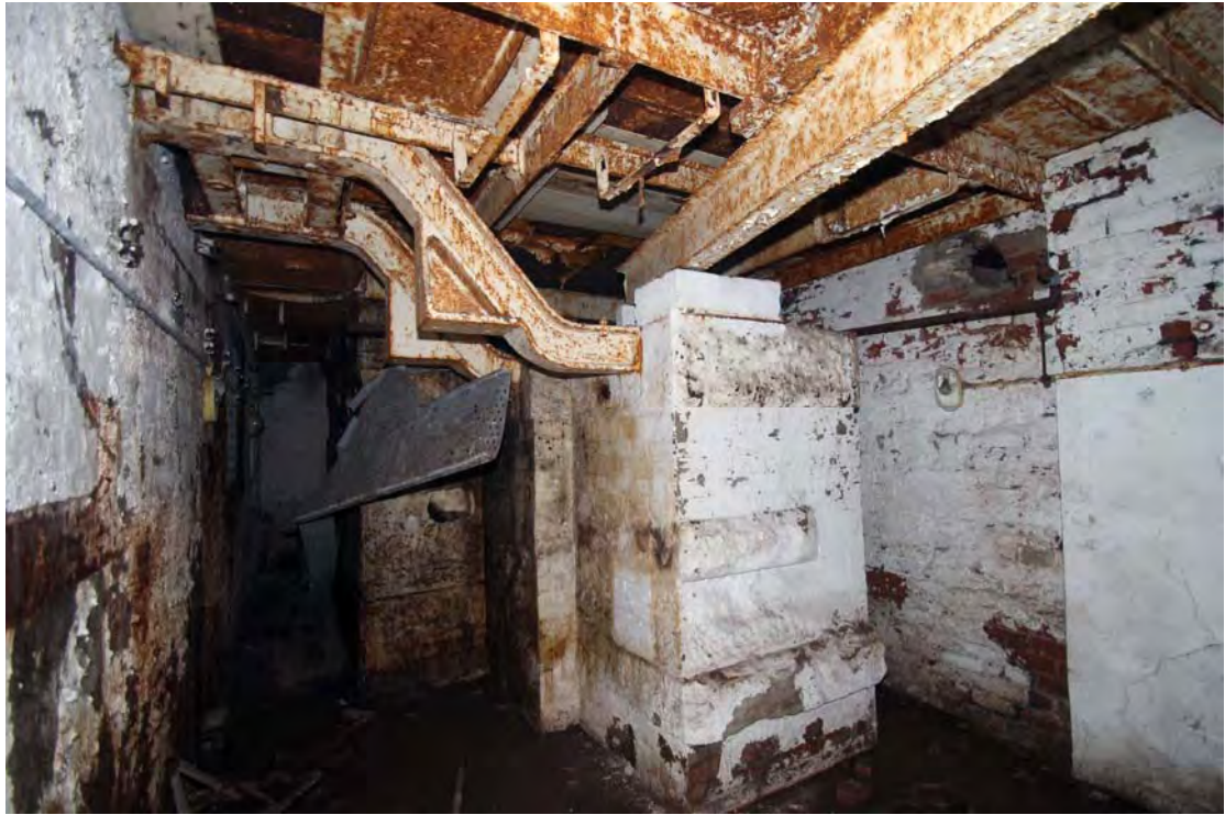
Plate 27. Engine House (Building 8), basement, viewed from east, showing cylinder bed in centre, and inserted ironwork to support later engine.
