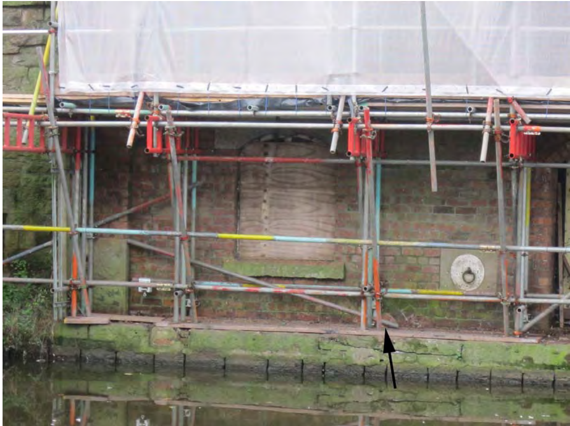
Plate 9. Boiler house east part (Building 9), viewed from north. Blocked arch for boiler blowdown pipes arrowed.
