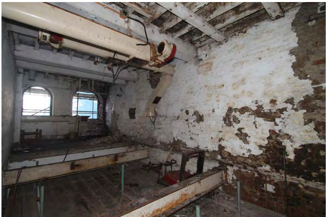
Plate 32. Engine House (Building 8), second floor, viewed from north-west, original timber ceiling over.
