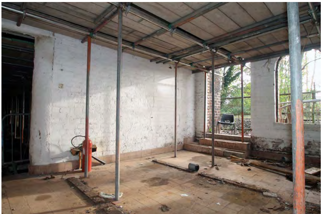
Plate 67. Building 2, first floor level, view from south-west, looking out onto railway Embankment.
