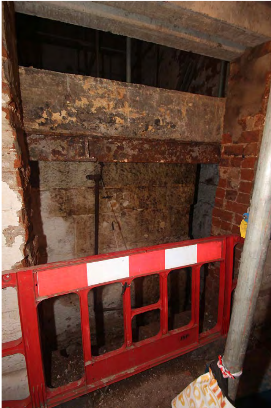
Plate 24. Looking into Engine House (8), from base of Stair Tower (7), viewed from west. Gritstone engine bed is topped by an iron kerb, which in turn has had a thick concrete floor poured onto it.
