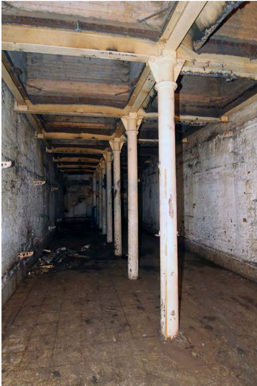
Plate 48. Building 17, ground floor, view looking northwards, large double doorway visible on right (east) side.
