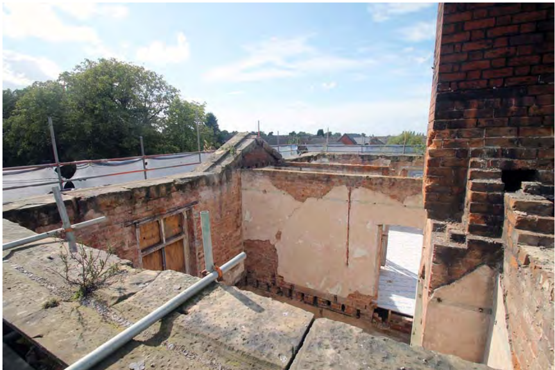
Plate 96. Mansion House, first floor, looking over room F2 towards pediment, viewed from north-east.
