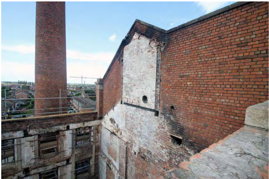
Plate 52. Building C, after fire, north internal wall, showing outline of clerestory.
