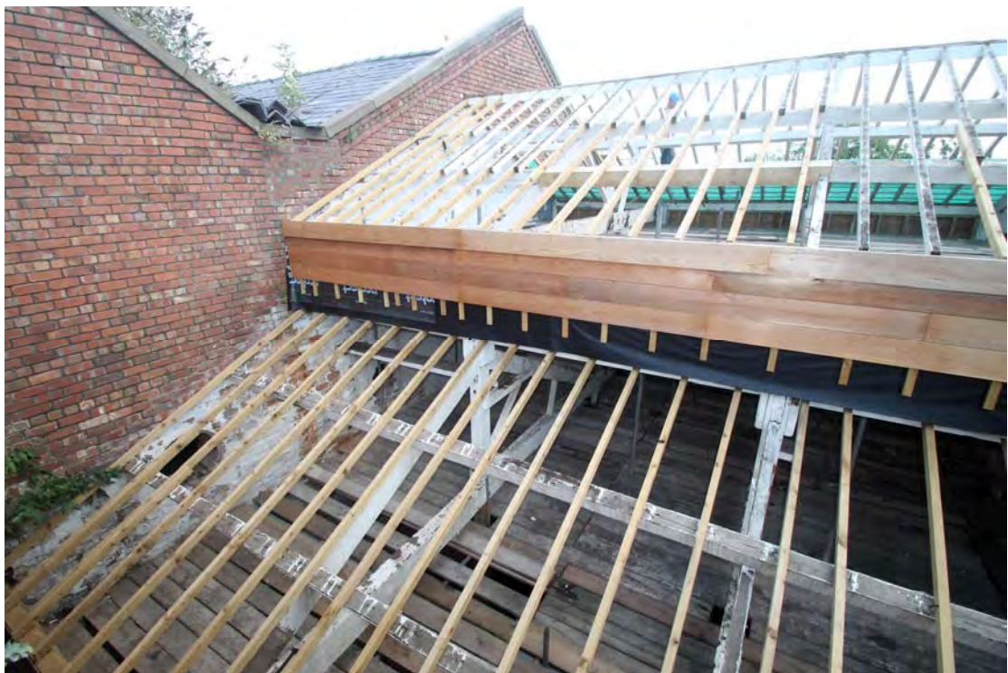
Plate 38. Original mill (Building 6), roof structure being replaced upon original timber king-post trusses.
