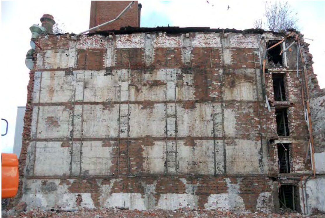
Plate 75. Warehouse Northern Bay (Building 1A), about to be demolished, viewed from south.
