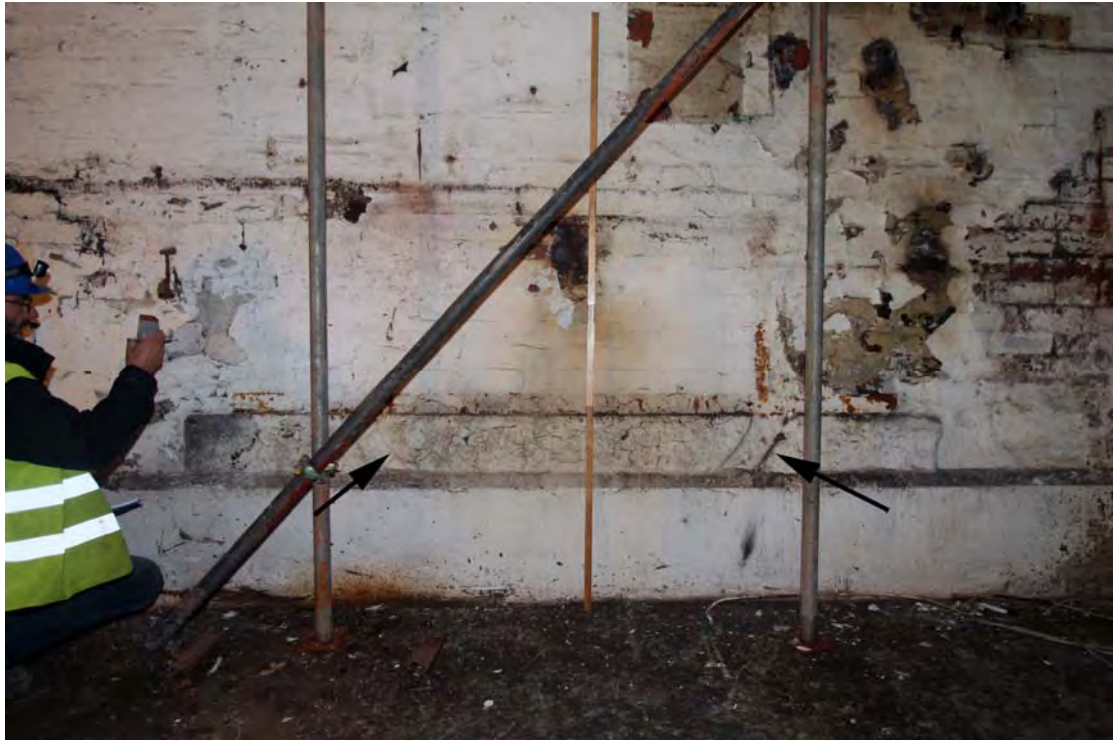
Plate 45. Former Beam Engine House, ground floor, south wall, showing blocked aperture with gritstone bed beneath, with circular score marks (arrowed), from pinion wheel on first motion shaft.
