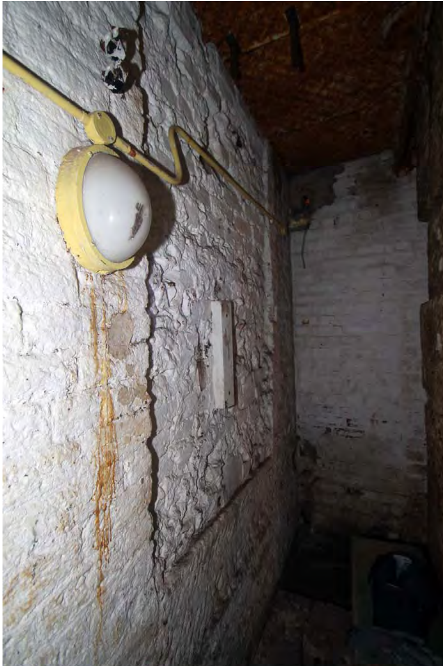
Plate 26. Engine House (Building 8), west end of south wall, showing first motion shaft housing, viewed from north-east.
