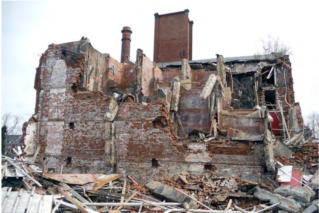
Plate 73. Warehouse Central Bay (Building 1B) under demolition, viewed from south, showing internal steel silos and concrete columns.
