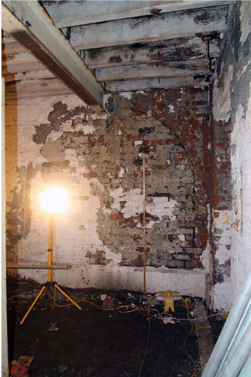
Plate 58. Building 10 (Wheat Receiving Plant), ground floor, viewed from south, showing doorway into Boiler House.
