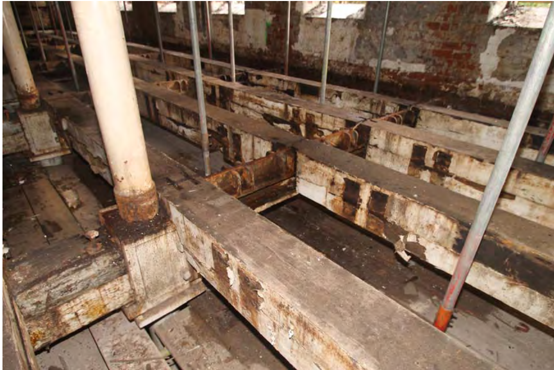
Plate 35. Original mill (Building 6), first floor, viewed from south-west, showing east-west cast-iron floor beams, probably intended to counter lateral thrust of railway embankment raised against east mill wall.
