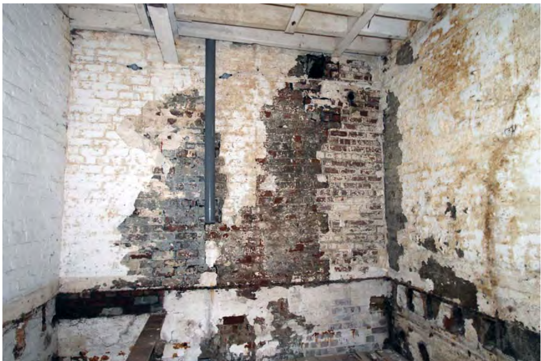
Plate 46. Former Beam Engine House, first floor, east end, blocked doorway to left, previously accessing Stair Tower (Building 7).
