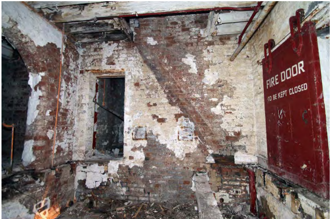
Plate 42. Stair Tower (Building 7), second floor, viewed from west, showing 'ghost' of removed stairs.
