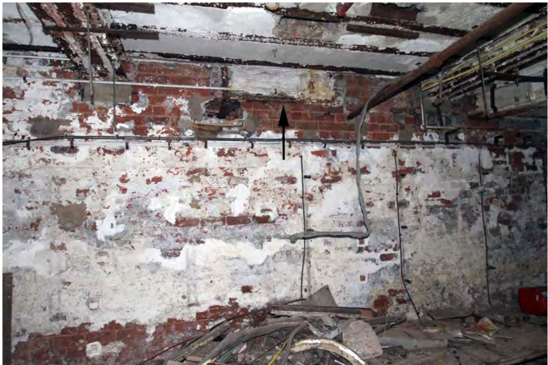
Plate 19. Boiler House ground floor (Building 9), viewed from north. Large cast-iron wallbox, probably related to 1901 inverted vertical steam engine.
