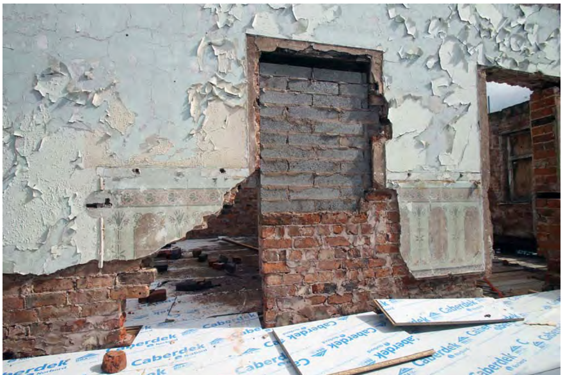
Plate 90. Mansion House, first floor, room F1, viewed from west. Wallpaper suggests location of stairwell.
