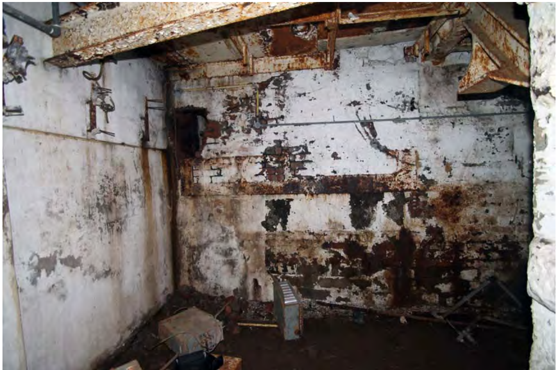
Plate 28. Engine House (Building 8), basement, east end, viewed from north, showing large cast-iron wallbox, now infilled, in centre
