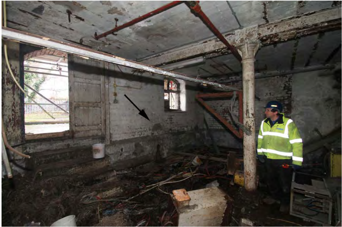
Plate 16. Boiler House ground floor (Building 9), viewed from south-west. Arch in canal wall arrowed, probably for boiler blowdown pipes.
