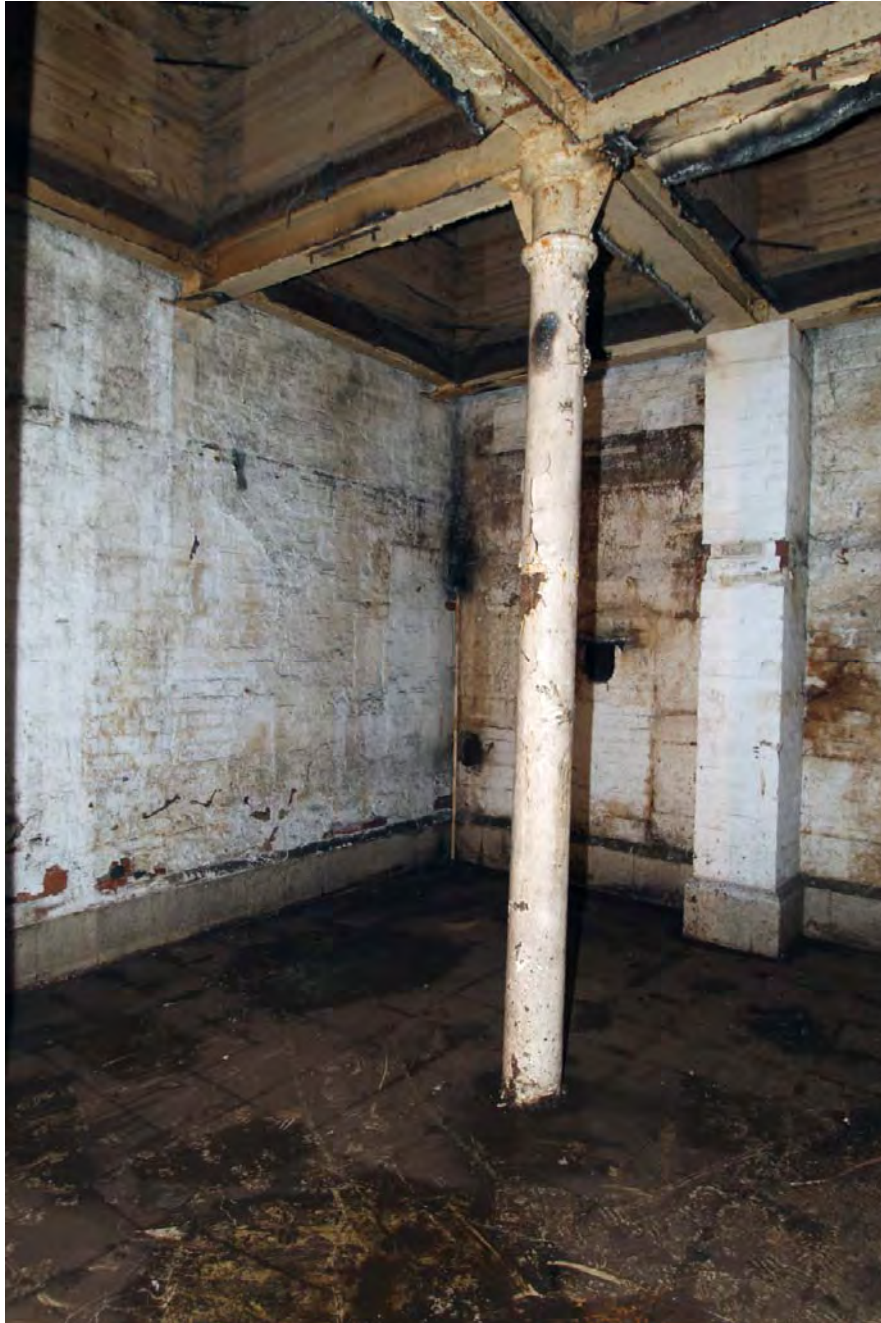
Plate 50. Building 17, ground floor, north end, viewed from south, with gritstone beds related to beam engine house 2 visible behind column, and blocked openings to left.
