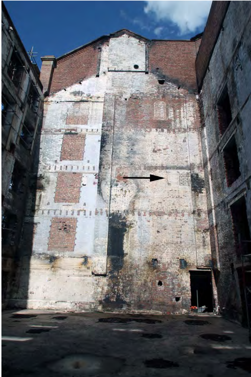
Plate 53. Building C, following fire, north internal wall, with entablature housing for beam engine 2, arrowed.
