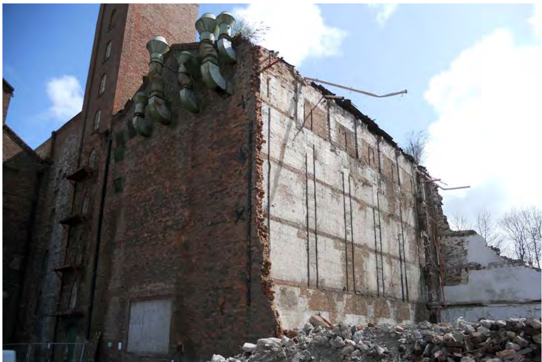
Plate 74. Warehouse Northern Bay (Building 1A), about to be demolished, viewed from south-west.
