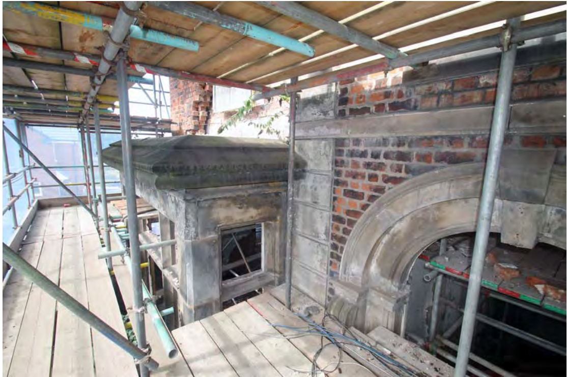
Plate 87. Mansion House, first floor, south elevation, showing upper bay window structure, viewed from south-east.
