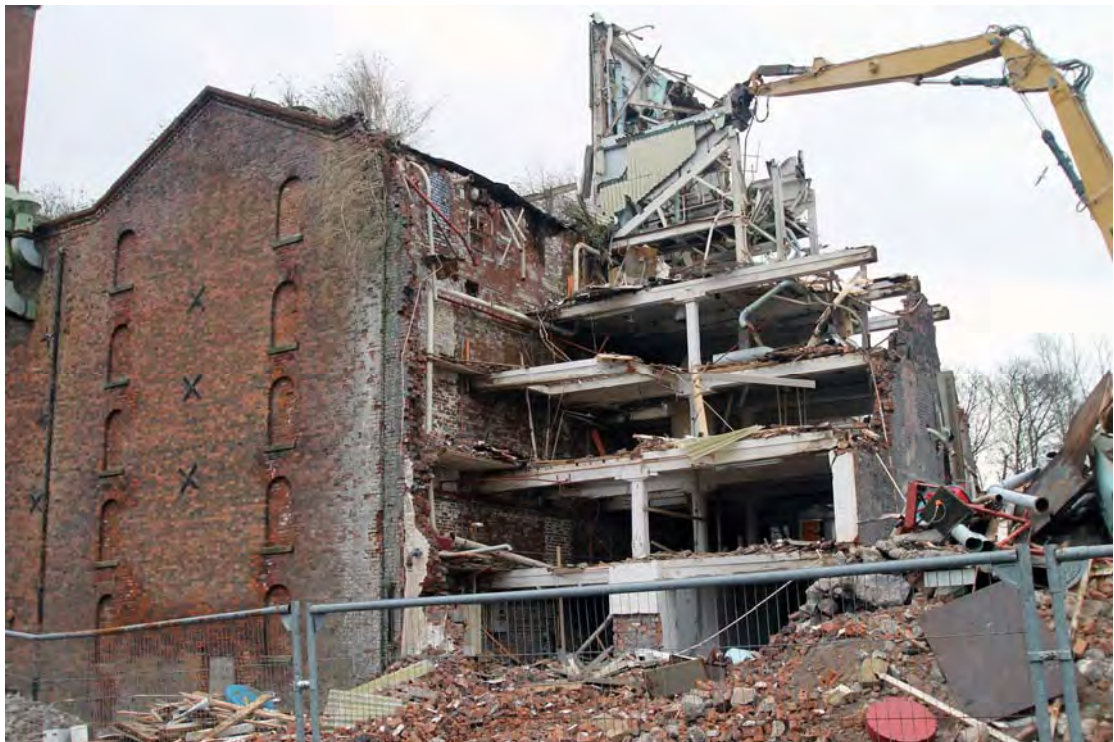
Plate 70. Warehouse Southern Bay (Building 1C) under demolition, viewed from south-west. Note heavy timber beams and columns and roof trusses.
