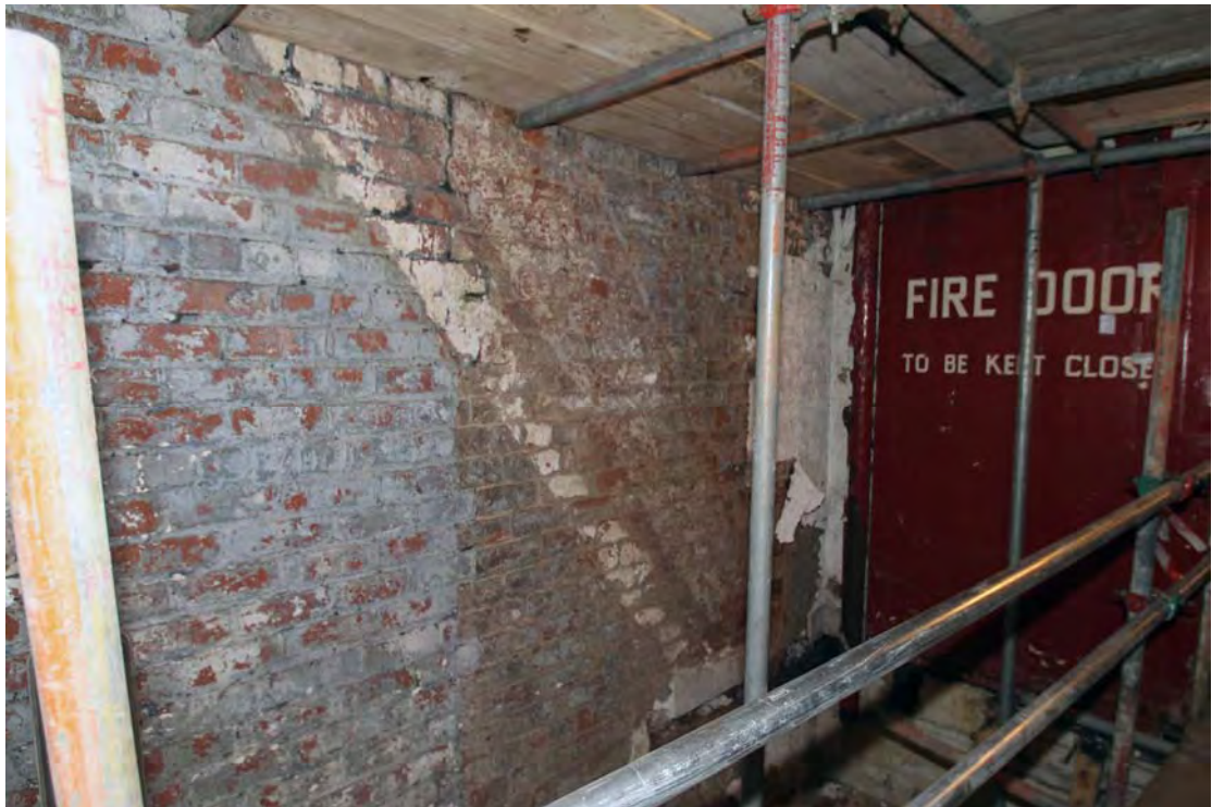
Plate 40. Stair Tower (Building 7), first floor, viewed from north-west, showing 'ghost' of removed stairs.
