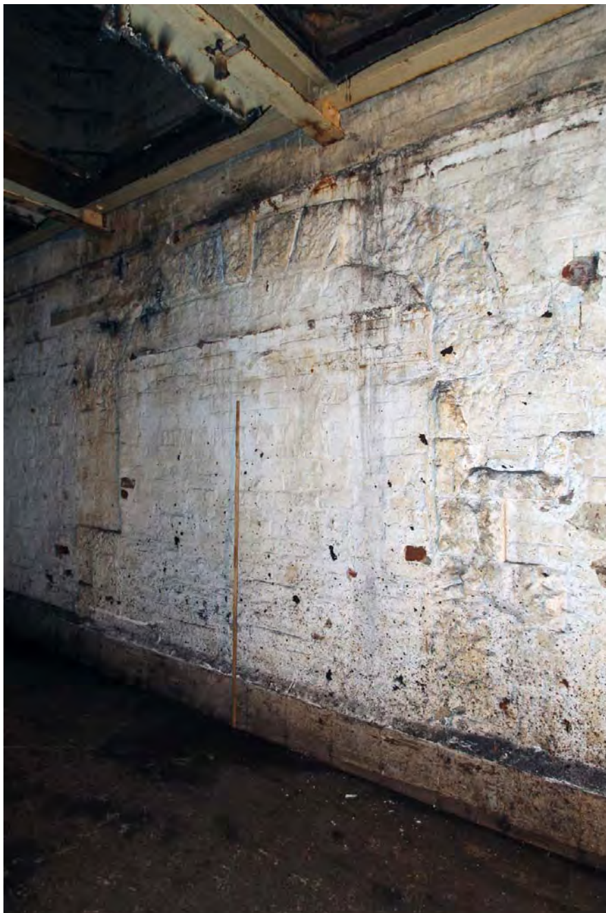
Plate 47. Building 17, ground floor, east wall, double doorway with elliptical head and rusticated voussoirs, which formerly led into Building 6.
