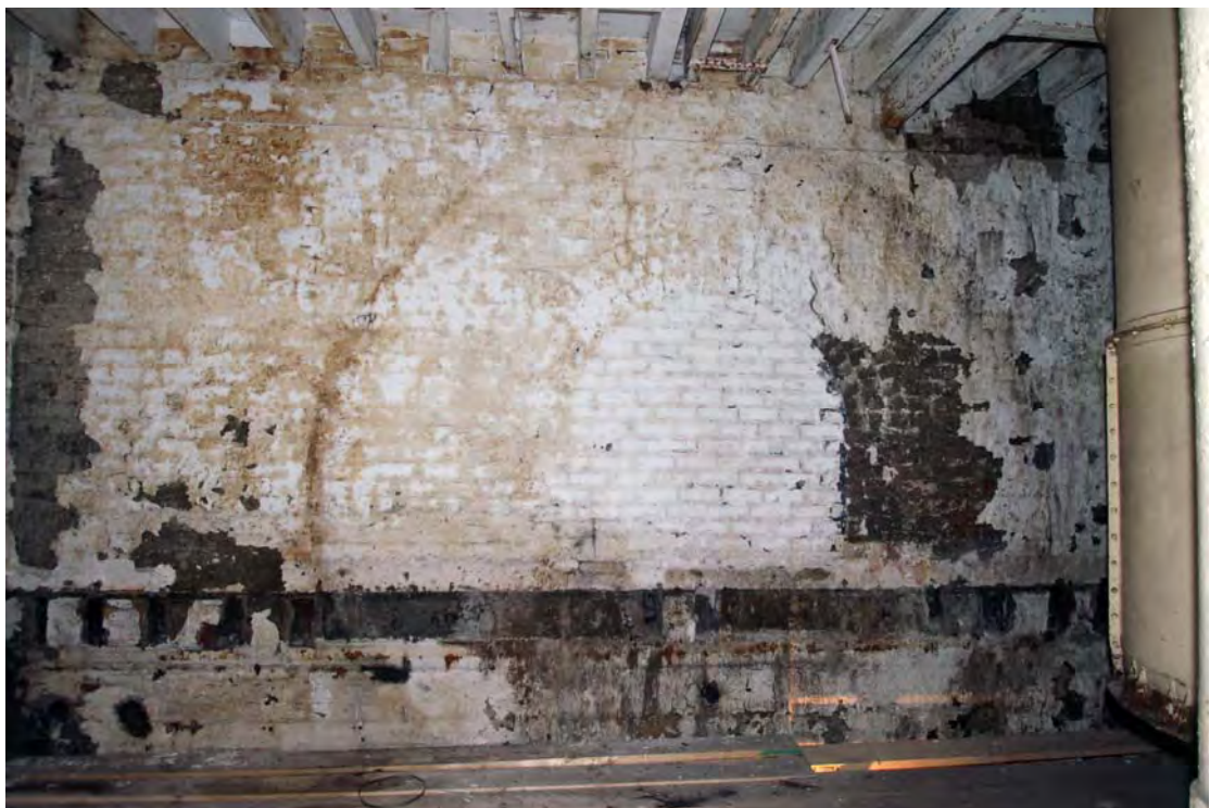
Plate 44. Former Beam Engine House (Building 11), first floor, south wall, showing circular 'ghost' of engine flywheel, probably caused by oil spatter on whitewash.
