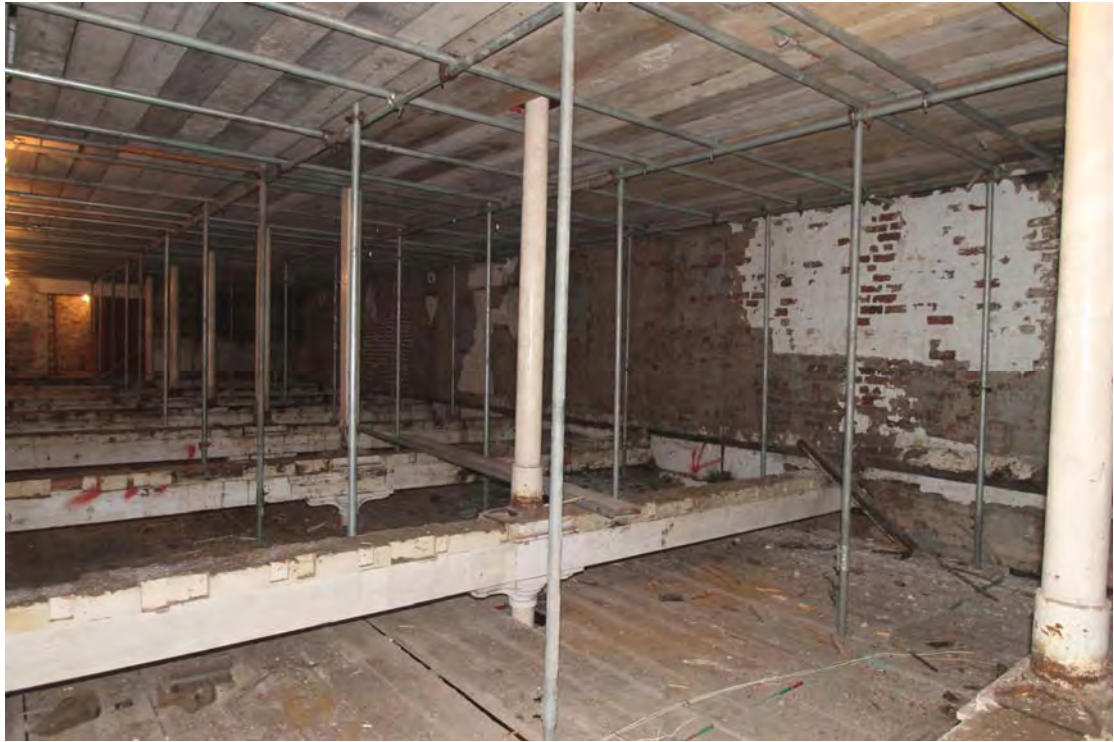
Plate 37. Original mill (Building 6), second floor, viewed from north-east, showing cast-iron column to timber beam connections.
