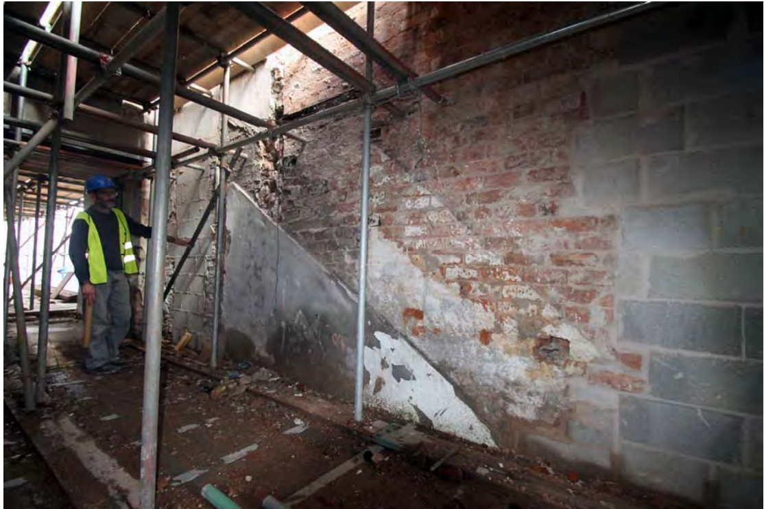
Plate 81. Mansion House, ground floor, Hallway (Room G1), showing ghost of staircase, viewed from south-west.
