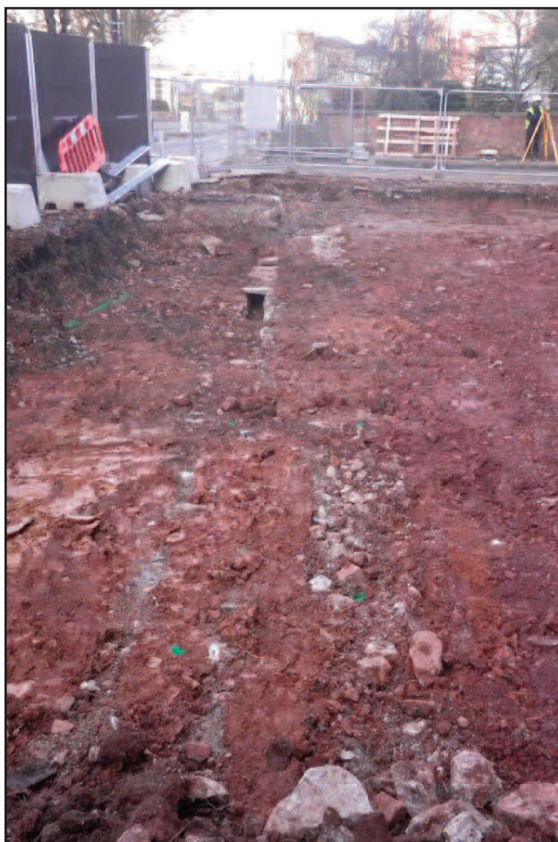
Plate 2 Looking north at the remains of 19th-century former boundary wall (106) and a stone drain (108), towards the north-west corner of the site
