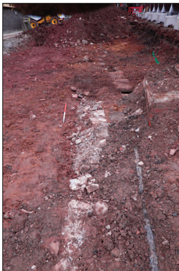
Plate 3 Looking south-west across the site at the remains of the former boundary wall (106) and stone drain (108)
