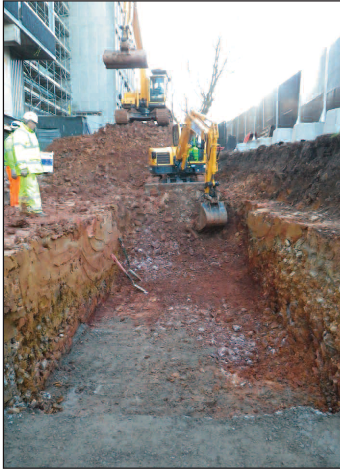
Plate 7 Excavating foundation trench for new retaining wall alongside Queens Road, looking south-west
