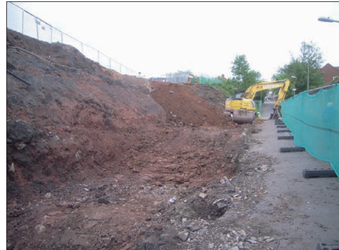
Plate 10 View north across the site during final phase of ground reduction work
