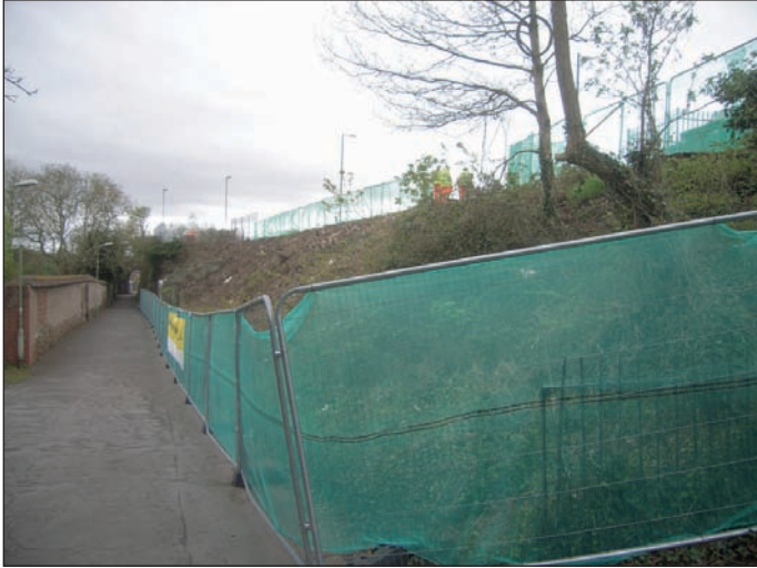
Plate 1 View south-west of the site, prior to the commencement of excavation/ground reduction work
