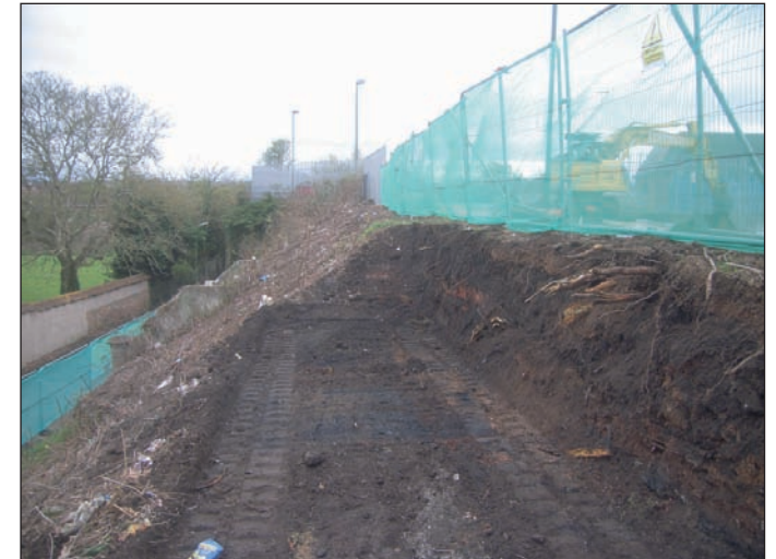
Plate 6 View south, showing east-facing 1.5m high section at the top of the embankment. Remains of a concrete water tank are visible on the lower slope
