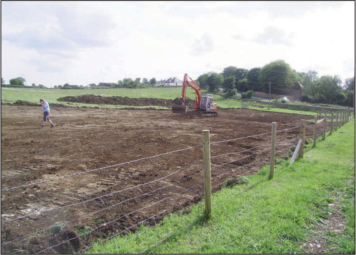
Plate 1 Stripping topsoil at the western end of the site, viewed from the north-east
