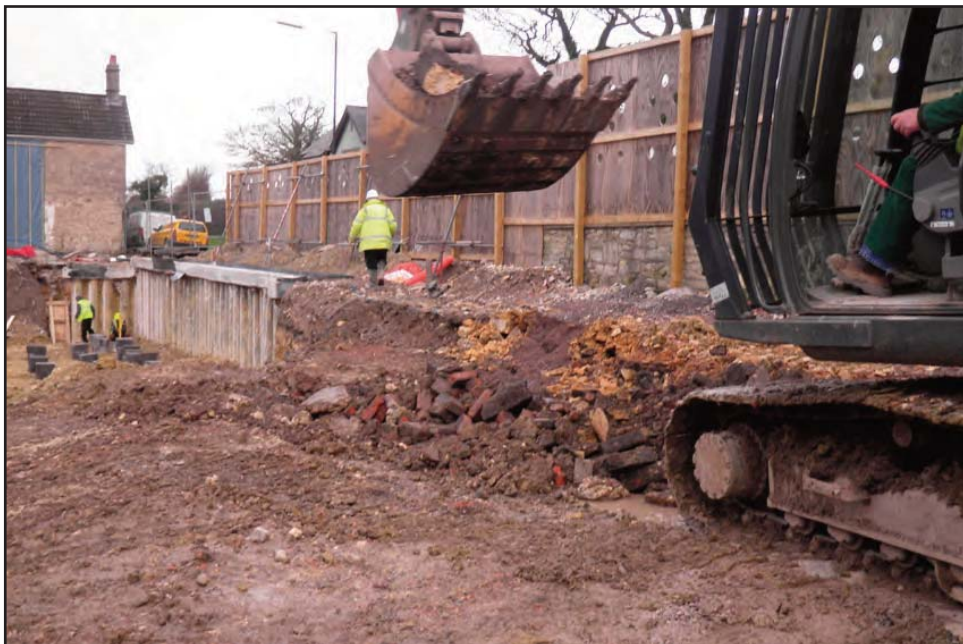
Plate 4 Ground reduction work in progress, on the site of plots 6-9, looking north-west
