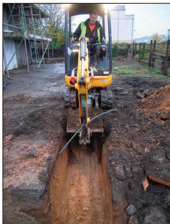
Plate 7 Excavating new-service trench to the north of the Old Gaol Stables, viewed from the east
