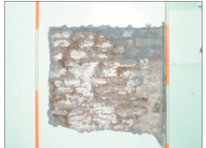
Plate 24 Stripped area in room 3, 1st floor exposing phases of stonework, looking east
