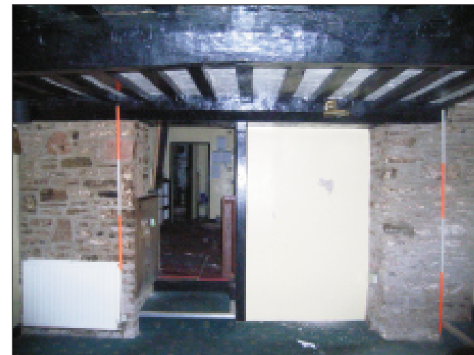
Plate 9 South internal elevation of room 1 of the historic core ground floor, looking south
