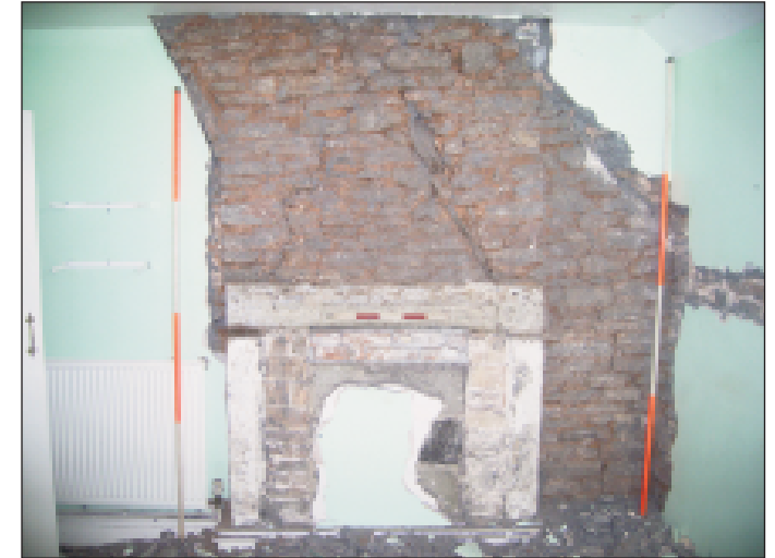
Plate 21 Stripped area in room 4, 1st floor exposing an original fireplace, looking east
