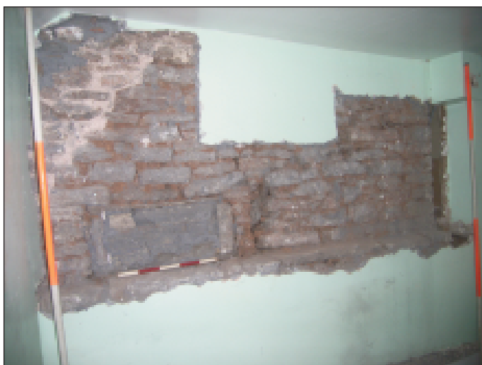
Plate 27 Stripped area in room 6, 1st floor exposing former rooflines and a blocked cupboard, looking north-east
