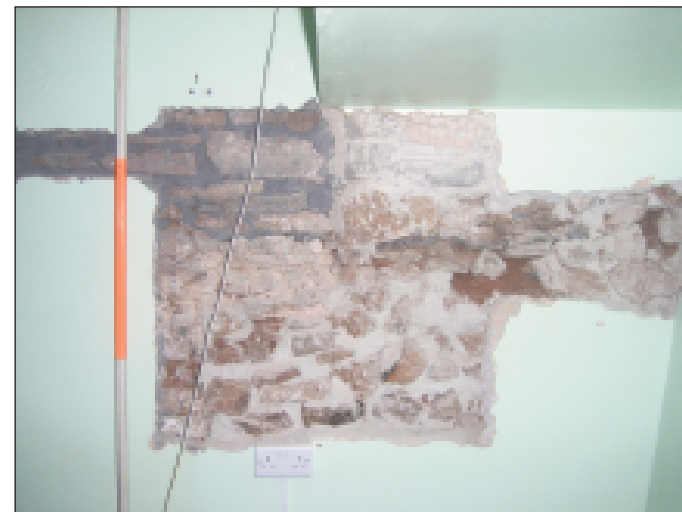
Plate 26 Stripped area in room 3, 1st floor exposing phases of stonework, looking west
