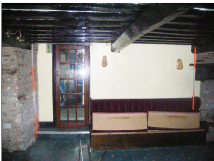
Plate 10 West internal elevation of room 1 of the historic core ground floor, looking north
