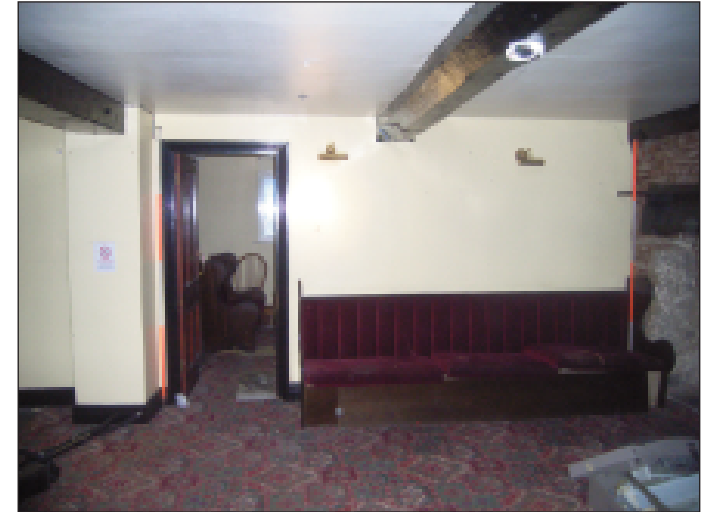
Plate 3 South internal elevation of room 2 of the historic core ground floor, looking south
