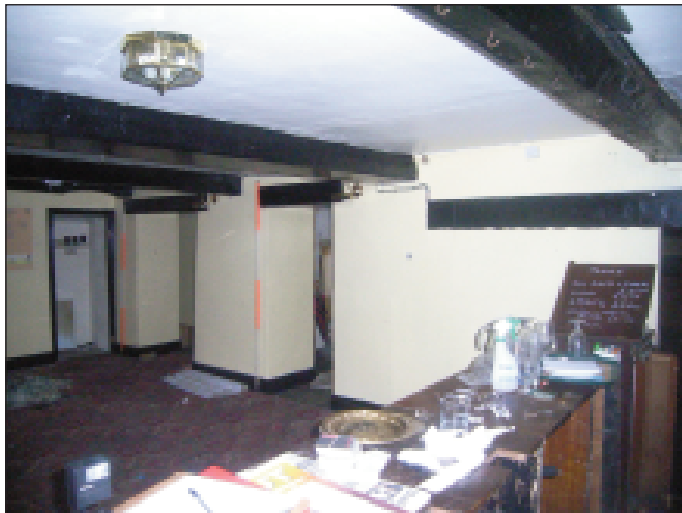
Plate 4 North internal elevation of room 2 of the historic core ground floor, looking north-west
