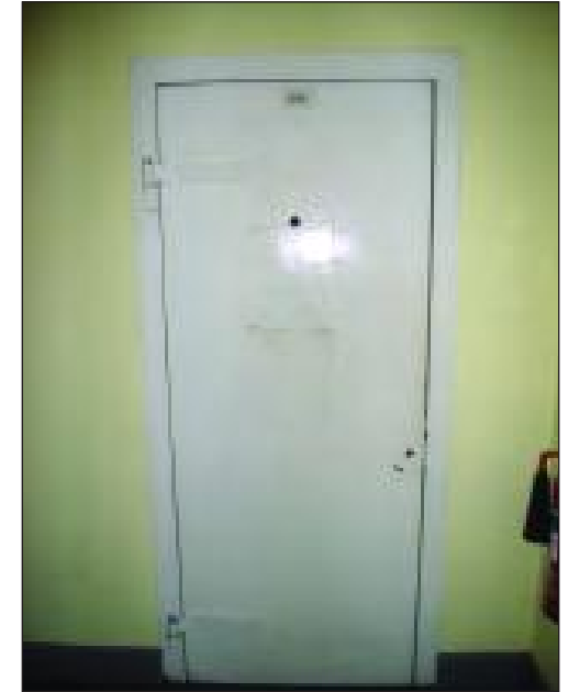
Plate 9 Door of a former cell in the middle of the main building, looking south-west
