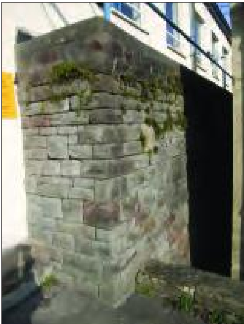
Plate 16 Retaining wall on the south-east face of the recreation block, looking north
