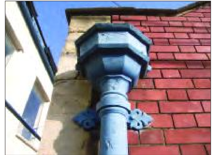
Plate 12 Ornate down-pipe and bracket on the south-west face of the 'stable' block of Redland Police Station, looking north-east
