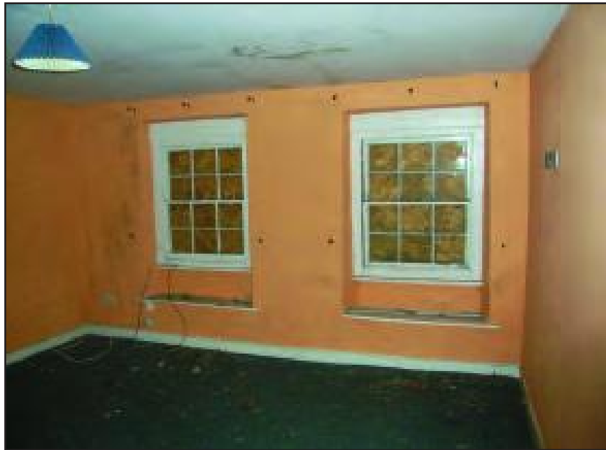
Plate 13 Second floor, living room in old Ferry House, showing window rebates, looking north-west
