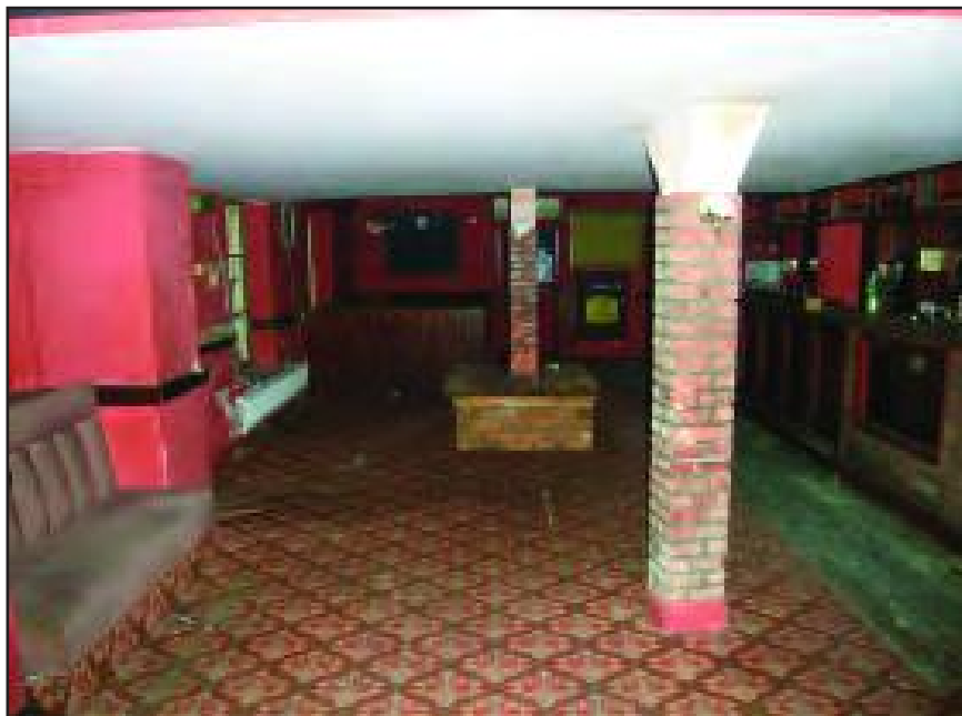
Plate 11 Ground floor open-plan bar area (historic walling removed in 1970s), looking north-east
