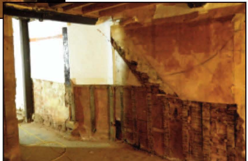
Plate 4 Exposed rubble stone wall with interlaced timberwork – looking north-east towards doorway to former lounge bar (‘Bar No. 1’)
