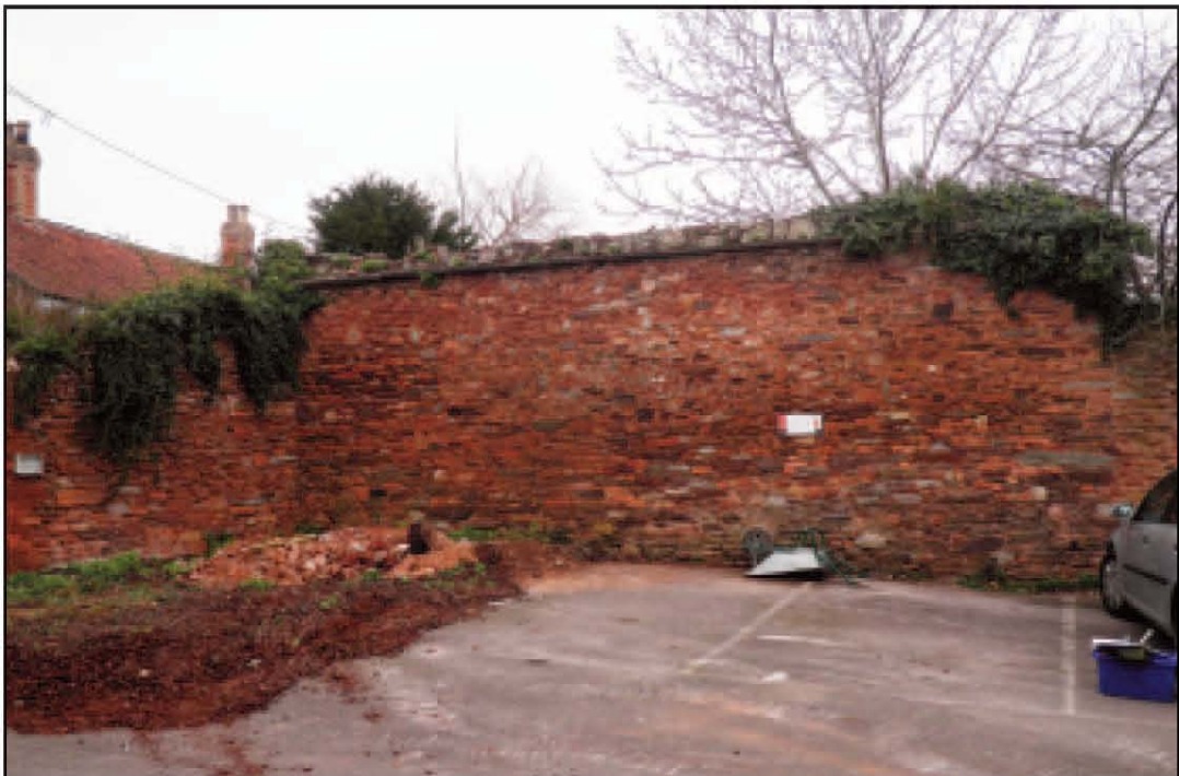
Plate 14 West-facing elevation of part of boundary wall with No. 60 Fore Street – looking north-east
