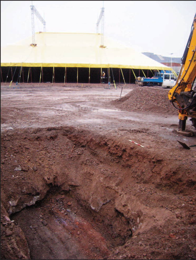
Plate 1 New drainage trench, showing modern made ground overlying 19th century made ground, viewed from the west
