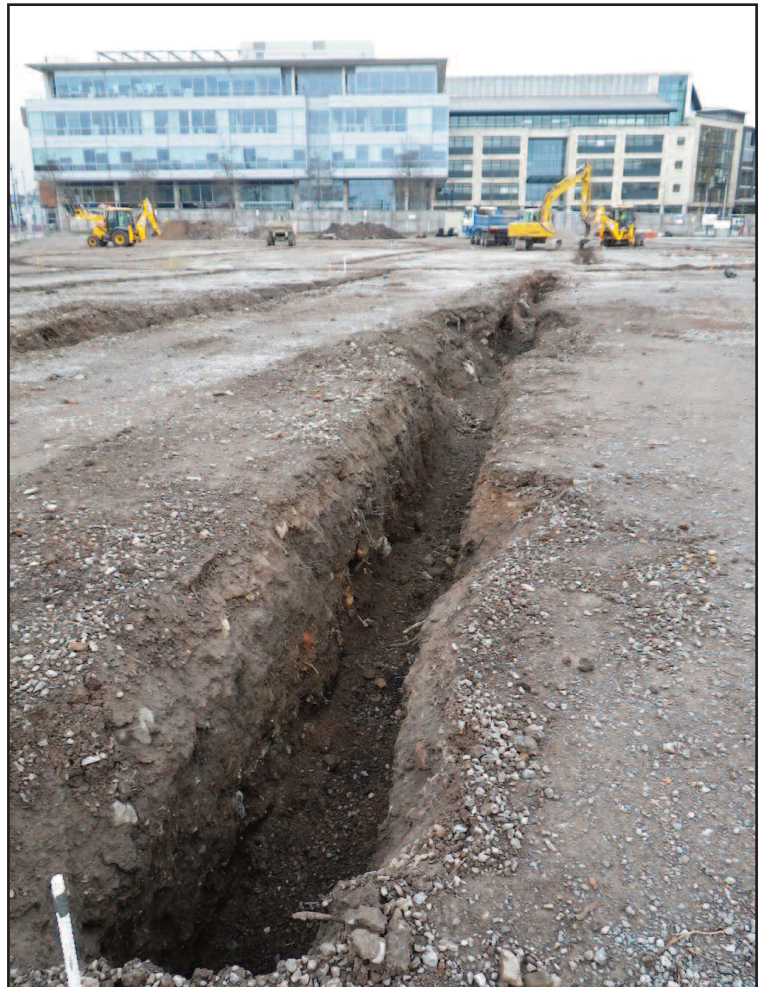
Plate 2 Foundation and drainage trenches for the new temporary events space, viewed from the east
