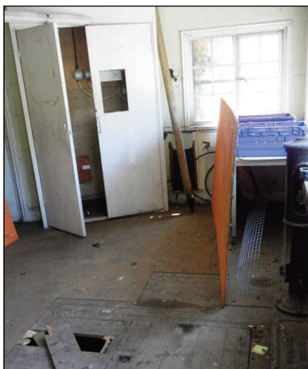
Plate 3 Interior of main room of the weighbridge house with a wooden hatch in the floor, looking south-east
