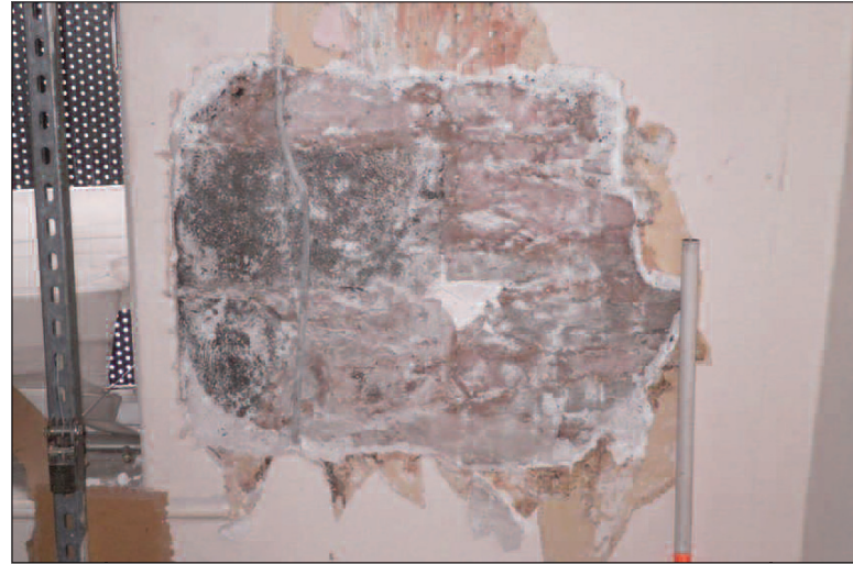
Plate 8 West sample patch of the south wall of the front east bedroom, looking south
