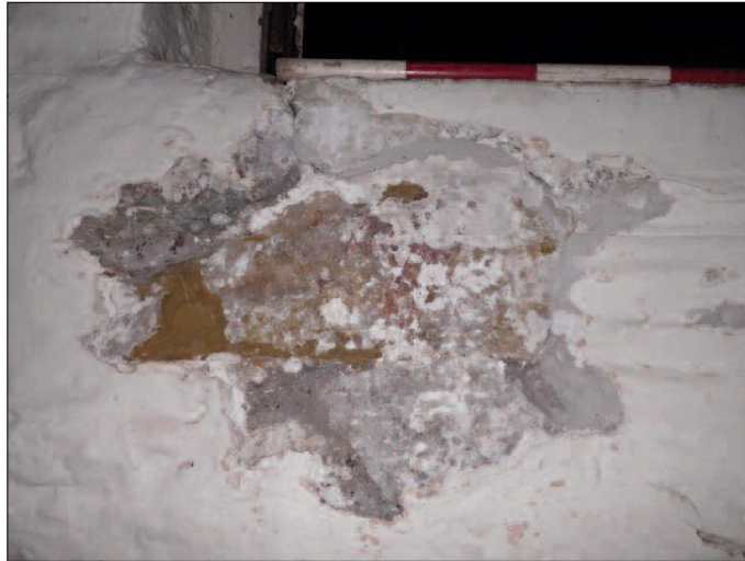
Plate 5 Exposed stonework of the south wall of the darts room, looking south
