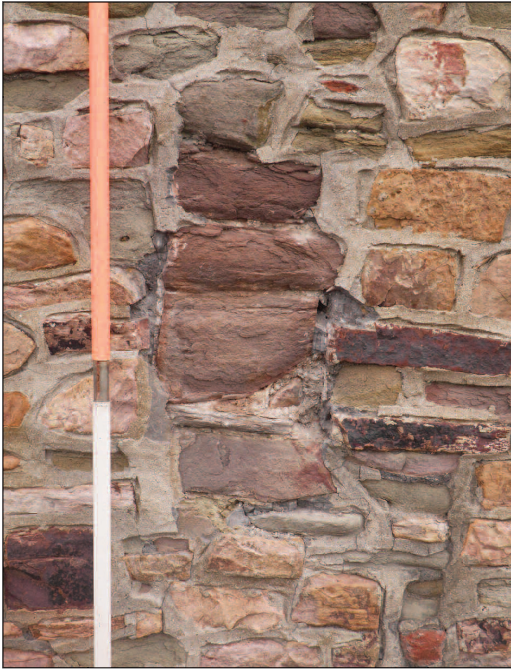
Plate 1 External face of west wall with repointing removed exposing light brown lime-based mortar, looking east
