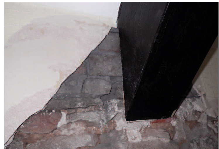
Plate 17 Rebuilt area around the inserted truss in the upstairs living area, looking north
