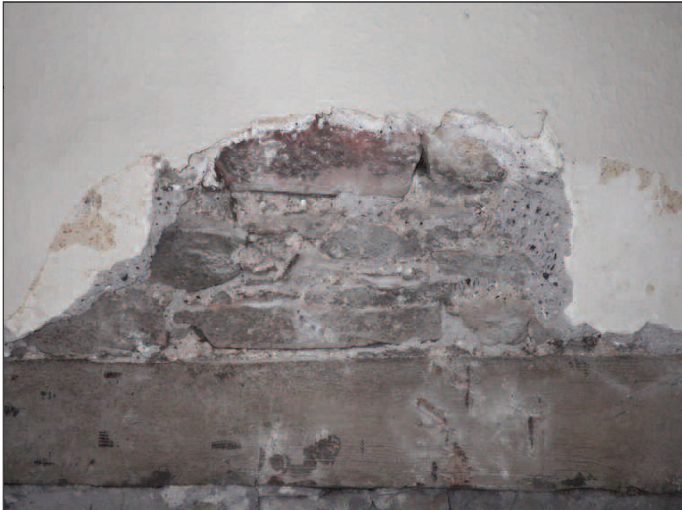
Plate 10 Area above the fireplace in the east wall of the front east bedroom, looking east
