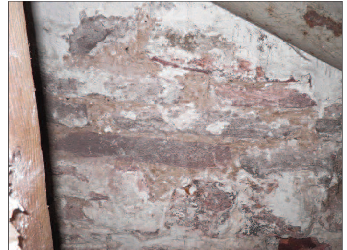
Plate 6 Exposed stonework of the west wall of the darts room section of stud wall removed, looking west
