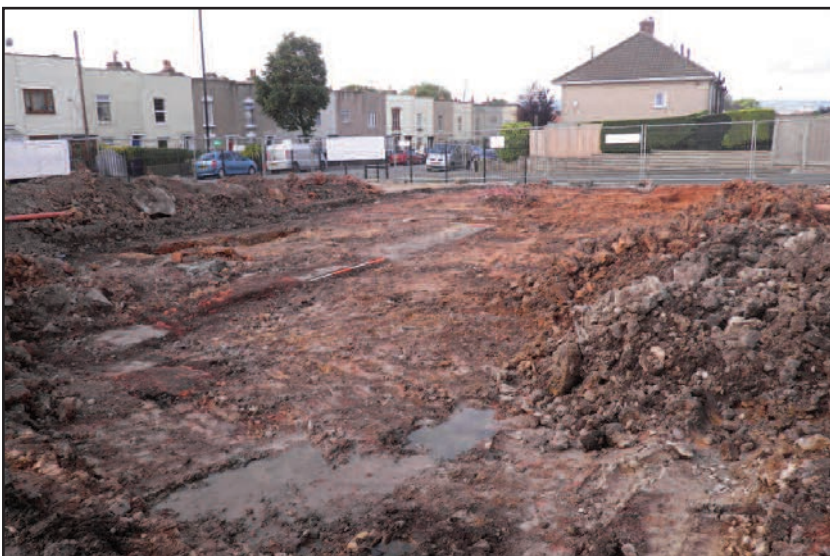
Plate 22 General view of the site from the north-east corner, foundations of the porch added in 1911 visible, looking south-west
