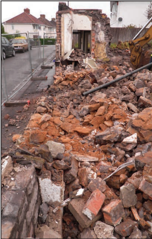
Plate 3 Demolished west end elevation with sections of original clay-bonded stonework visible, looking north
