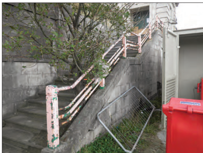
Plate 28 Staircase to the flat roof of the north side wing with original railings, looking south-east
