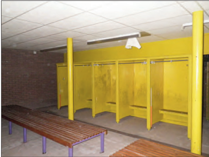
Plate 19 Womens changing room in north side wing with original cubicles, looking south-west
