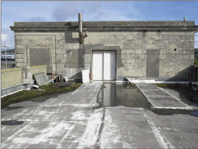
Plate 13 South-facing elevation of the central pavilion building first floor viewed from the south side wing roof, looking north
