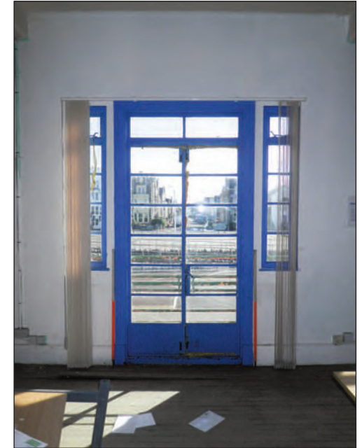
Plate 9 Glazed doors leading to the first floor balcony of the central pavilion building, looking east
