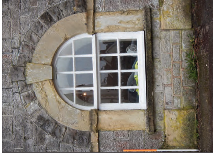
Plate 4 Ground floor window of the east elevation of the principal building, looking west
