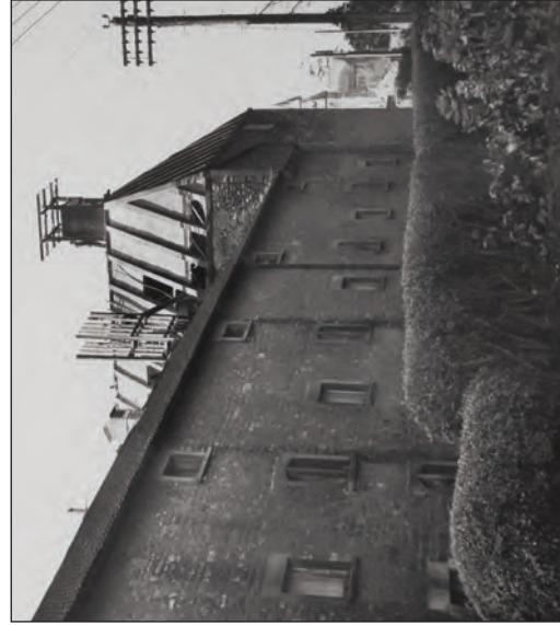
Plate 41 1960s photograph of the west end of the principal building and the new saladin box kilns being constructed
