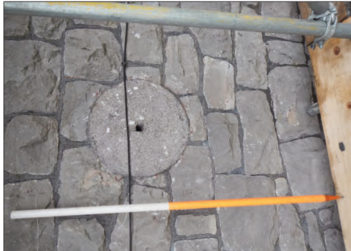
Plate 34 Cement 'scar' of a wall plate on the east elevation of the malt house, looking west
