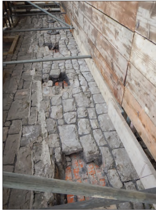
Plate 35 Blocked holes in the north elevation of the malt house where iron beams sat previously, looking south-west
