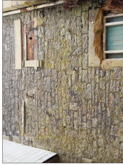
Plate 18 Cut-off iron beams at different heights in the south-facing elevation of the principal building, to the east of the bridge, looking north
