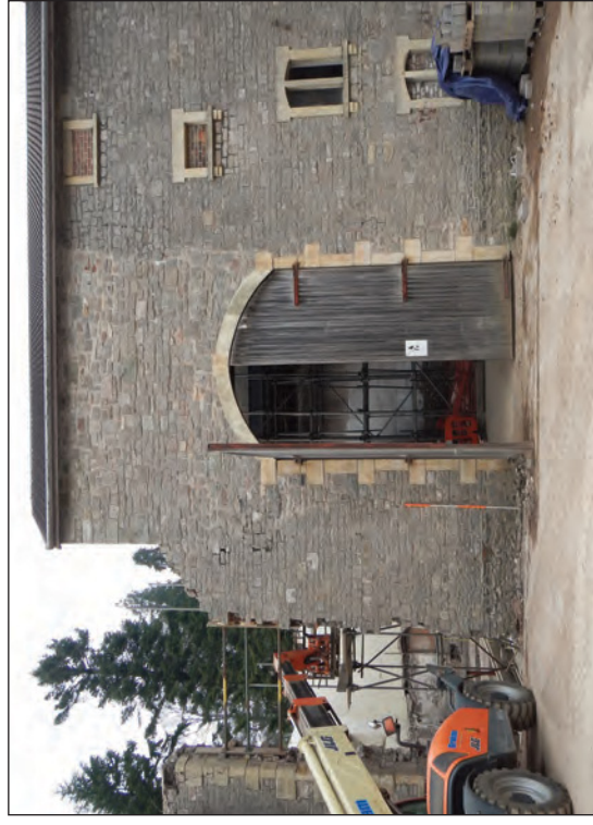
Plate 15 Modern opening and rebuild at the west end of the south elevation of the principal building, looking north
