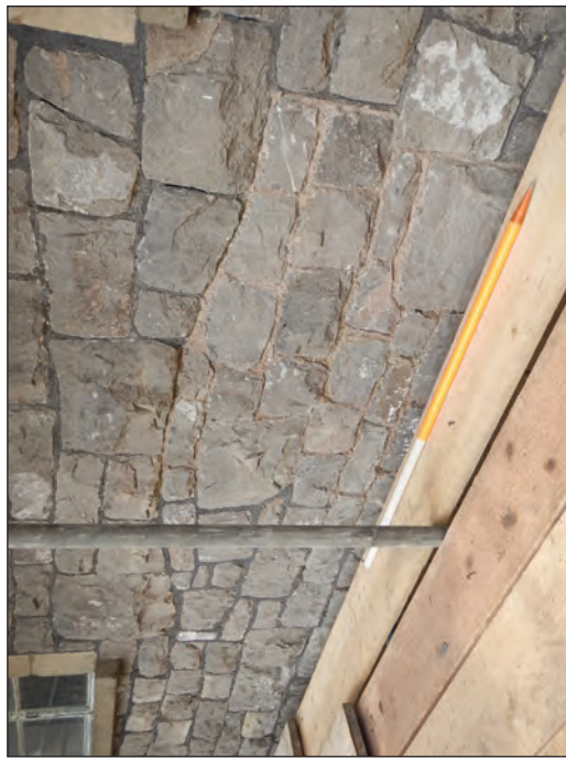
Plate 33 Blocked window opening in the east elevation of the malt house, looking south-west
