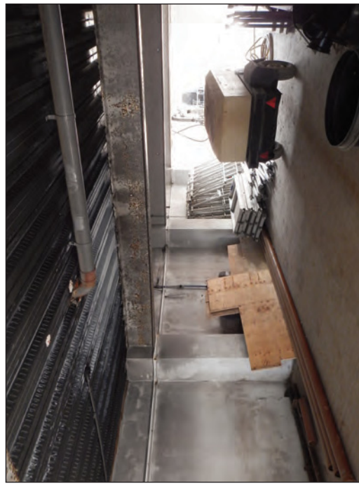
Plate 24 Underside of the modern mezzanine floor in the principal building, looking south-west
