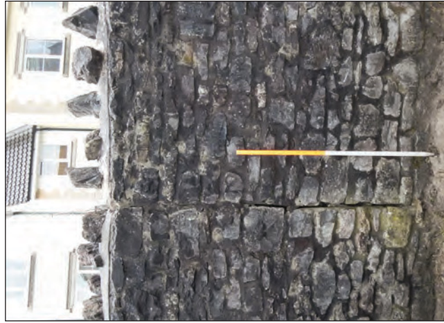
Plate 37 Break in boundary wall, looking south-east
