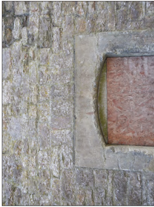
Plate 9 North elevation of the principal building, altered archway at the west end, looking south
