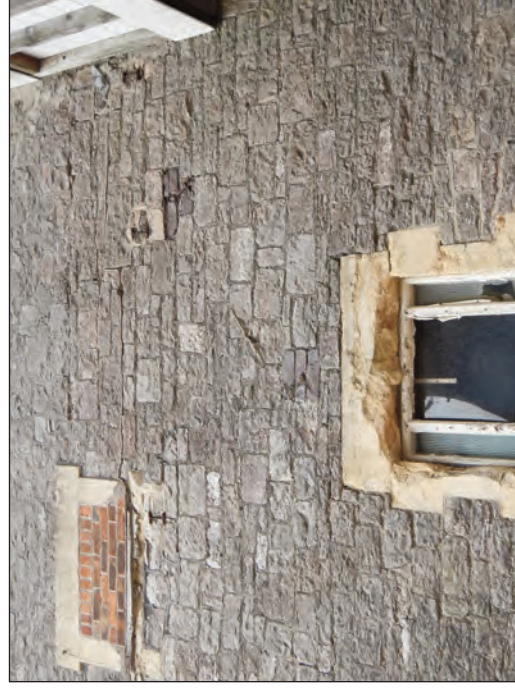
Plate 17 Cut-off iron beams at different heights in the south-facing elevation of the principal building, to the west of the bridge, looking north
